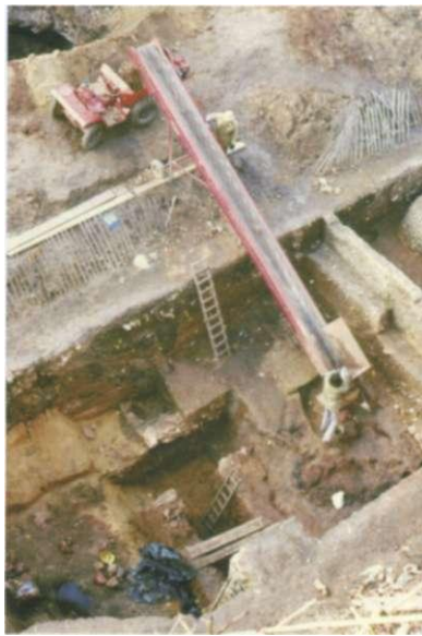
Excavations in progress on the site of the Cups Hotel in 1973 (x on the plan).
