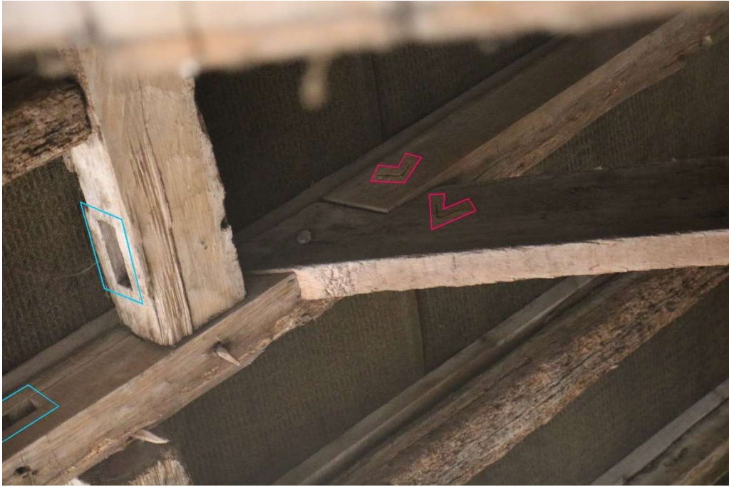
Photograph 7 Detail of half-dovetail joint and carpenter's marks (in pink) in the collars and rafters of the coach house. Area's evidencing reuse highlighted in blue. Photograph taken facing south-west.
