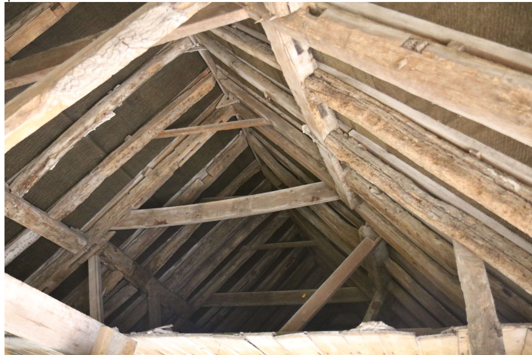
EEX60095_PhotoGraph_018 Detail of roof construction of coach house. Photograph taken facing east.
