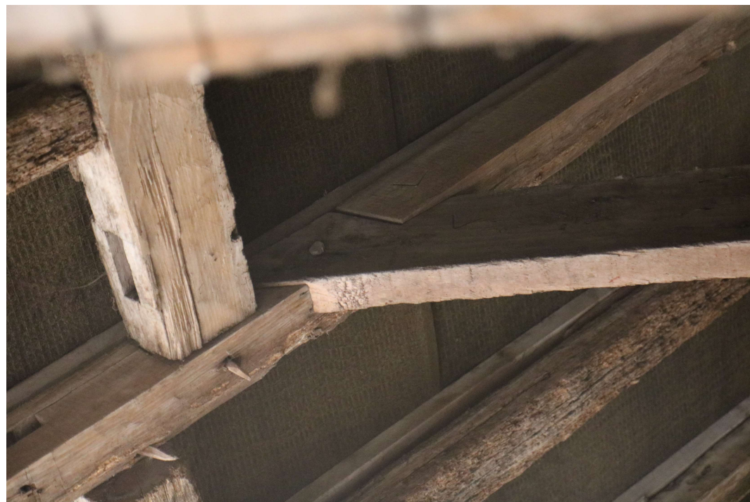
EEX60095_PhotoGraph_020 Detail of half-dovetail joint and carpenter's marks in the collars and rafters of the coach house. Photograph taken facing south-west.
