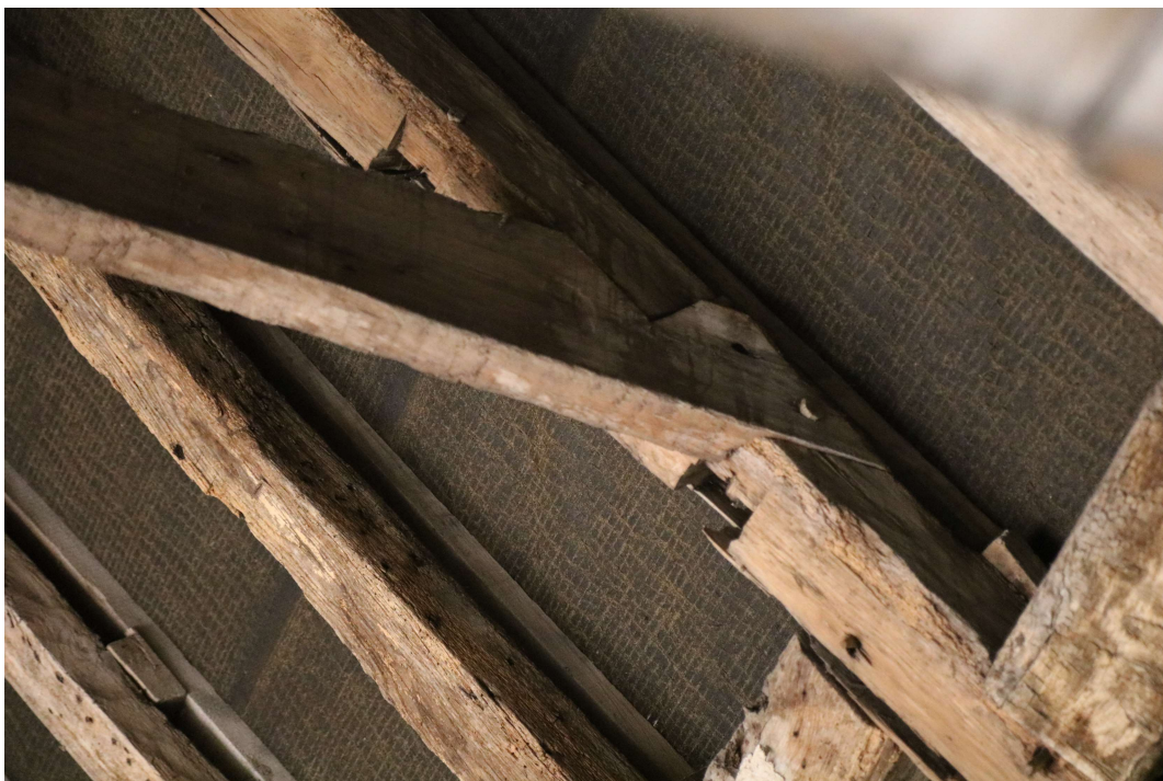
EEX60095_PhotoGraph_019 Detail of half-dovetail joint in the collars and rafters of the coach house. Photograph taken facing north-west.
