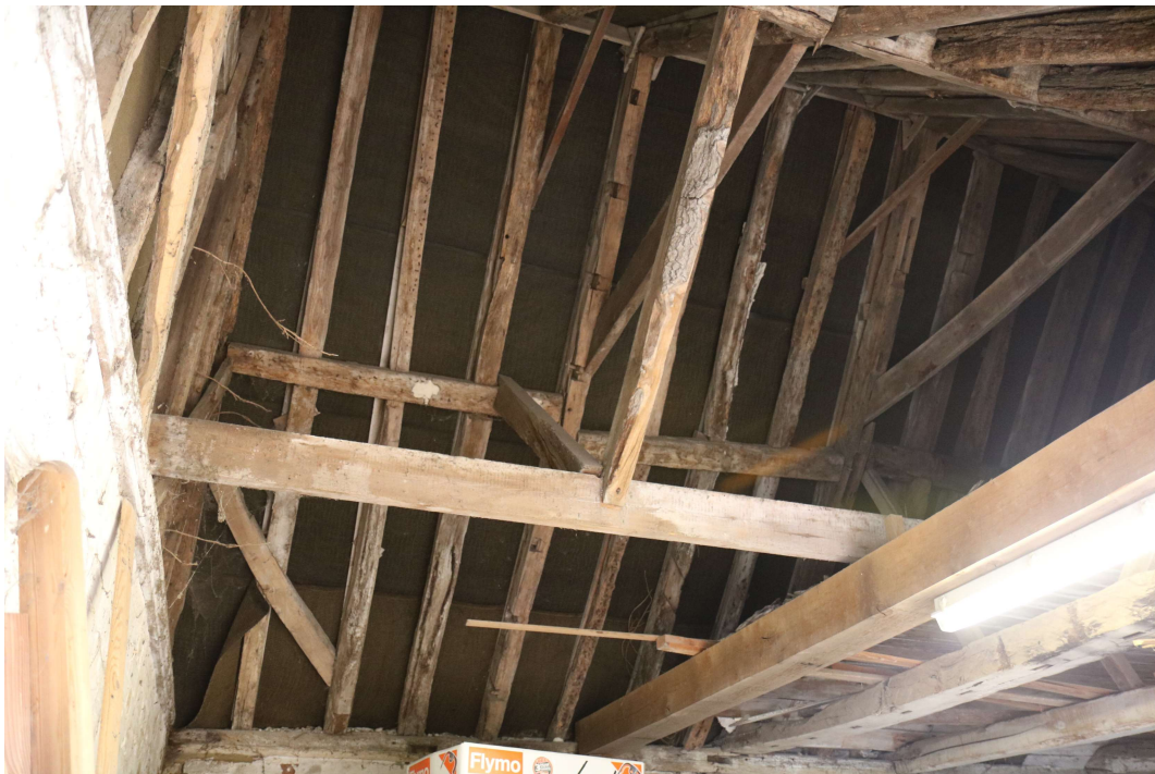
EEX60095_PhotoGraph_015 Detail of roof construction of coach house. Photograph taken facing north-east.
