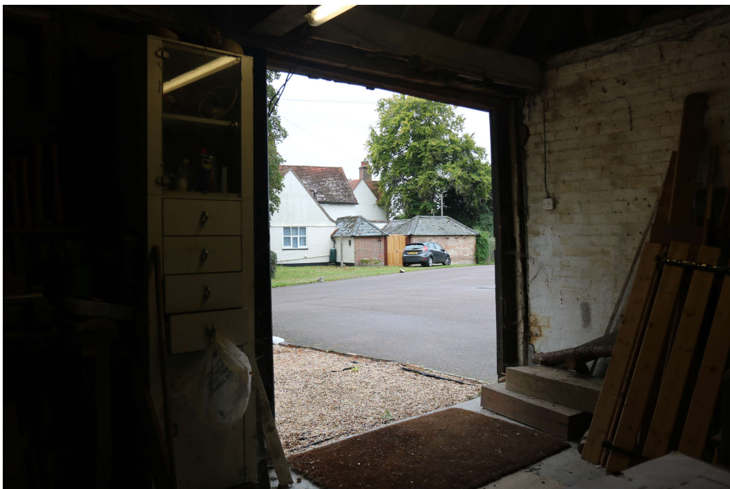
EEX60095_PhotoGraph_027 Detail of doorway in south-western wall of coach house. Photograph taken facing south-west.
