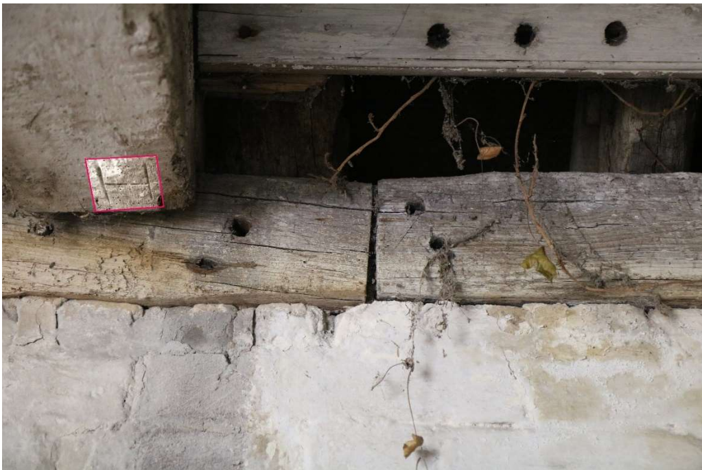
Photograph 8 Detail of north-eastern wall-plate scarf-joint and tie-beam carpenter's mark (in pink). Photograph taken facing north north-east.
