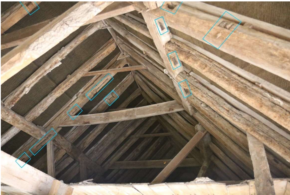
Photograph 6 Detail of roof construction of coach house. Area's evidencing reuse highlighted in blue. Photograph taken facing east.
