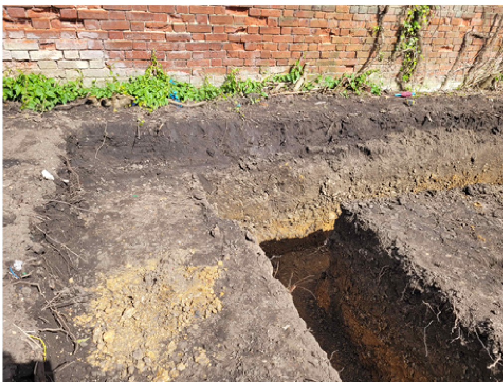
Photograph 3 Foundation trenches, looking east-north-east, showing depth of topsoil stripped prior to work starting.
