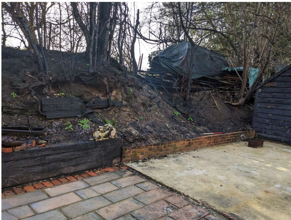
Photograph 1 Damage to dyke prior to reconstruction work, view south-east.
