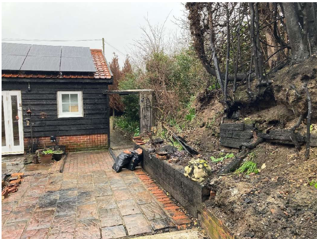
Photograph 3 Damage to dyke prior to reconstruction work, view north north-east (photograph courtesy of Dr Jess Tipper).
