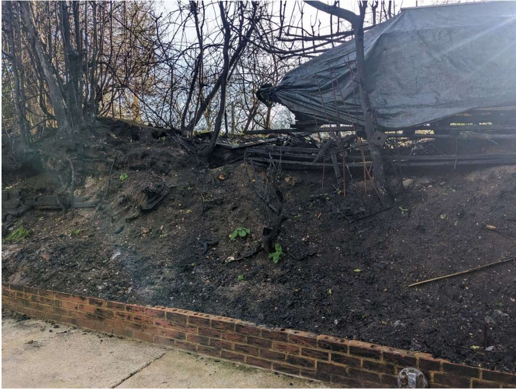
Photograph 2 Damage to dyke prior to reconstruction work, view north-east.
