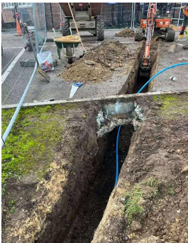
Photograph 9 Working shot of service trench, view west. The concrete surface in the background is the beginning of L5.
