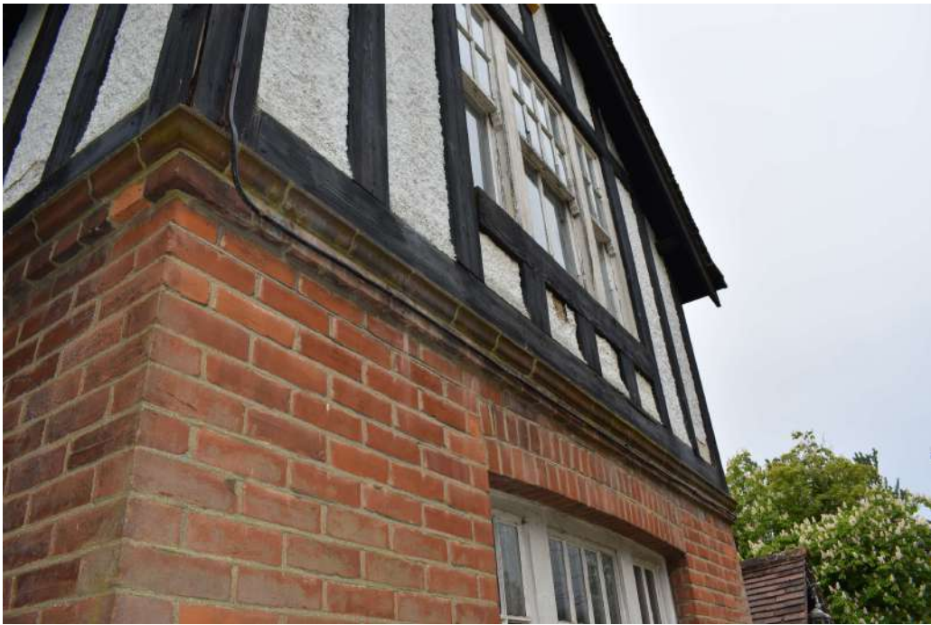
Photograph 3 Detail of moulded oversailing brickwork of northern elevation. Photograph taken facing south-west.
