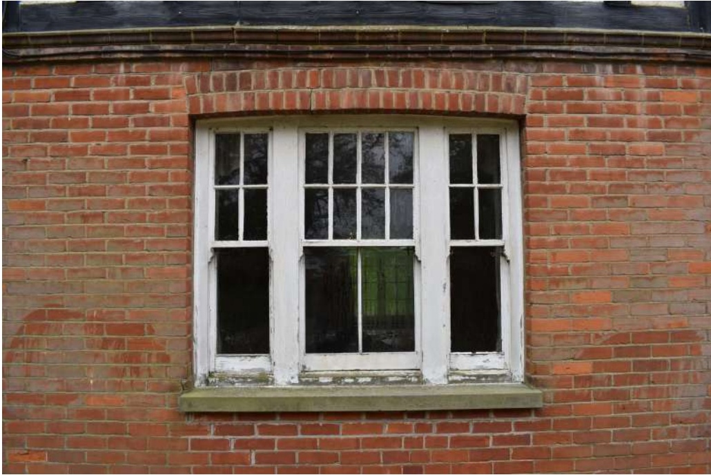
Photograph 6 Detail of ground floor window of northern elevation. Photograph taken facing south south-west.
