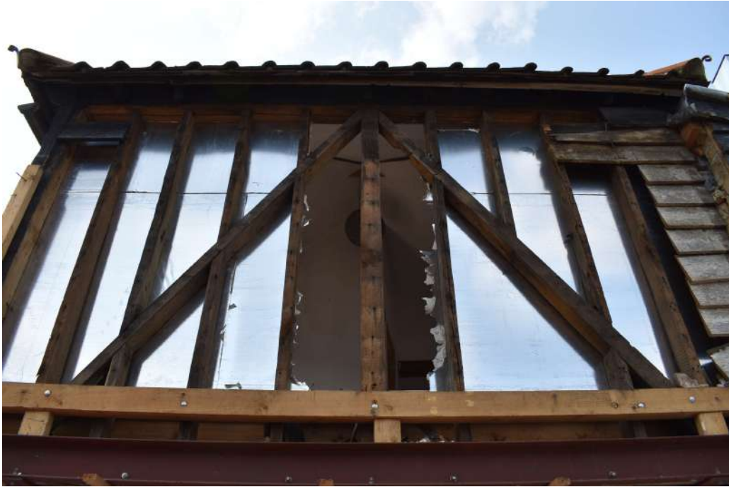
Photograph 37 Detail of timber-framing in first floor of range 2. Photograph taken facing north-west.
