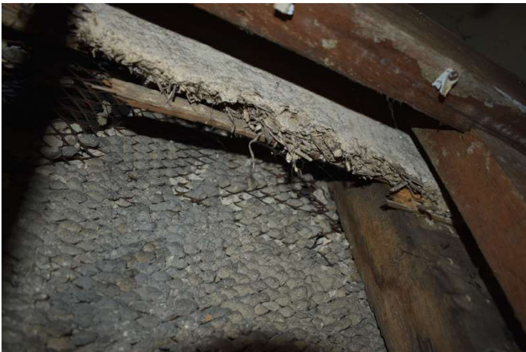
Photograph 33 Detail of plaster in north-east wall of range 10. Photograph taken facing east.
