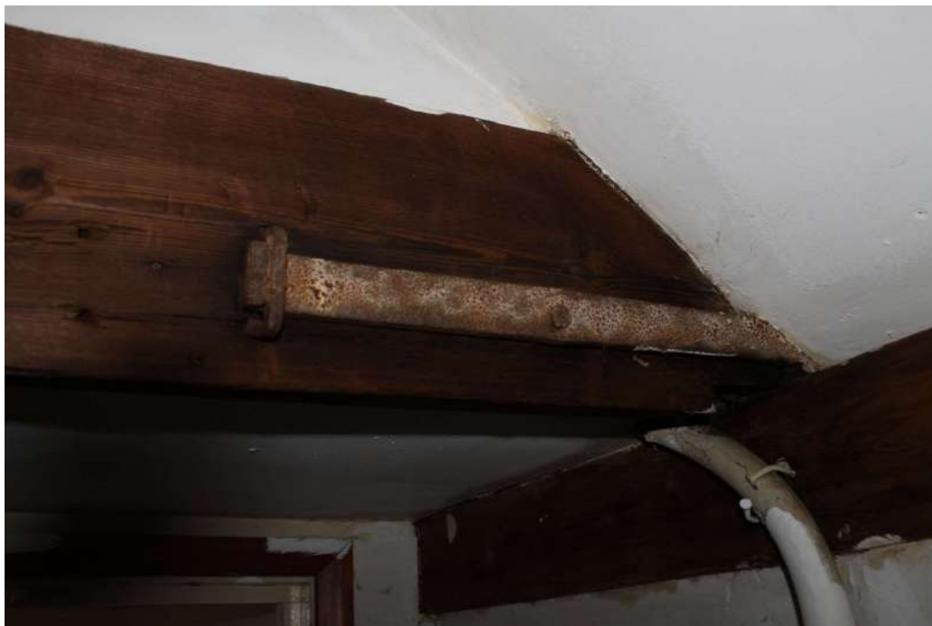
Photograph 13 Detail of iron strap joint on tie-beam in range 2. Photograph taken facing north.
