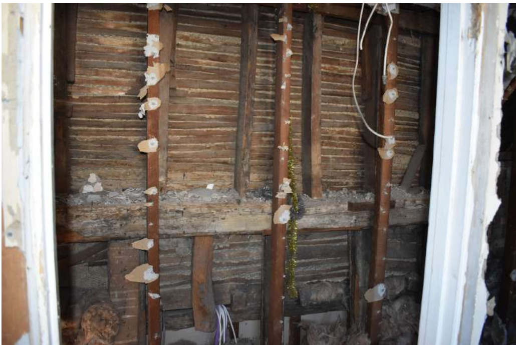
Photograph 31 Detail of timber-framing, including laths, in south-eastern wall of range 10. Photograph taken facing south-east.
