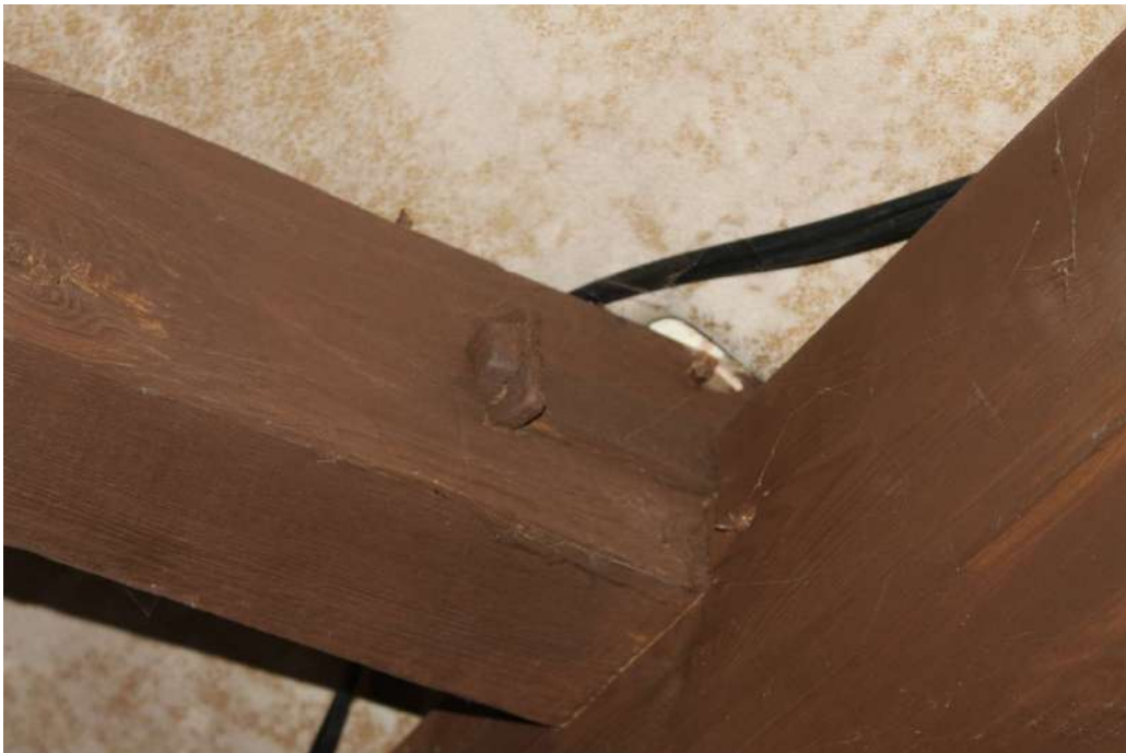
Photograph 15 Detail of iron strap on southern tie-beam in range 3. Photograph taken facing north-east.
