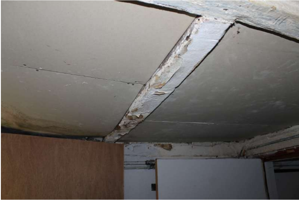
Photograph 28 Detail of floor joists in ceiling of range 4. Photograph taken facing west.
