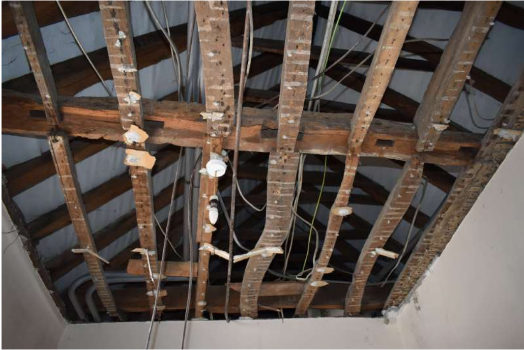
Photograph 34 Detail of ceiling joists and tie-beam in range 6. Photograph taken facing north-west.
