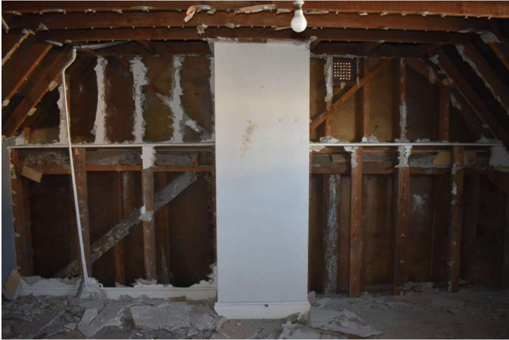
Photograph 32 Detail of timber-frame in south-western wall of range 10. Photograph taken facing south-west.
