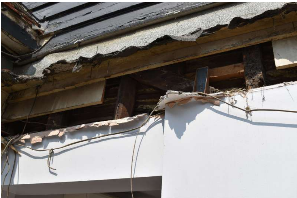
Photograph 25 Detail of timber-framing in south-west wall of range 6. Photograph taken facing north.
