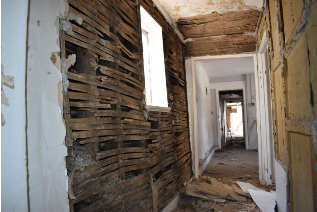
Photograph 35 Detail of laths in north-eastern wall of range 6. Photograph taken facing south-east.
