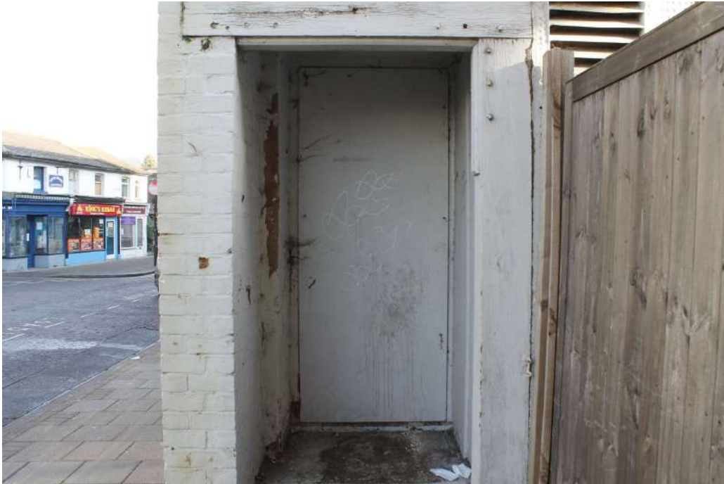
Photograph 8 Detail of doorway on south-west elevation of range 10. Photograph taken facing north-east.
