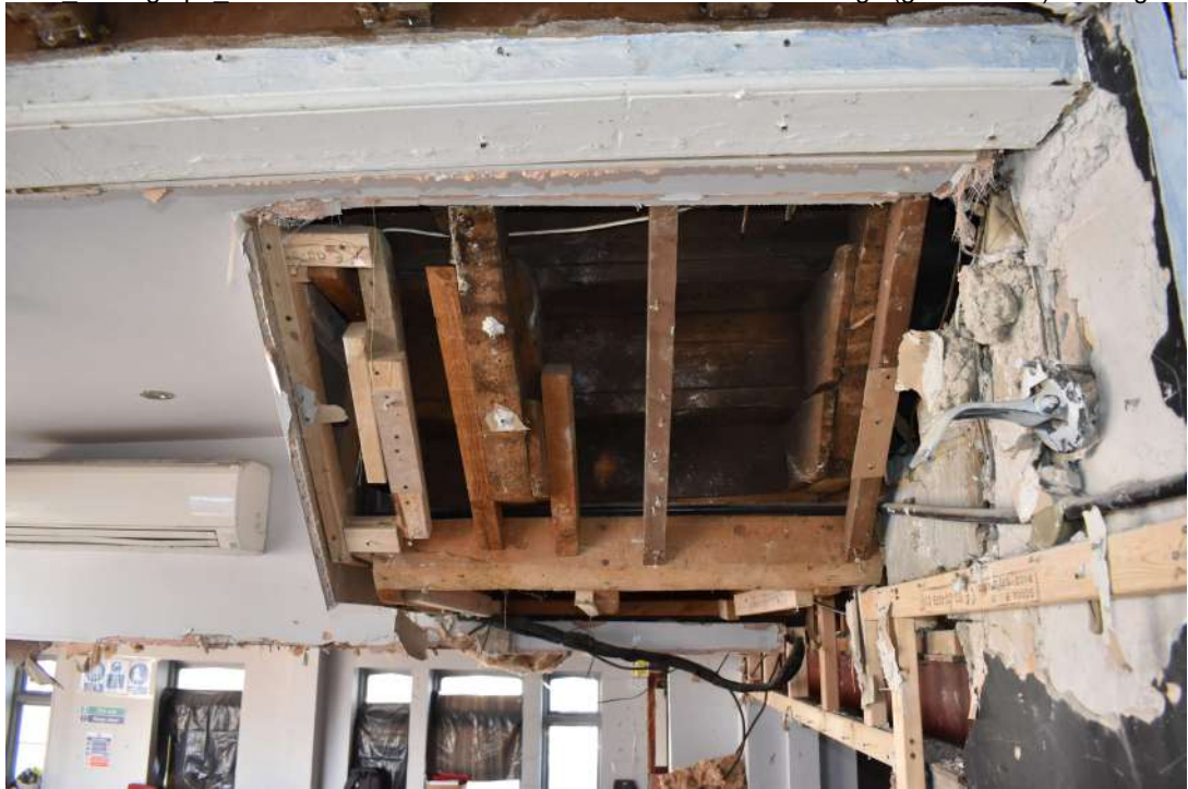
CF98 Photograph 149Detail of under-stair construction in north-west range (ground floor). Photogra...
