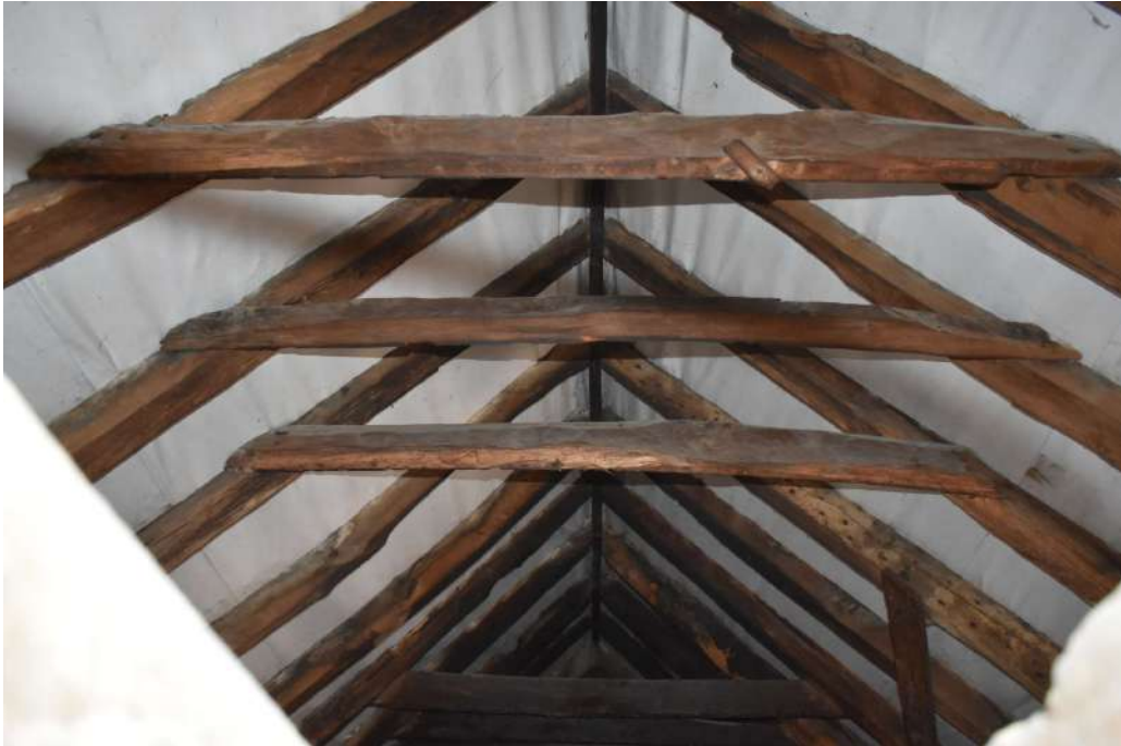
Photograph 16 Detail of roof construction of range 6. Smoke blackened timbers visible towards the rear. Photograph taken facing south-east.
