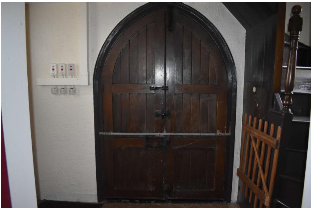
Photograph 17 Detail of door in north wall of entrance hall. Photograph taken facing north.
