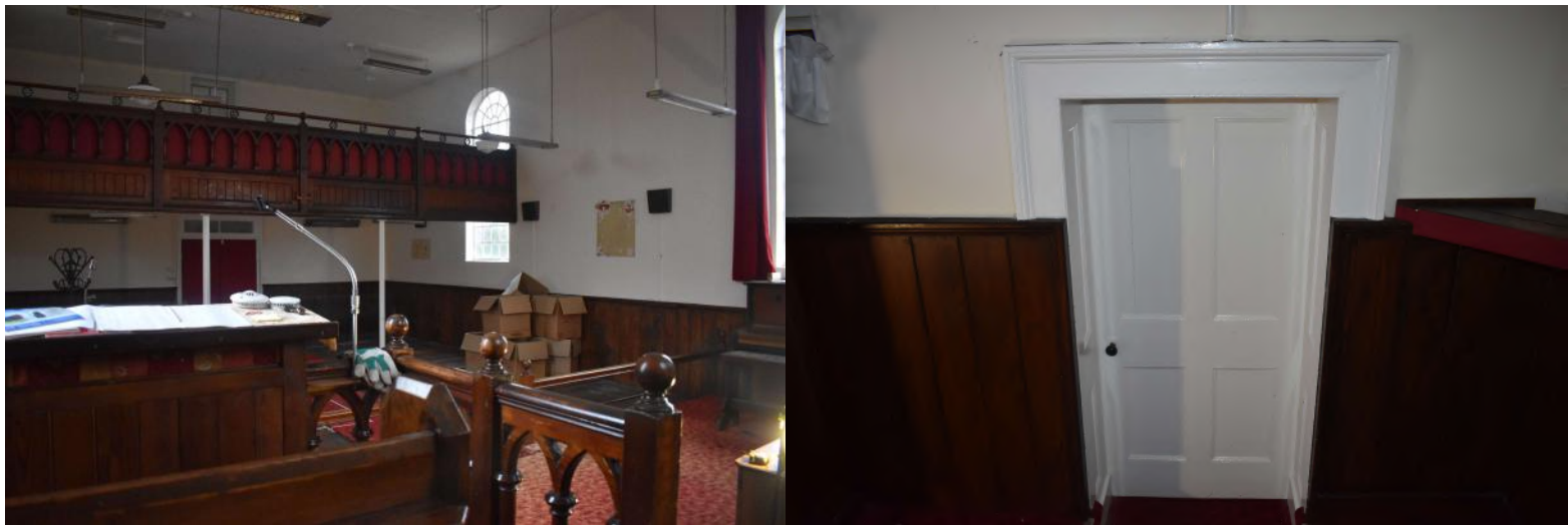
ECC4764_PhotoGraph_041Detail of internal door between main hall a... ECC4764_PhotoGraph_042Internal detail of window on south wall of m...
