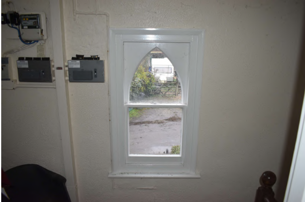
Photograph 18 Internal detail of window on north wall of landing. Photograph facing north.
