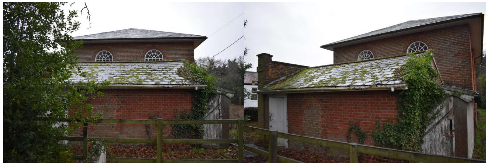
ECC4764_PhotoGraph_021Detail of window on south elevation. Photo... ECC4764_PhotoGraph_022Detail of window on south elevation. Photo...
