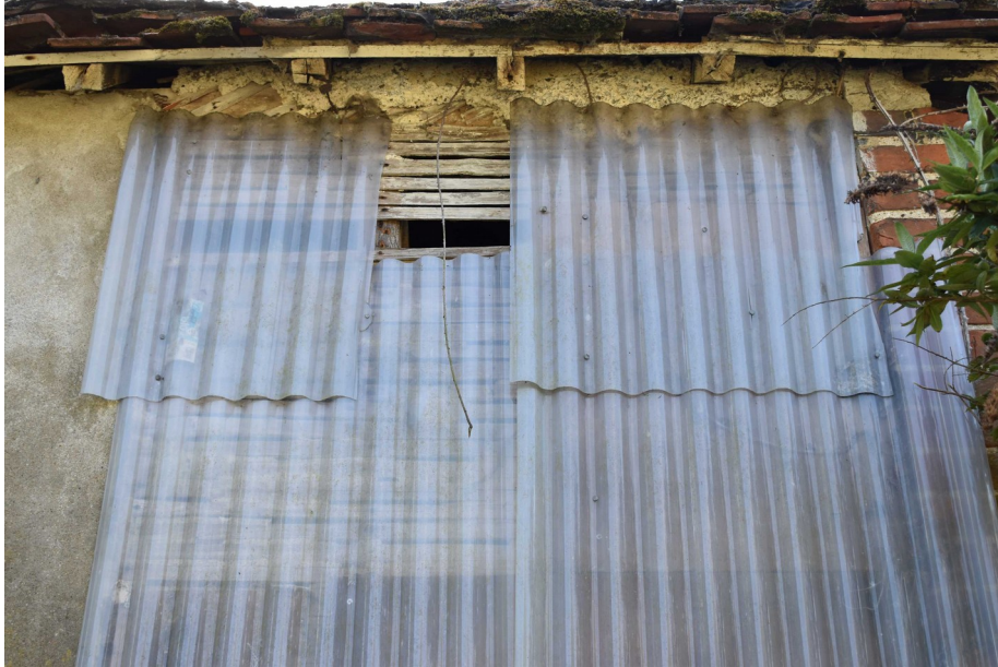
Photograph 15 Exposed laths on north-west elevation of coach house. Photograph taken facing south-east.
