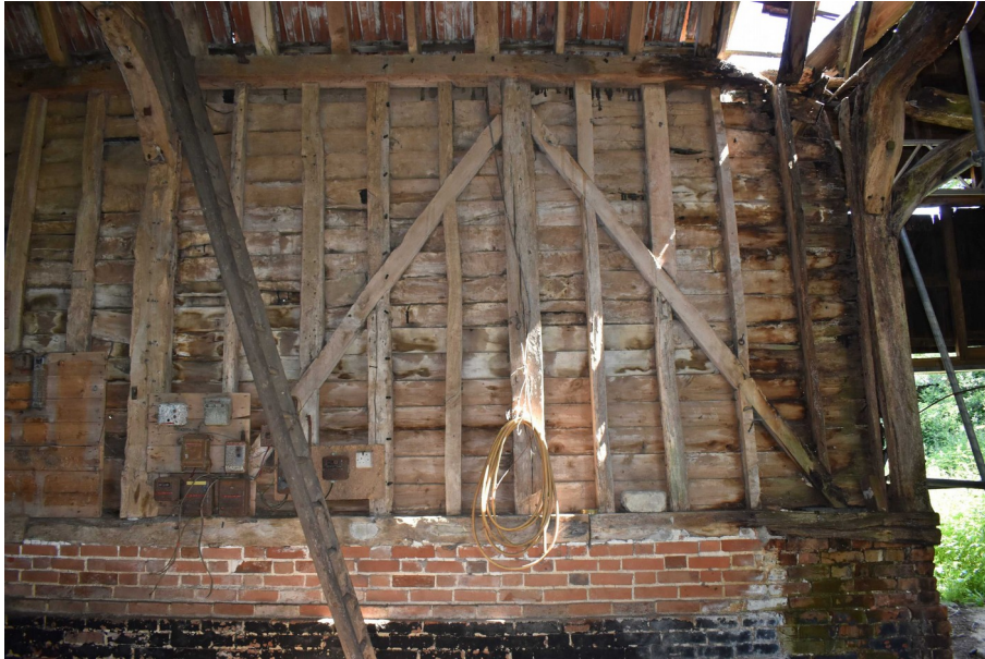
Photograph 7 North-east elevation of bay 2 showing water damage. Photograph taken facing south-west.
