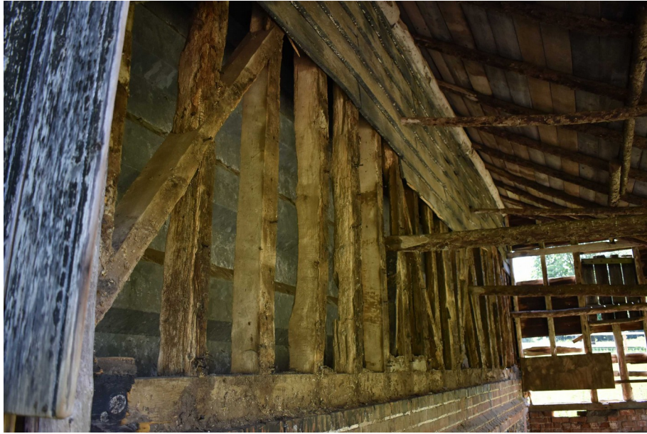
Photograph 2 Exposed timbers on south-west elevation of threshing barn. Photograph taken facing east.
