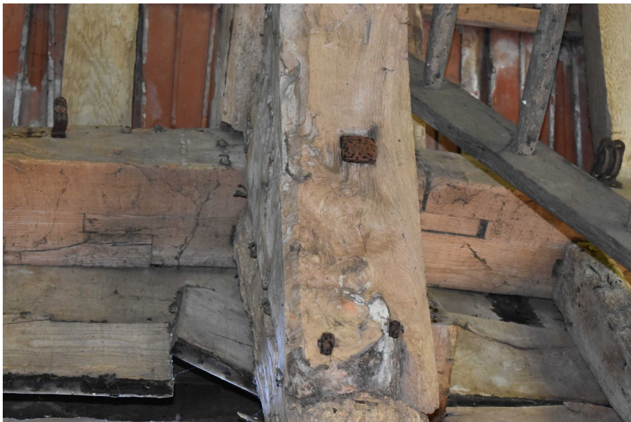
Photograph 6 Scarf joint on wall plate of north-east elevation between bays 1 and 2. Photograph taken facing north-east.
