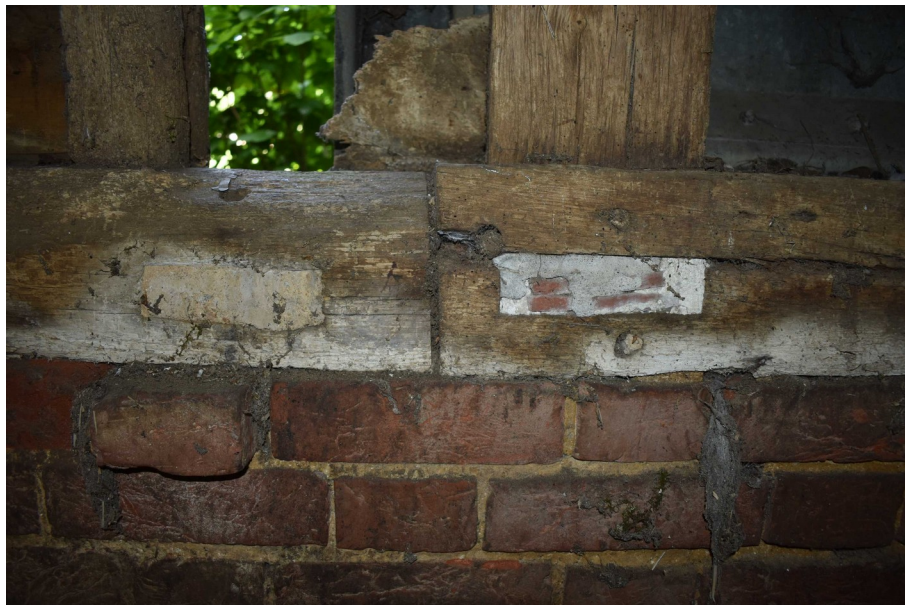
Photograph 9 Detail of scarf joint and filled mortices on sill-beam of north-east elevation in bay 4. Photograph taken facing north-east.
