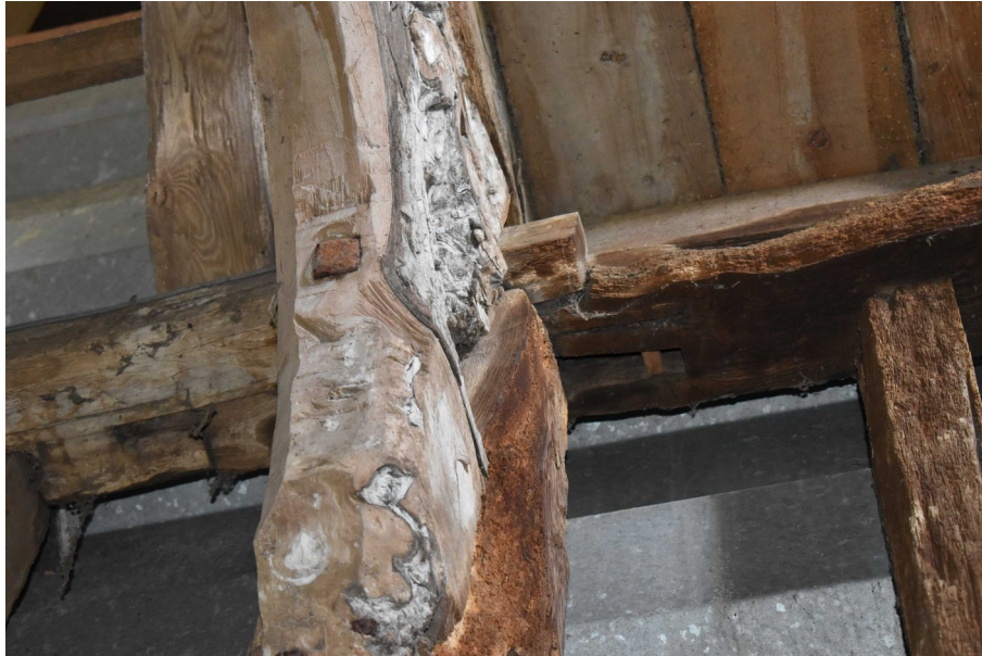
Photograph 10 Scarf joint and re-used timber in wall-plate in north-east elevation between bays 4 and 5. Photograph taken facing north-west.
