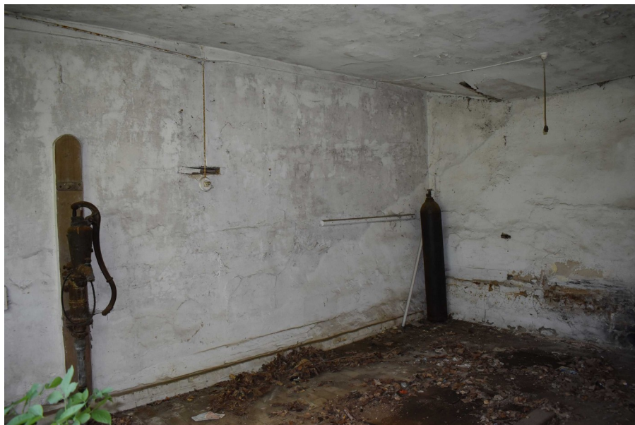
Photograph 21 Interior of garage showing water pump and gas lamp mount. Photograph taken facing north-east.
