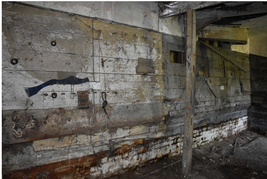
Photograph 19 Wooden cladding on walls in main room of coach house. Photograph taken facing south-east.
