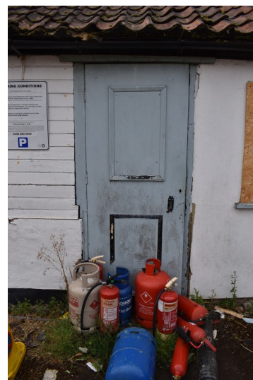
Photograph 3 Inserted modern door on north-west elevation of outbuilding. Photograph taken facing south-east.
