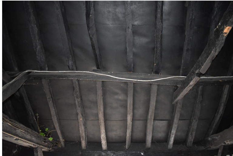
Photograph 12 Detail of hand-sawn rafters on south-eastern pitch of roof above bay 2. Photograph taken facing south-east.
