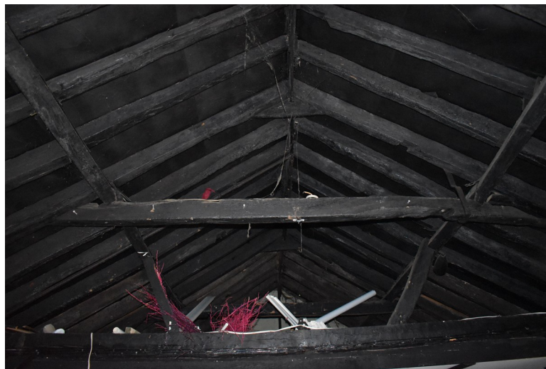
Photograph 10 Detail of roof of outbuilding above bay 4, showing struts, collars and clasped-purlins. Photograph taken facing north-east.
