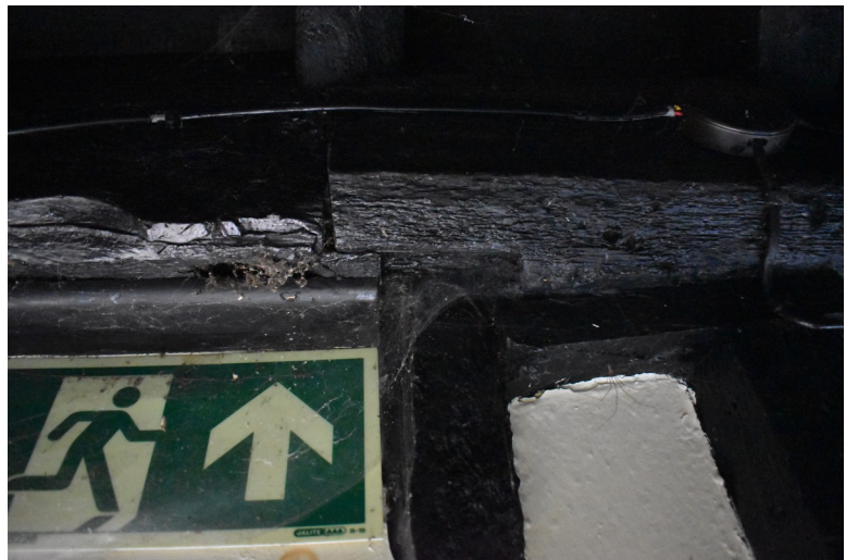
Photograph 18 Detail of partly degraded edge-halved scarf joint in south-east wall-plate of bay 2. Photograph taken facing south-east.
