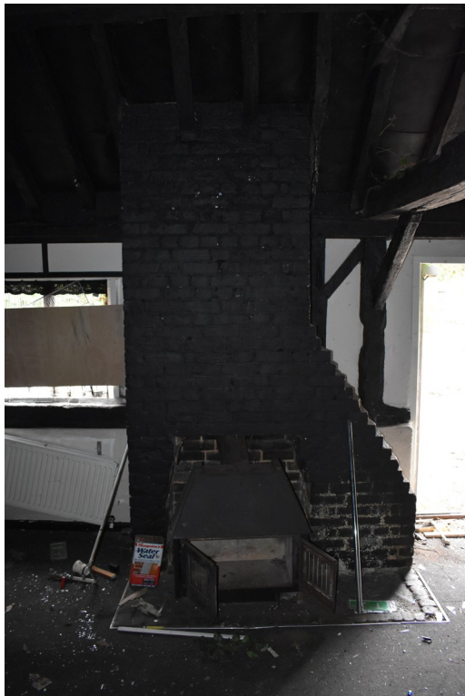
Photograph 15 Detail of inserted fireplace and chimney in south-east end of bay 3. Photograph taken facing south-east.
