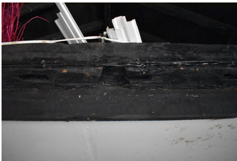
Photograph 11 Underside of tie-beam between bays 3 and 4, showing inverted lap-joint and earlier mortices. Photograph taken facing north-east.
