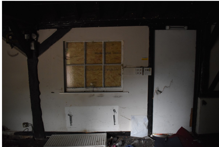
Photograph 8 Interior shot showing north-west elevation of bay 3, showing fixed six-light window. Photograph taken facing north-west.
