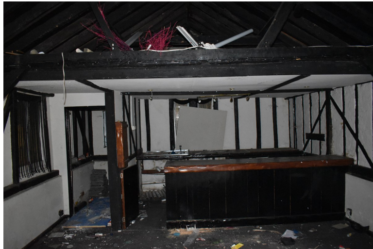
Photograph 16 Detail of bay 4, showing inserted bar, stud wall and attic space. Brick plinths beneath timber-frame rendered. Photograph taken facing north-east.
