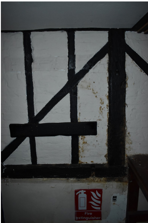
Photograph 17 Detail of inserted brick-nogging on south-east elevation of bay 4. Photograph taken facing south-east.
