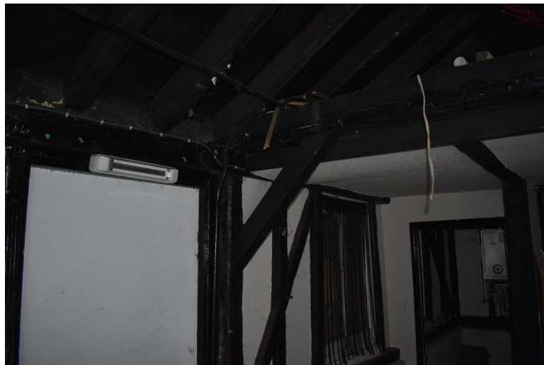
Photograph 13 Detail of machine-cut brace supporting north-west end of tie-beam between bays 3 and 4. Photograph taken facing north.
