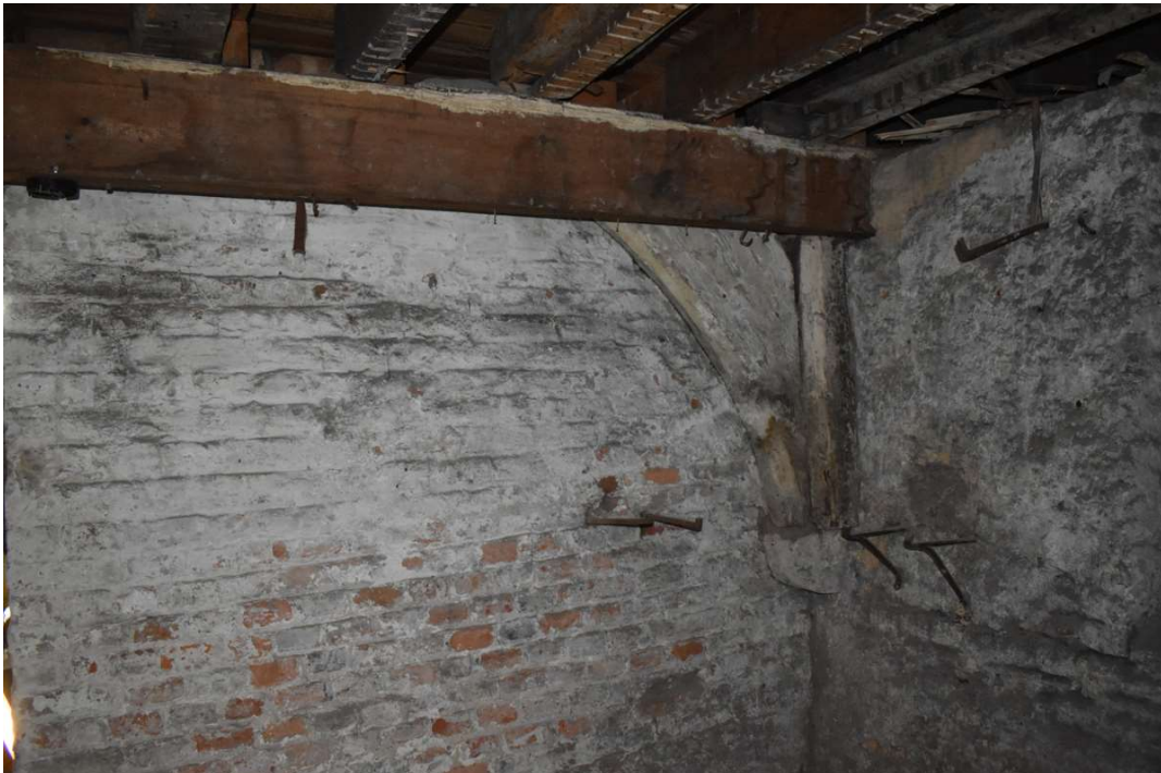
Photograph 21 Detail of western arched-brace between bays 3 and 4, showing original corbel, modern replacement binding-beam and 19th-century brick wall subdividing bays, looking southwest.
