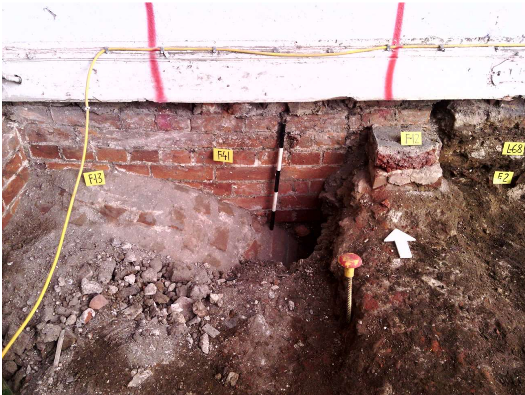
Photograph 3 Well cap F13 with brick underpinning F41 beneath standing wall F42 and plinth F12, looking north.
