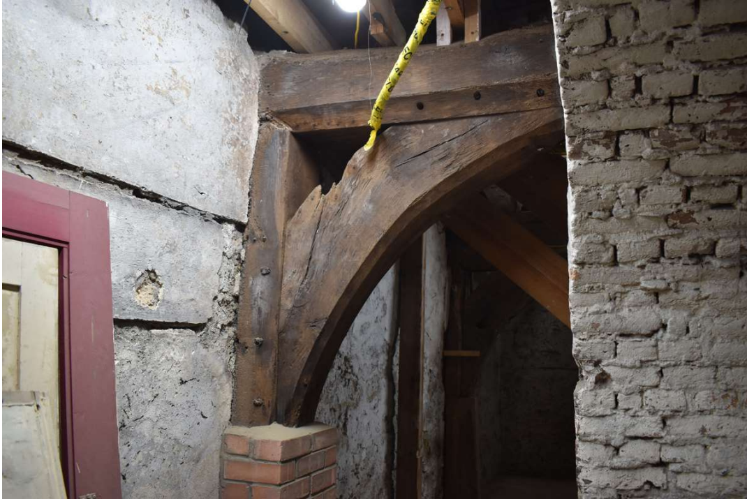
Photograph 20 Detail of arched-brace supporting eastern end of binding-beam between bays 2 and 3. Brick pillar visible below. Looking southeast.
