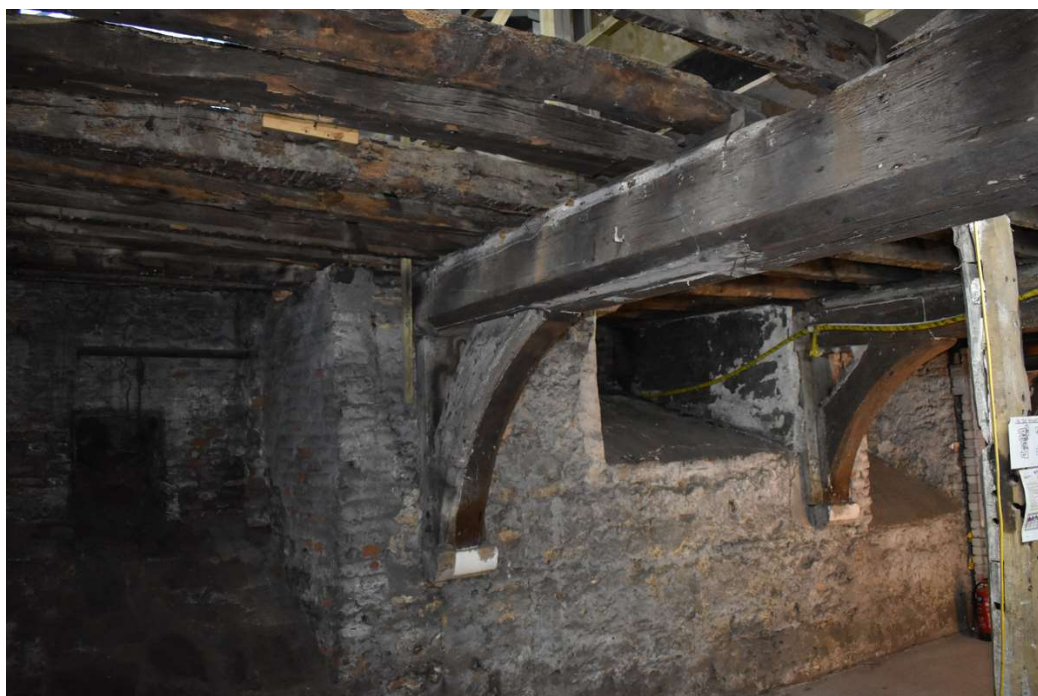
Photograph 18 Bay 1 of cellar, showing access chutes in western wall and arched-brace supporting binding-beam, looking northwest.
