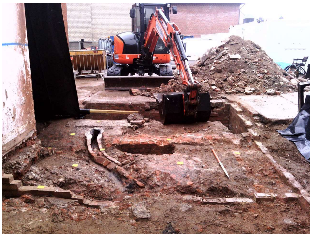
Photograph 4 Brick soakaway F4, drain F16 and wall foundation F17 (Phase 2) surrounded by 20th-century wall foundations F19 in LBC bricks (Phase 3), looking east.
