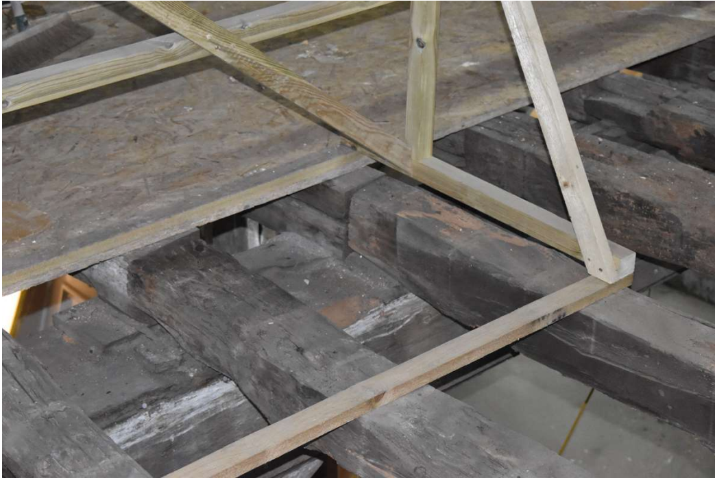
Photograph 27 Detail of abutting joists sitting on the binding-beam between bays 1 and 2. Slight depressions in binding-beam for original joists visible, looking northeast.
