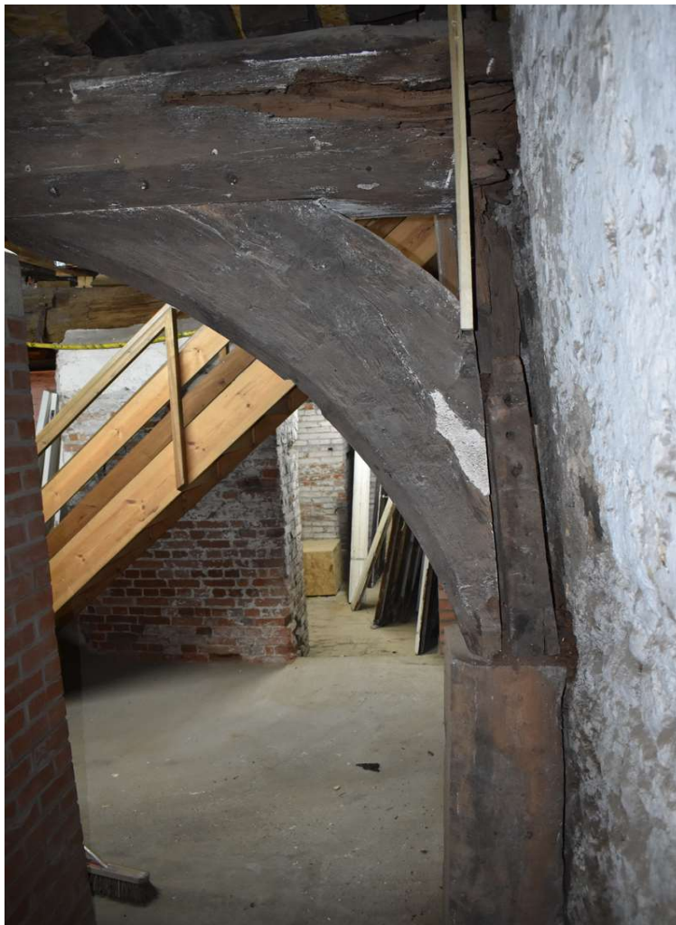
Photograph 19 Detail of eastern brace supporting binding-beam between bays 1 and 2, showing modern post support, looking north.
