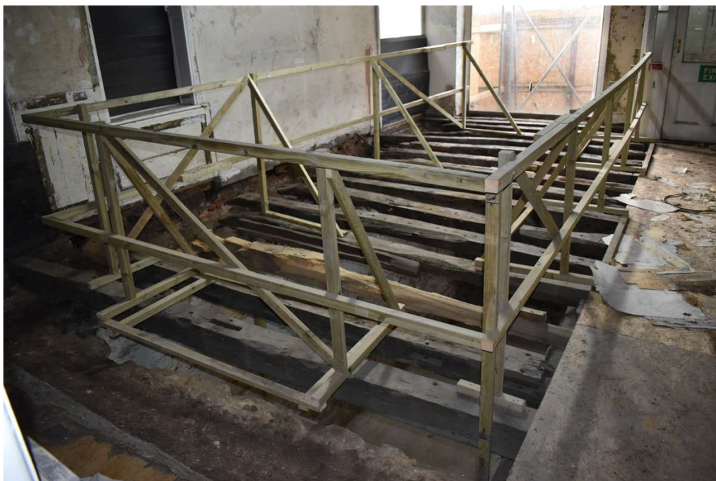
Photograph 24 Section of exposed joists above bay 1 after removal of floorboards, looking southwest.
