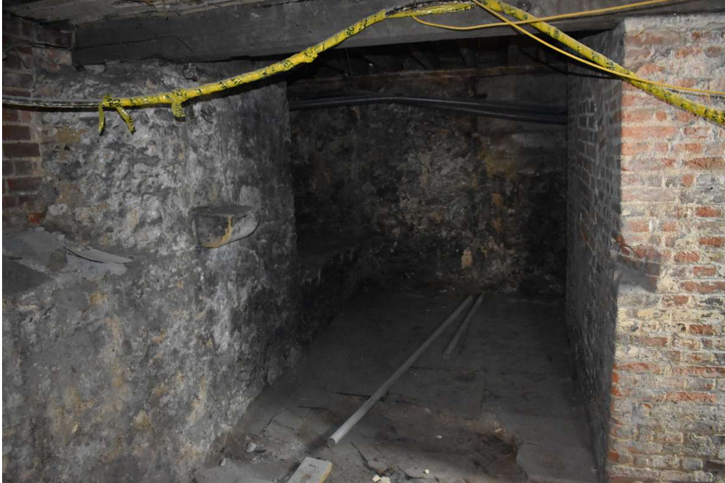
Photograph 22 Bay 5, showing the corbel that would have supported the original truss. Inserted 17th-century brick arch to right, looking north.
