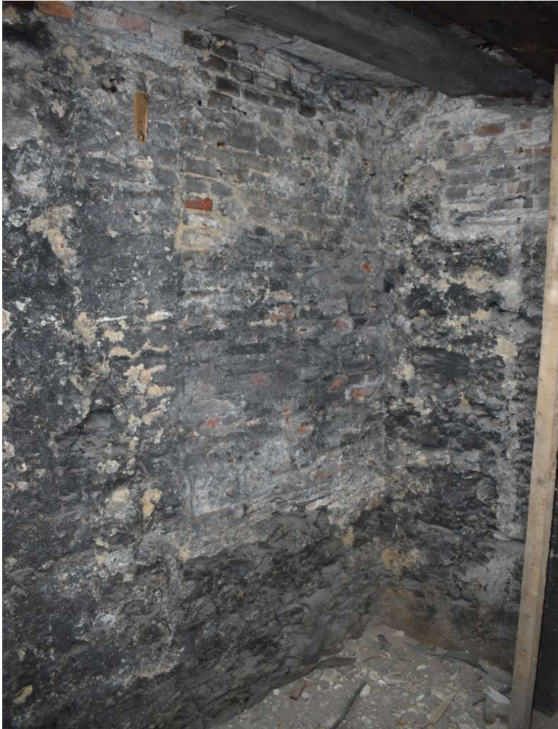
Photograph 34 Detail of brickwork in eastern wall of bay 6, possibly indicating the location of a blocked entranceway into another part of the cellar, looking southeast.
