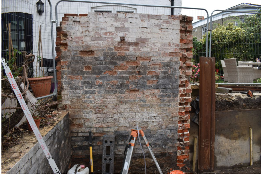
Photograph 4 Detail of red brick wall that was keyed into south end of demolished structure (joints visible on right side of wall). Photograph taken facing south.
