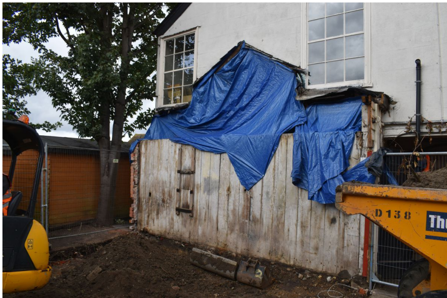
Photograph 5 Detail of northern half of building surviving underneath 1970s first-floor extension. Scar on first-floor shows roof pitches of demolished half. Wooden panel division visible with projecting brick wall visible to left. Photograph taken facing north-west.
