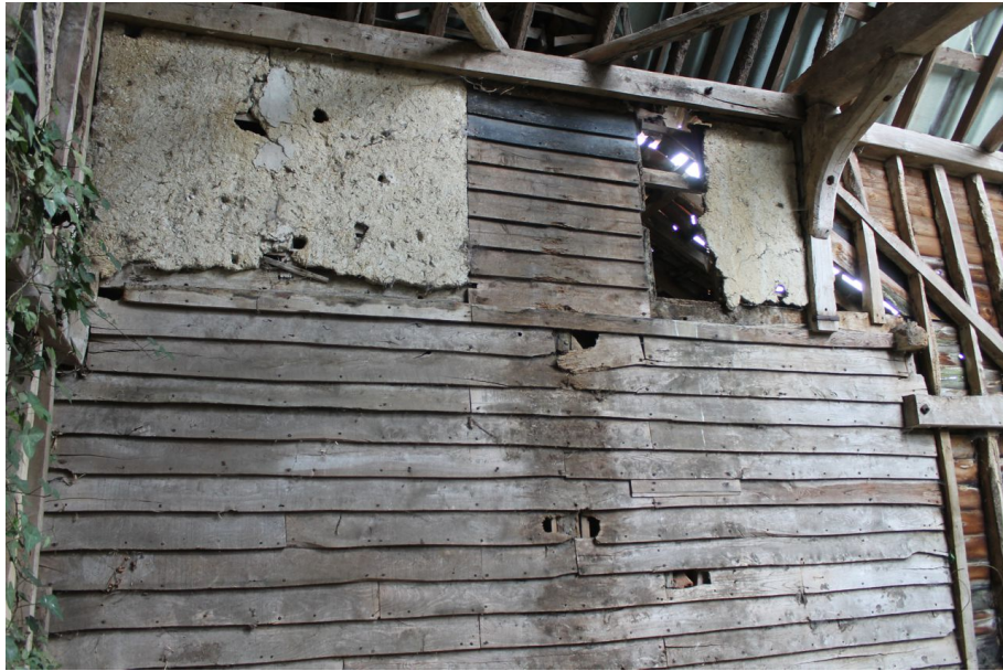
Photograph 8 East elevation of bay 1, showing weatherboarding, patches of lath and plaster and partial principal-post bolted to the frame of the adjacent building. Photograph taken facing east.
