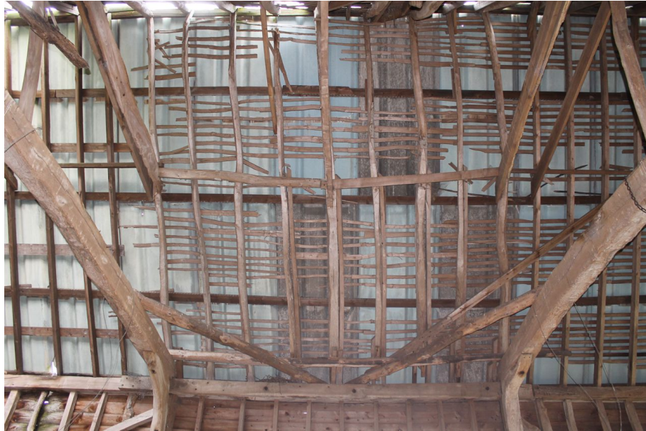
Photograph 4 Eastern roof pitch above bay 3 in threshing barn, showing hand-sawn original rafters, purlin and battens. Photograph taken facing south-east.
