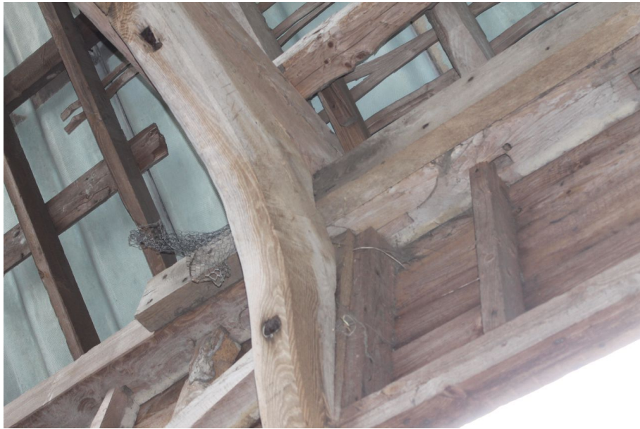
Photograph 10 Detail of scarf joint behind east knee brace supporting tie-beam between bays 2 and 3. "II" carpenter's mark visible on knee brace. Photograph taken facing east.
