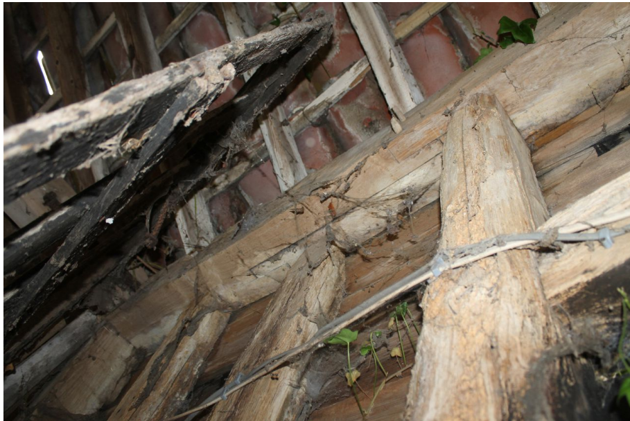
Photograph 34 Detail of scarf joint on northern wall-plate of bay 3. Photograph taken facing north.
