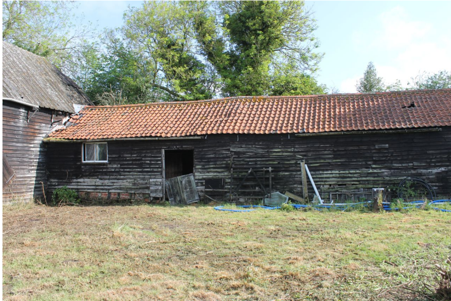
Photograph 20 South-west elevation of the six-bay building. Inserted modern plastic-framed window visible, alongside damaged stable door. Photograph taken facing north.
