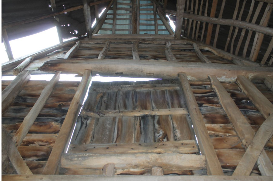
Photograph 18 Detail of underside of wall-plate above pitching door in midstrey, showing mortices. Photograph taken facing north-west.
