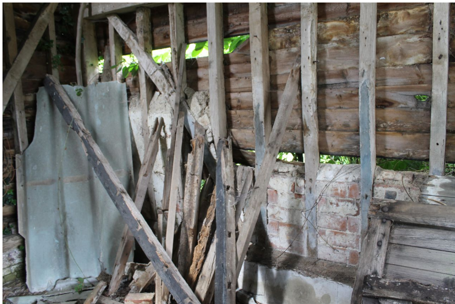
Photograph 19 North elevation of midstrey, showing inserted modern brick-nogging. Photograph taken facing north.
