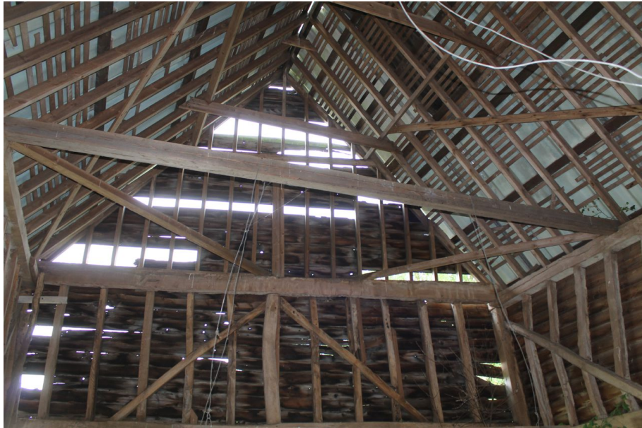
Photograph 6 Inserted modern machine-cut tie-beam between bays 4 and 5. Photograph taken facing south-west.
