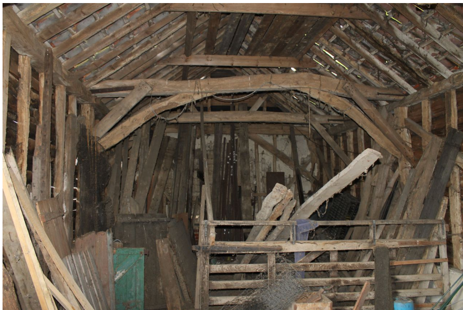
Photograph 25 Centre of structure, showing tie-beam between bays 3 and 4 and behind that, inserted dividing wall. Photograph taken facing north-west.
