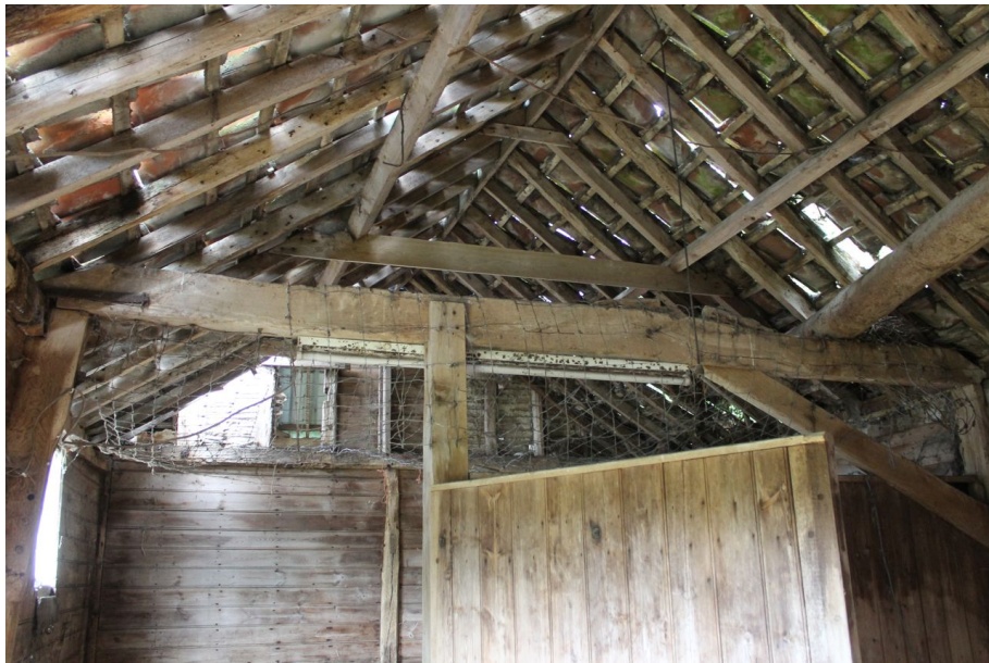
Photograph 24 Tie-beam between bays 1 and 2, with removed southern brace. Photograph taken facing north-west.
