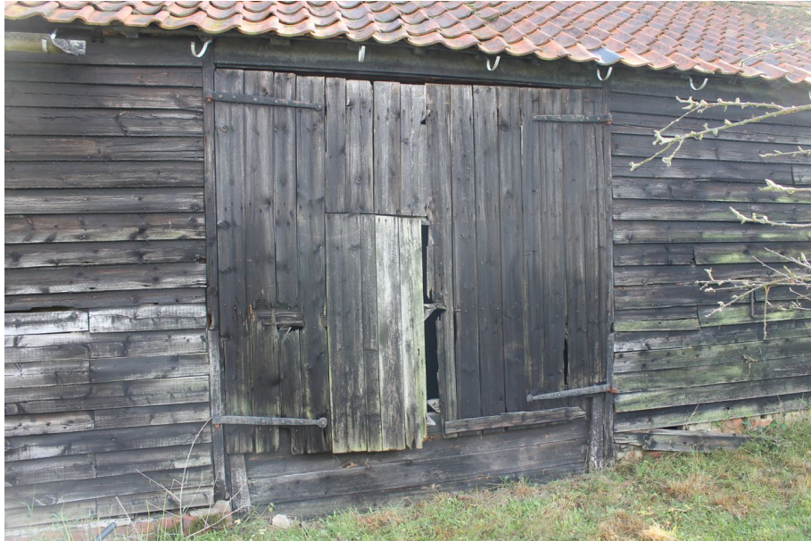
Photograph 22 Barn door on south-west elevation of six-bay building. Photograph taken facing north-east.
