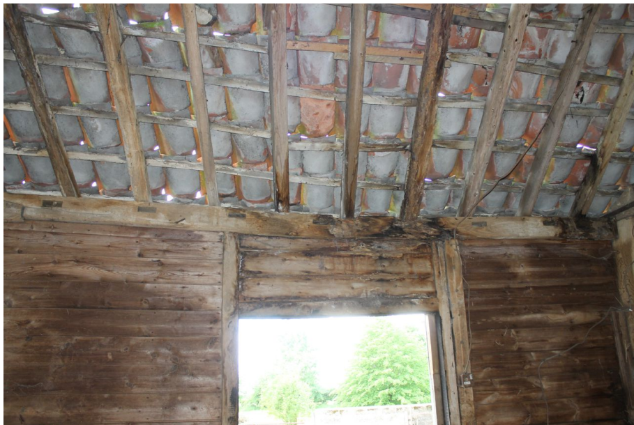
Photograph 30 Detail of rudimentary scarf joints on southern wall-plate of bay 2, with short length of reused timber between them. Photograph taken facing south-west.
