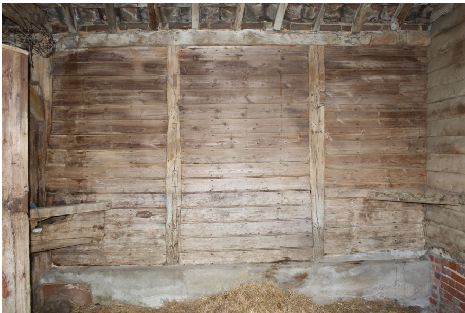
Photograph 27 Northern elevation of bay 2, showing internal timber panelling and reused intermediate posts. Photograph taken facing north-east.
