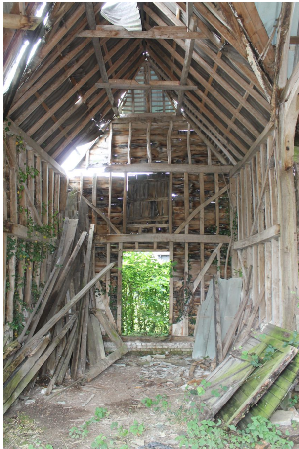
Photograph 17 Midstrey of barn, showing inserted pitching door on upper register. Photograph taken facing north-west.
