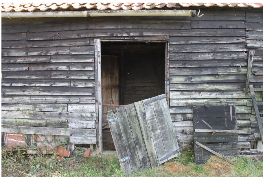
Photograph 23 Detail of damaged stable door on south-west elevation of six-bay building. Exposed timber-frame and brick-nogging visible to left. Photograph taken facing north-east.
