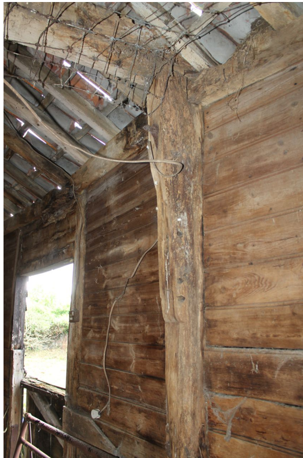
Photograph 28 Detail of jowled principal-post on south elevation between bays 1 and 2, with removed brace. Photograph taken facing south.
