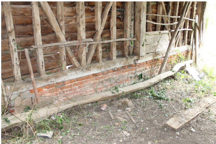
Photograph 15 Detail of brick plinth and sill-beam on east elevation of bays 4 and 5. Rudimentary scarf joint visible in centre of sill-beam. Photograph taken facing south.
