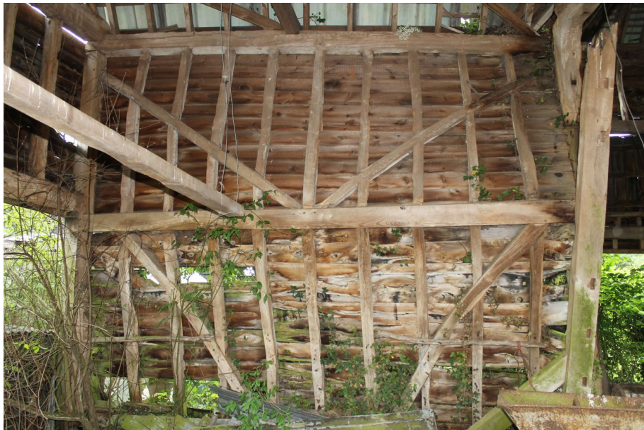
Photograph 13 West elevation of bays 4 and 5. Note lack of principal-post and single girding-beam bridging both bays. Photograph taken facing north-west.
