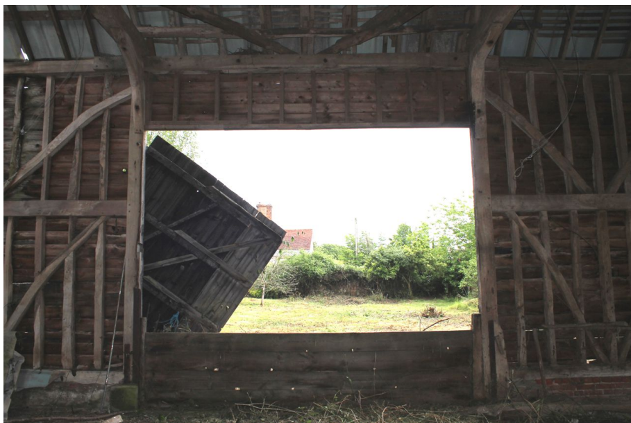
Photograph 11 East elevation of bay 3, showing barn doors. Machine-cut studs visible above. Photograph taken facing south-east.
