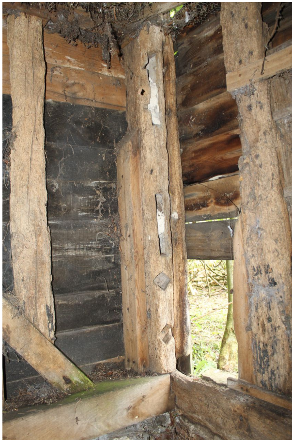
Photograph 37 South-east corner post of building in bay 6, showing diamond mullion mortices. Photograph taken facing south.
