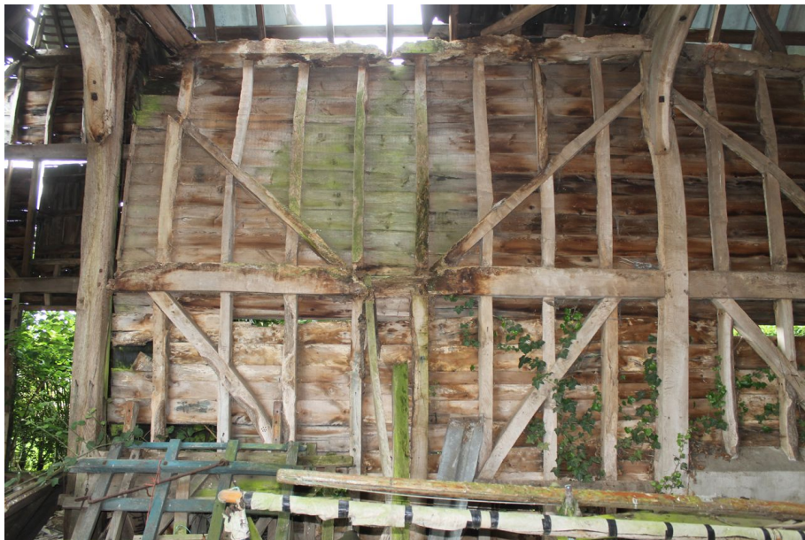
Photograph 9 West elevation of bay 2, showing extensive water damage to wall-plate and girding-beam. Photograph taken facing north-west.
