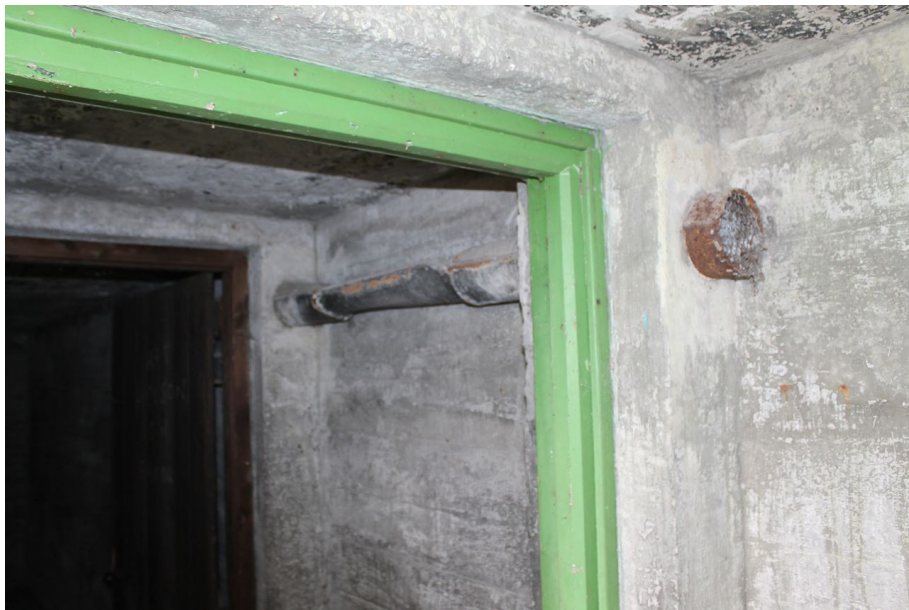
Photograph 8 Detail of inserted metal vent and pipe in north of air-raid shelter, adjacent to entrance. Photograph taken facing south-west.
