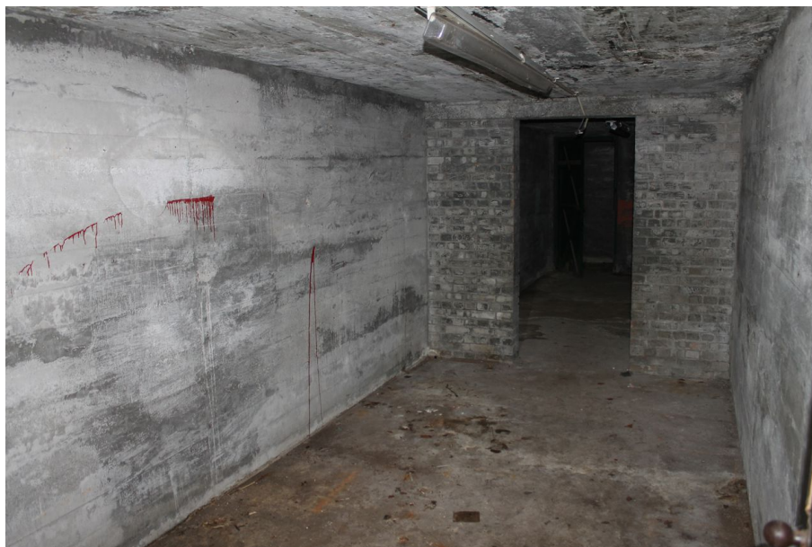
Photograph 3 Interior of air-raid shelter, showing dividing brick wall. Photograph taken facing south-east.
