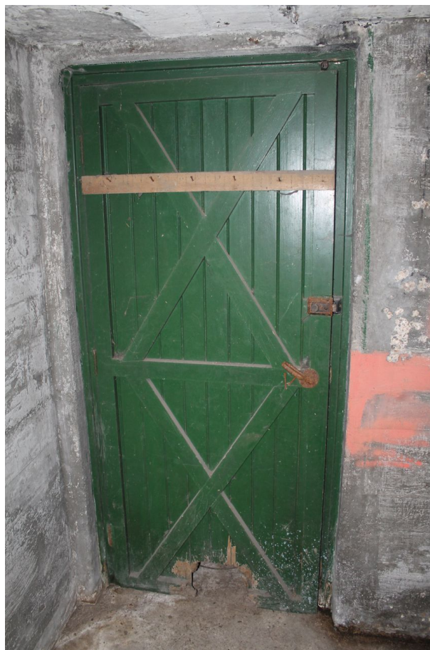
Photograph 6 Detail of southern door on interior of air-raid shelter, showing cross-battens on rear. Photograph taken facing south.
