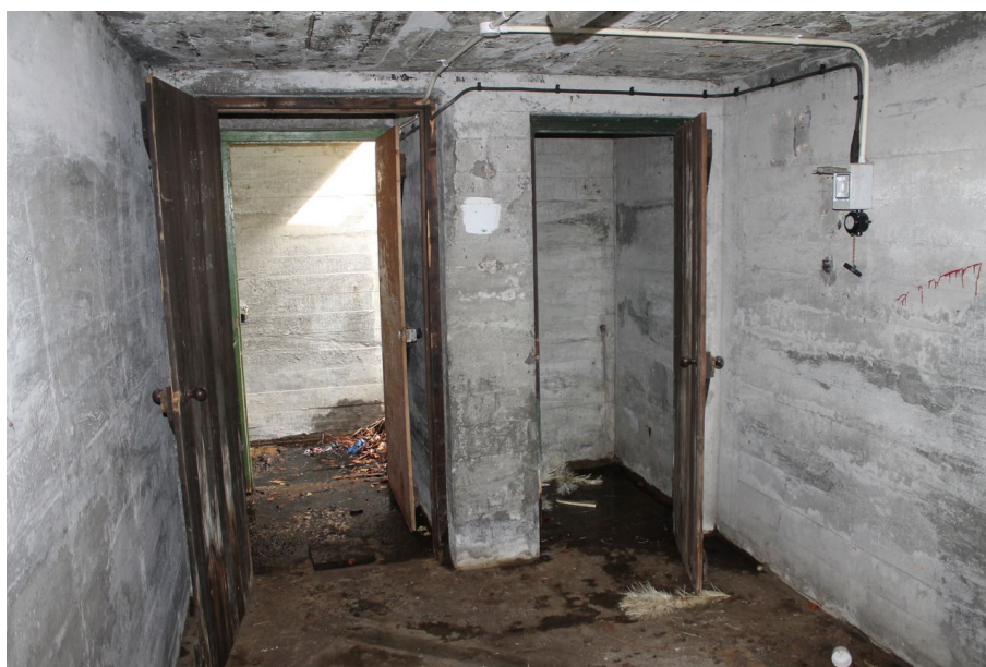
Photograph 4 Interior of air-raid shelter, showing separate room next to northern entrance. Photograph taken facing north-east.
