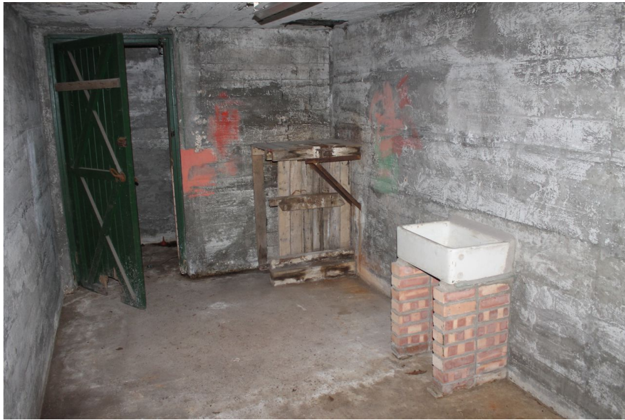
Photograph 5 Interior of air-raid shelter, showing inserted sink and desk in south of structure. Photograph taken facing south-west.
