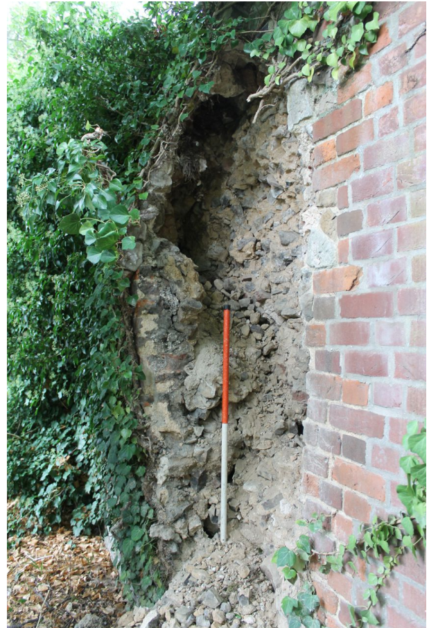
Photograph 3 Collapsed section of wall prior to recording and reduction in height for stabilisation. Photograph taken facing north-east.
