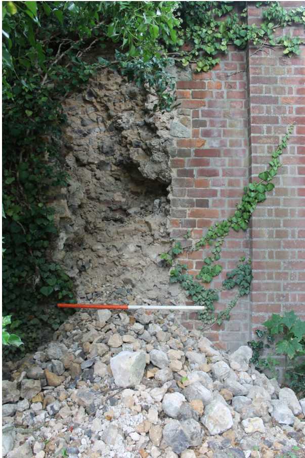
Photograph 2 Collapsed section of wall prior to recording and reduction in height for stabilisation. Photograph taken facing east.
