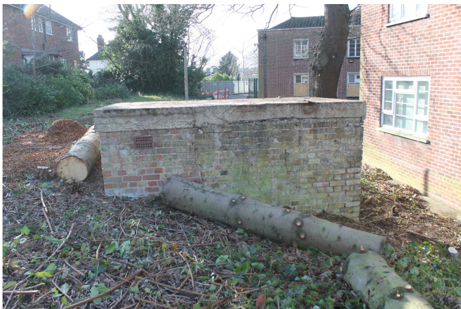
Photograph 2 North-west elevation of air-raid shelter, showing differing types of brickwork. Photograph taken facing south-east.
