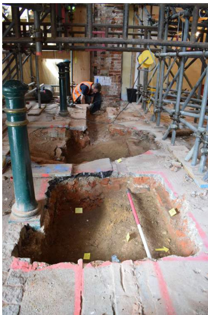
Photograph 16 Pad F showing brick wall foundation F12 (Phase 3) to the north and trench F13 for the demolished 1905 shop façade to the south, looking west.
