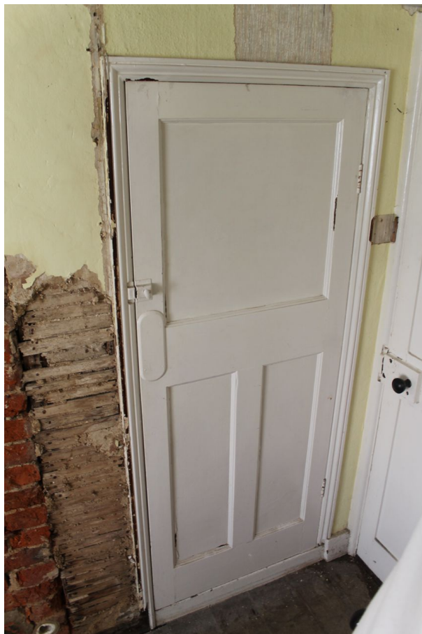
Photograph 11 Detail of three-panel door leading into cupboard extension. Photograph taken facing west.
