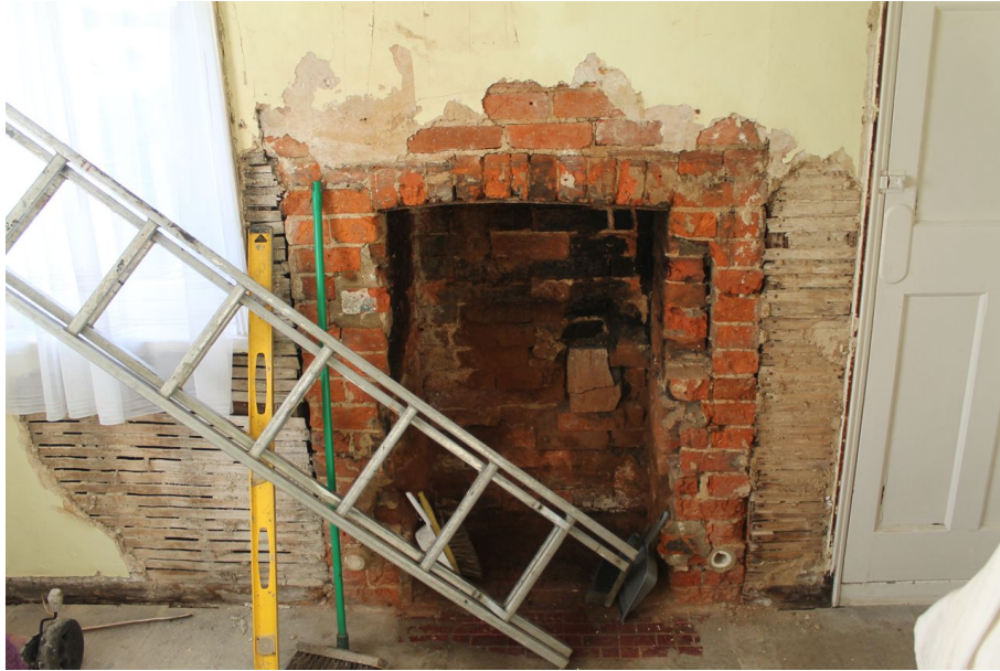
Photograph 10 Detail of brick fireplace in south-west room on ground-floor. Photograph taken facing south-west.
