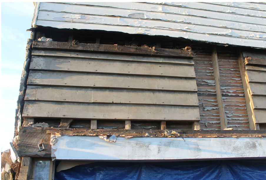
Photograph 7 Detail of timber-framing on upper register of north-east elevation, showing primary-bracing. Photograph taken facing south-west.
