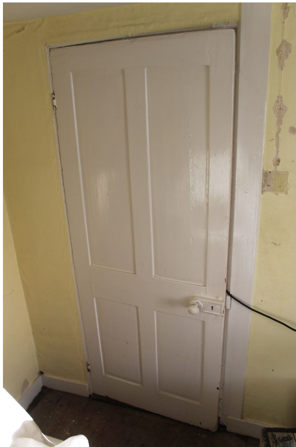
Photograph 13 Four-panel door between south-west room and entrance hall on ground-floor. Photograph taken facing north.
