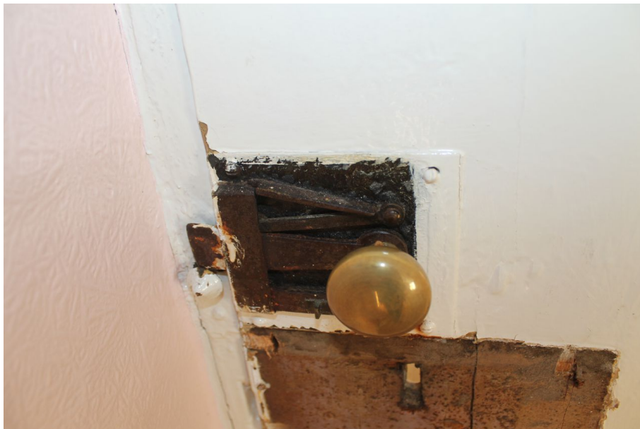
Photograph 21 Detail of spring lock on door in south-west room on first-floor. Photograph taken facing north-east.
