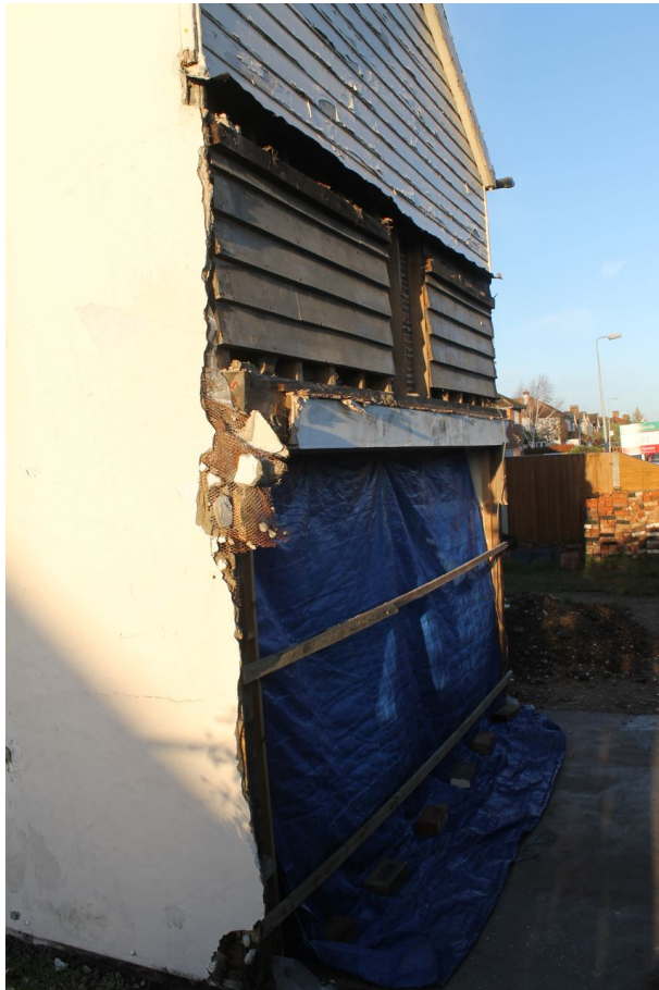
Photograph 6 North-east elevation of building. Lower register entirely removed, timber framing partially visible on upper register. Photograph taken facing west.
