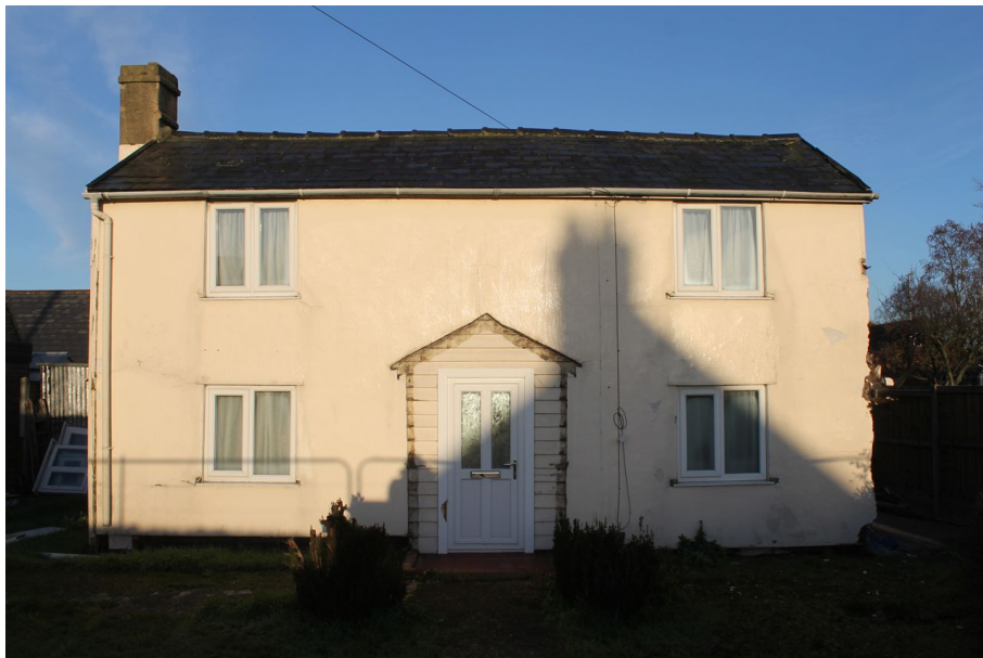
Photograph 1 South-east elevation of building. Modern windows and door visible, along with scar left by demolition of porch.
