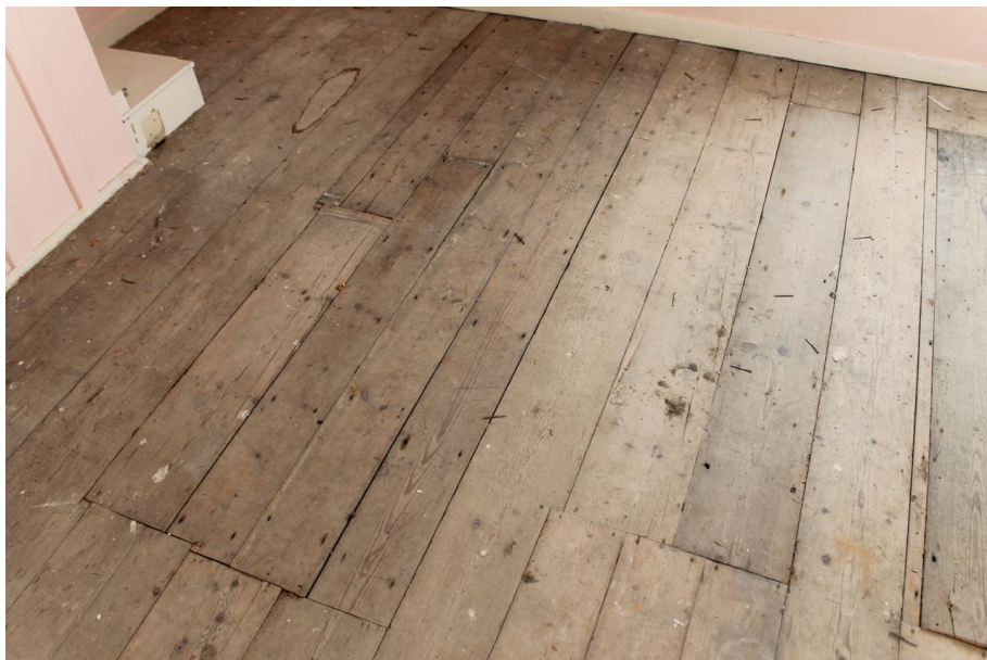
Photograph 19 Varying floorboard widths in south-west room on first-floor. Photograph taken facing east.
