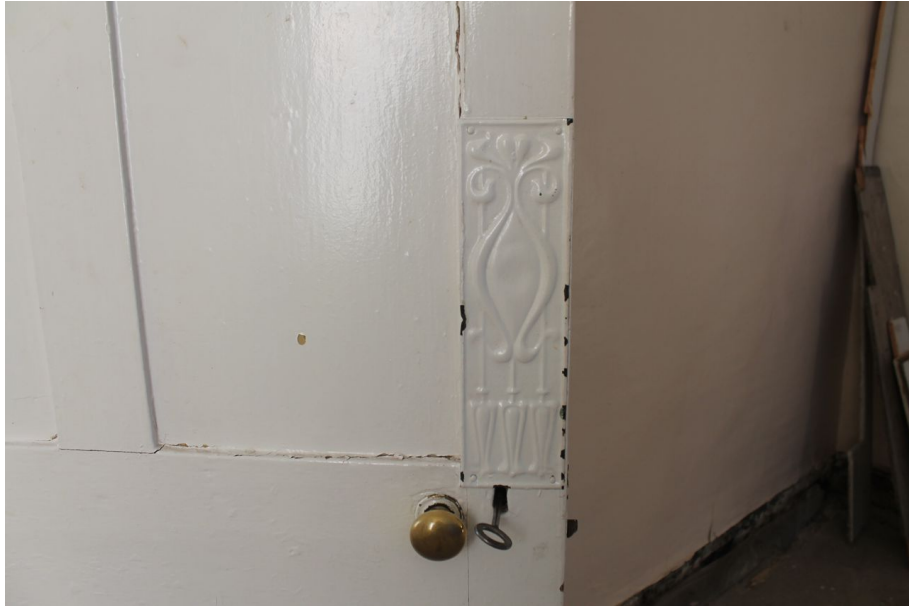
Photograph 14 Detail of embossed metal panel on door between north-east room and entrance hall on ground-floor. Photograph taken facing west.
