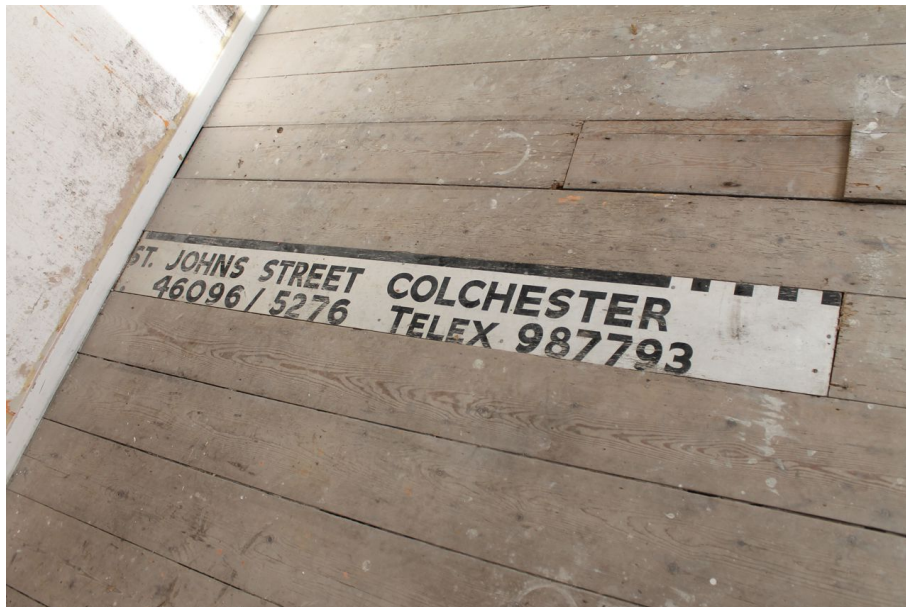
Photograph 16 Detail of replacement floorboard in north-east room on first-floor. Photograph taken facing north-east.
