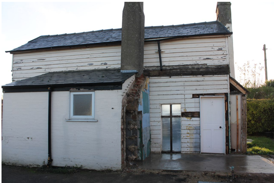
Photograph 3 North-west elevation of building. Demolished kitchen extension visible to right. W.C. extension visible to left. Photograph taken facing south-east.
