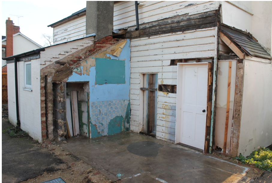
Photograph 4 Location of demolished kitchen extension. Four-panel door visible, as well as brick chimney of kitchen. Photograph taken facing east.
