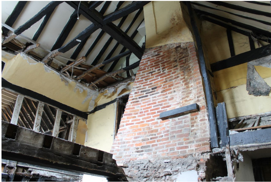
Photograph 41 Chimney stack in Structure A after soft strip. Photograph taken facing north.
