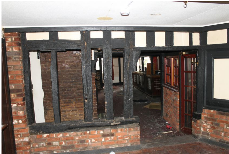
Photograph 18 Original stud-work viewed from Structure B. Inserted modern timber clear, as is original header for doorway. Photograph taken facing south-east.
