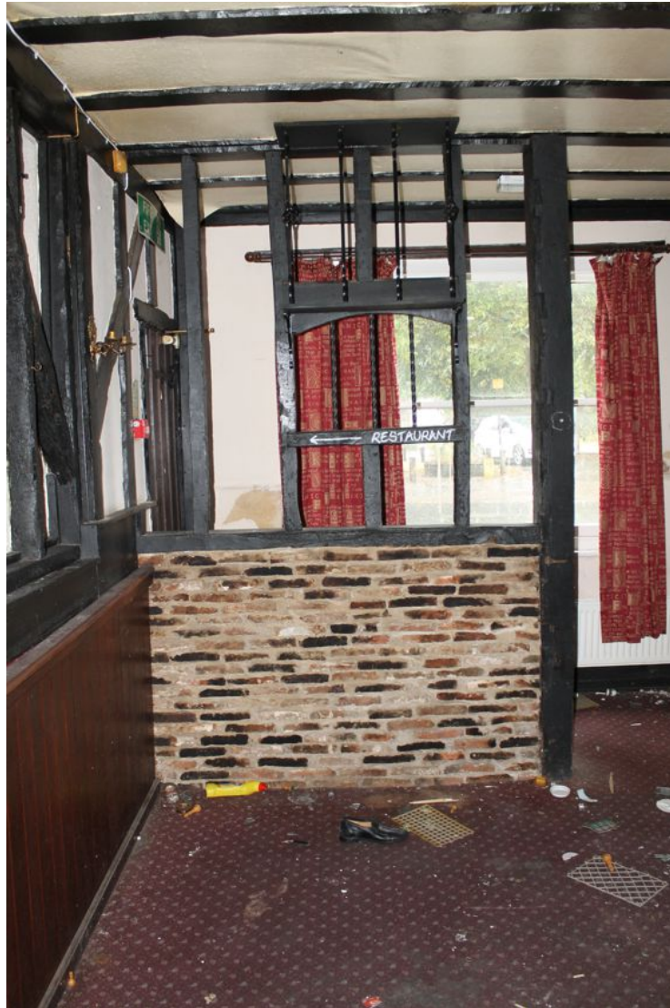
Photograph 39 Modern wall in Structure F consisting of re-used bricks and a re-used tie-beam (to right). Photograph taken facing south-east.
