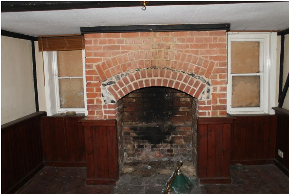
Photograph 27 Repaired fireplace on north-west ground-floor elevation of Structure B. Photograph taken facing north-west.
