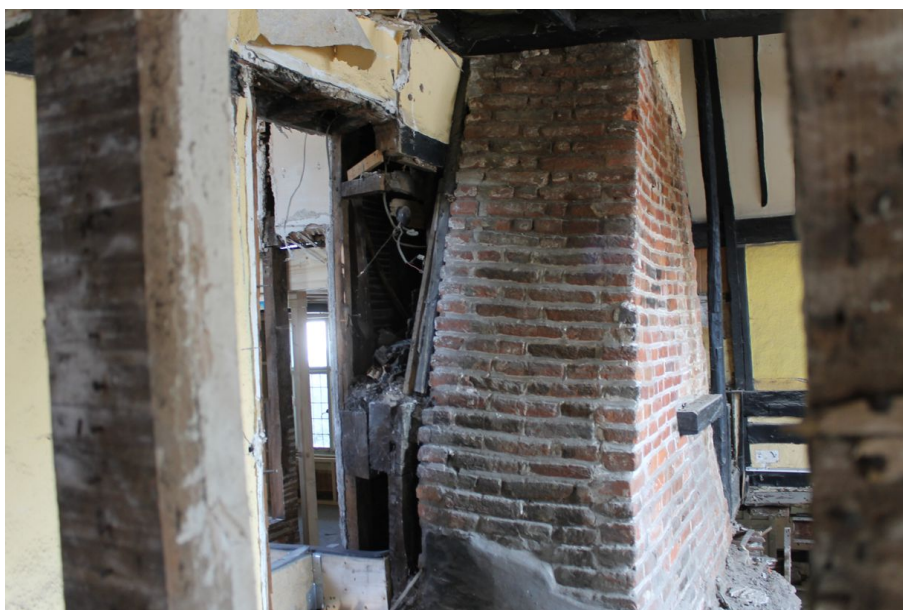
Photograph 49 Detail of north-west side of chimney stack, showing beams and surviving plaster behind in Structure A. Photograph taken facing east.
