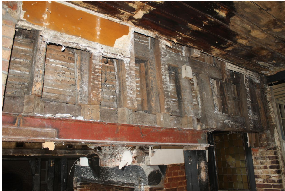
Photograph 42 Exposed partially surviving studs and girding-beam on south-east elevation of Structure A after soft strip. Photograph taken facing north.
