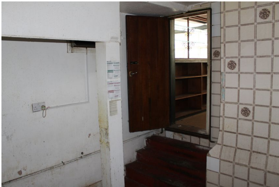
Photograph 35 Photo showing floor-level difference between Structure D and Structure C. Photograph taken facing east.
