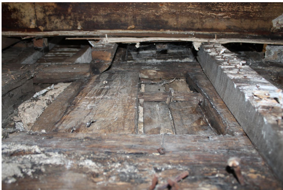
Photograph 44 Detail of timber panelling infill on south-east elevation of Structure A, showing grooves for planks and strap. Photograph taken facing north-west.
