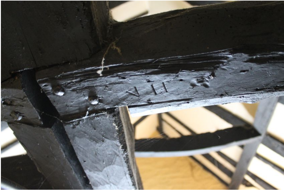
Photograph 22 Detail showing carpenter's mark "VII" on underside of brace to collar-purlin. Photograph taken facing north-east.
