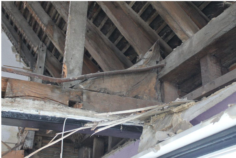
Photograph 55 Detail of inverted knee brace on south-eastern end of the northernmost tie-beam in Structure C. Photograph taken facing north-east.
