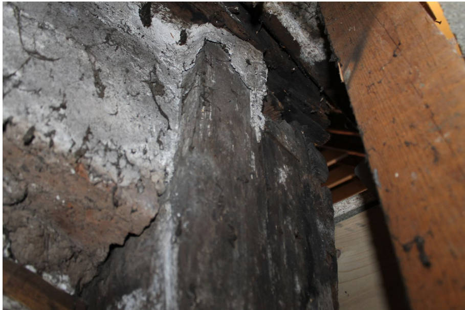
Photograph 48 Detail of mortice on northern corner-post of Structure A, possible for supporting girding-beam of northern wing. Photograph taken facing west.
