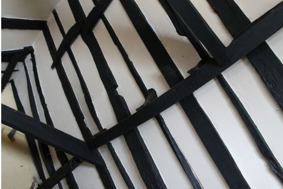
Photograph 24 North-west pitch of Structure A's roof. Showing later bracing, collars and purlin. Photograph taken facing west.
