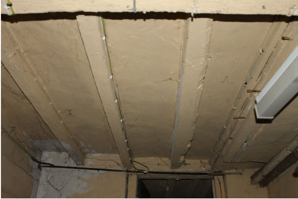
Photograph 31 Underside of ground-floor of Structure C, observed from cellar. Re-used timbers visible. Photograph taken facing north-west.
