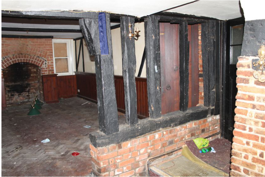
Photograph 17 Section of surviving original stud-work in north-west wall of Structure A. Modern inserted timber blocking doorway second from right. Mortise for brace supporting original first-floor highlighted in blue. Photograph taken facing north.
