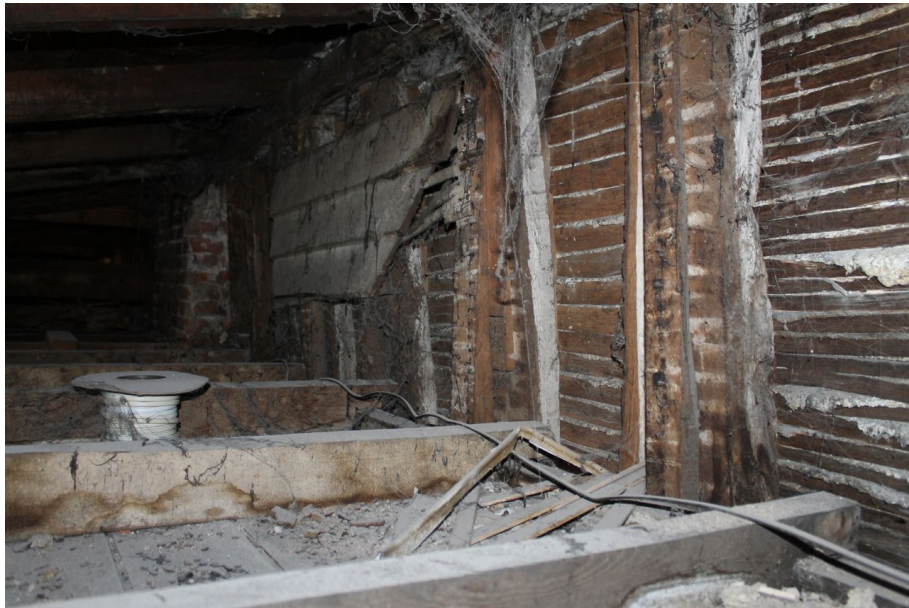
Photograph 45 Upper register of Structure A's south-east elevation, showing surviving weatherboarding. Photograph taken facing west.
