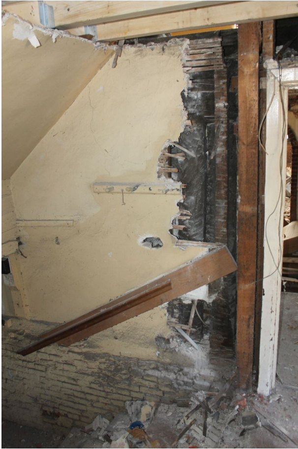
Photograph 53 Partially exposed sill-beam and reused studs behind fireplace in Structure A, supported on the 16th century cellar walls. Photograph taken facing south-east.
