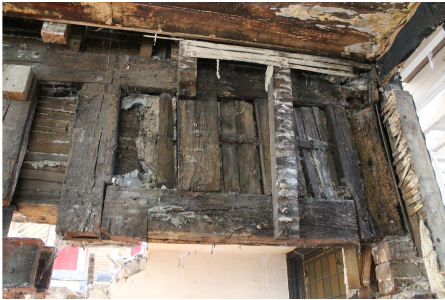
Photograph 43 Detail of timber panelling infill on south-east elevation of Structure A, above original doorway lintel. Photograph taken facing north-west.
