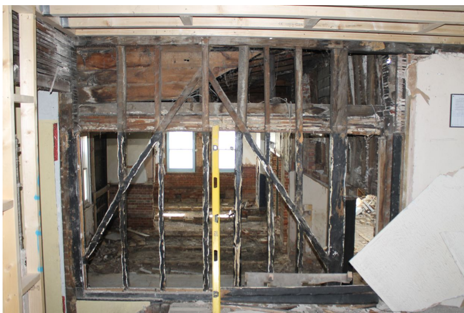
Photograph 59 Timber-framing in north-east end of Structure F, showing machine-cut timbers that have been altered to appear hand-sawn. Photograph taken facing south-west.
