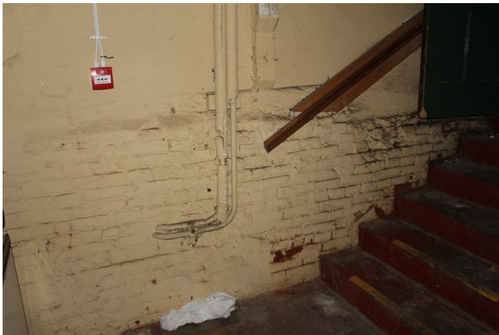
Photograph 29 English-bond brickwork on south-west elevation of cellar, probably associated with Structure A. Photograph taken facing south-west.
