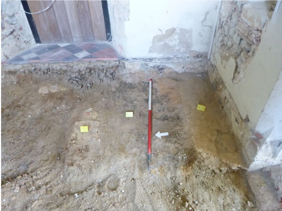
Photograph 3 Detailed shot of lime mortar (F2) and brick pads (F1) in south-east corner of Chapel. Photograph taken facing east.
