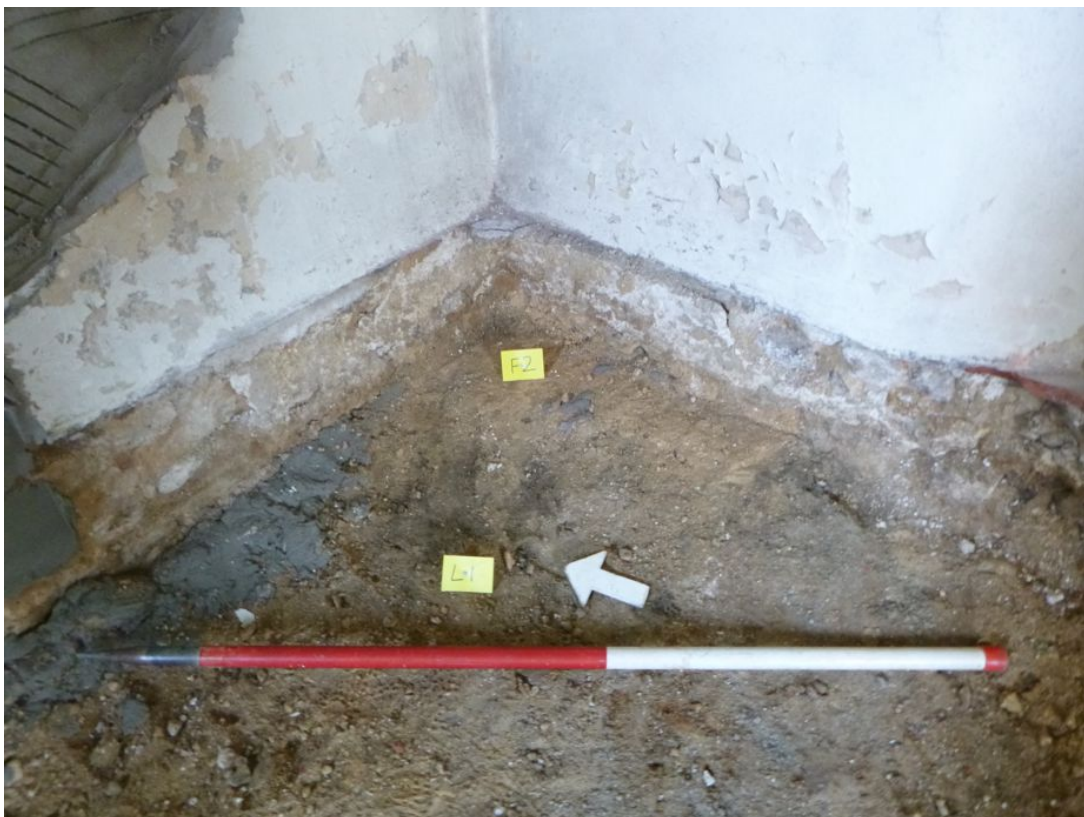
Photograph 4 Detailed shot of lime mortar (F2) in north-east corner of Chapel. Photograph taken facing north-east.
