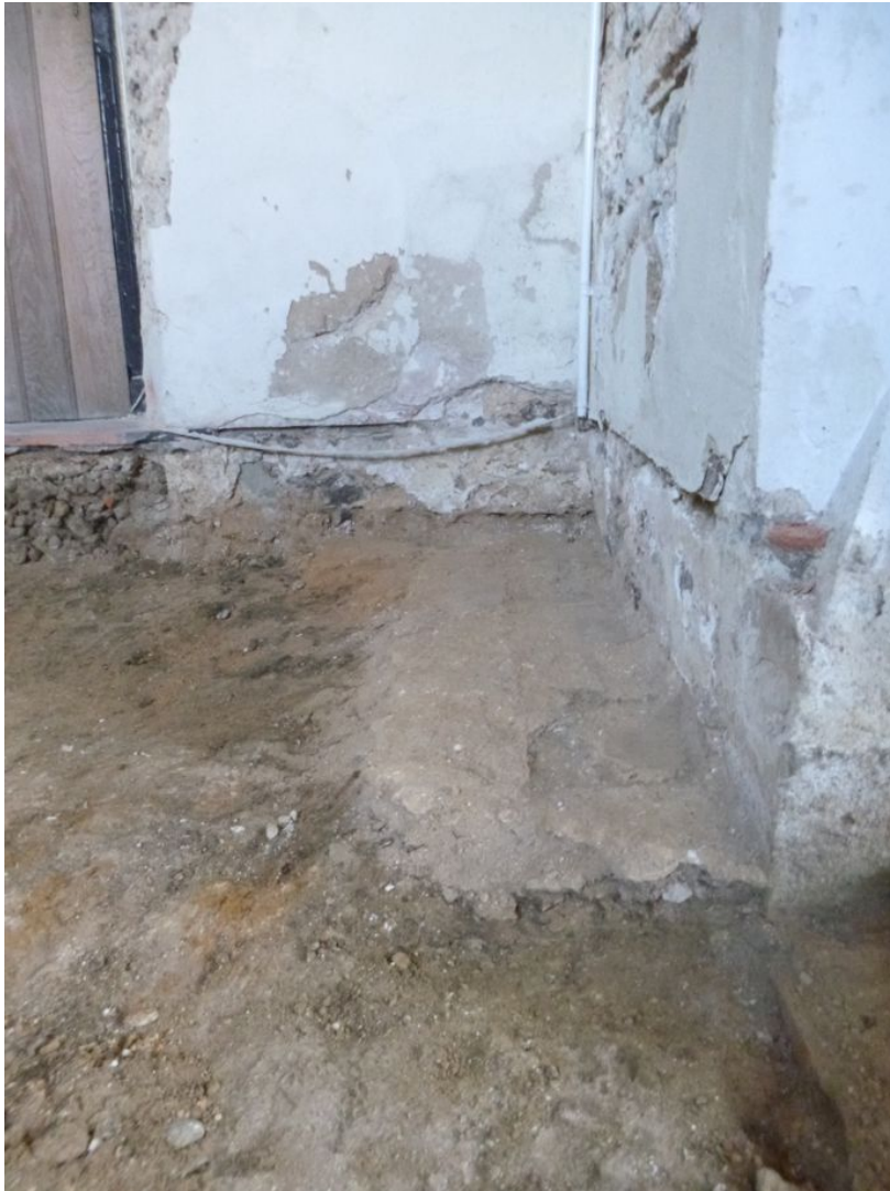
Photograph 5 Section of lime mortar (F2) in south-east corner of Chapel, showing thickness. Photograph taken facing east.
