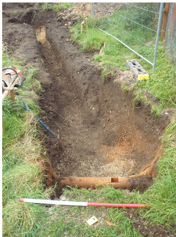
Photograph 3 Drainage trench, showing shallower east end and original service run to be diverted. Photograph taken facing north-west.
