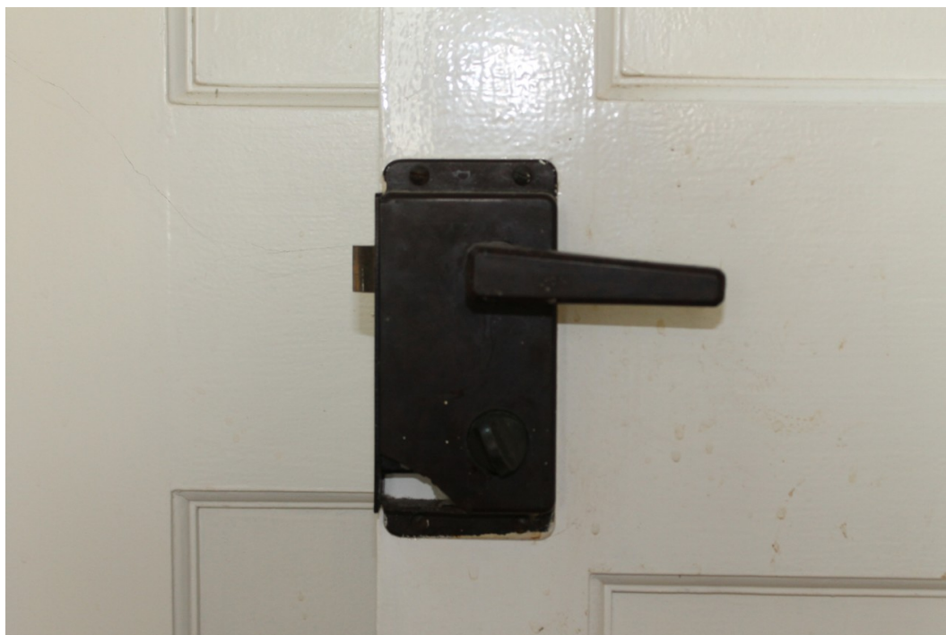
Photograph 19 Bakelite door handle and locking mechanism on the interior of the bathroom door to No.4 Winnocks.
