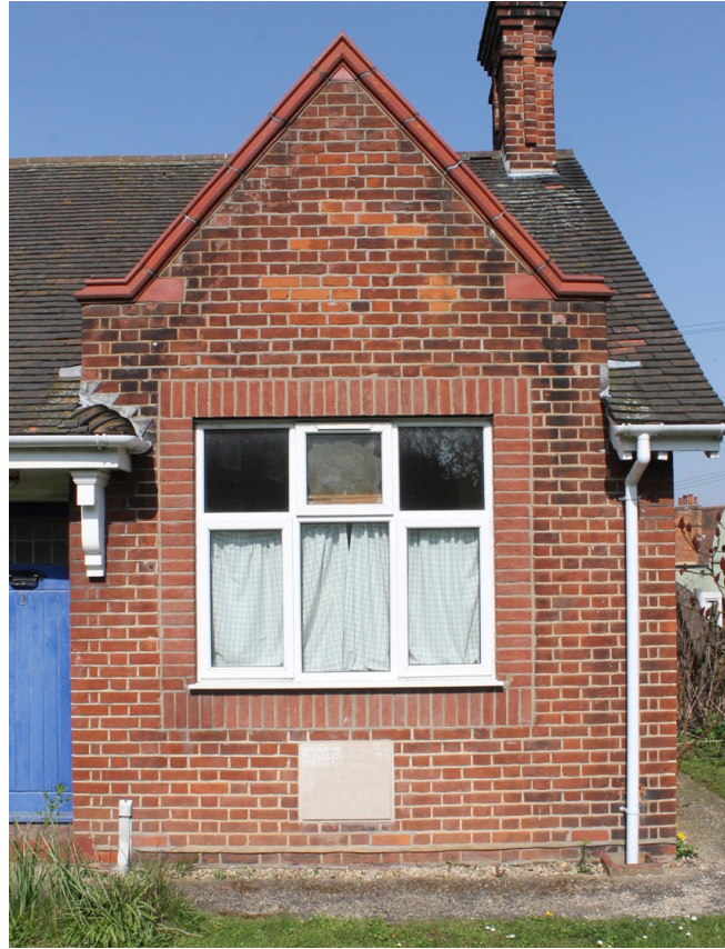
Photograph 5 Replacement UPVC window and brick surround to No.1 Winnocks – view north-west.
