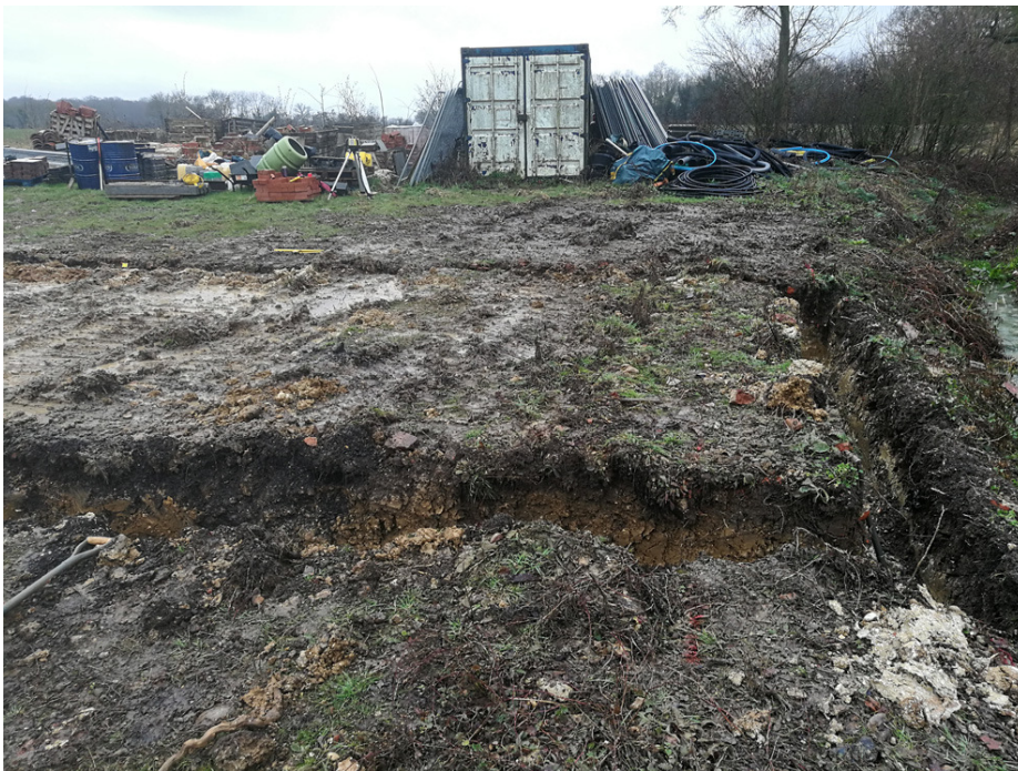
Photograph 3 Overview, showing the northern extent of site and drainage ditch, looking W
