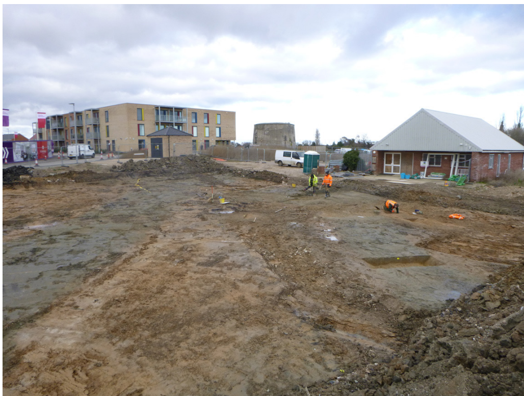
Photograph 1 Southeastern corner of the excavation area with L5 on the left and F24 on the right, looking NE.
