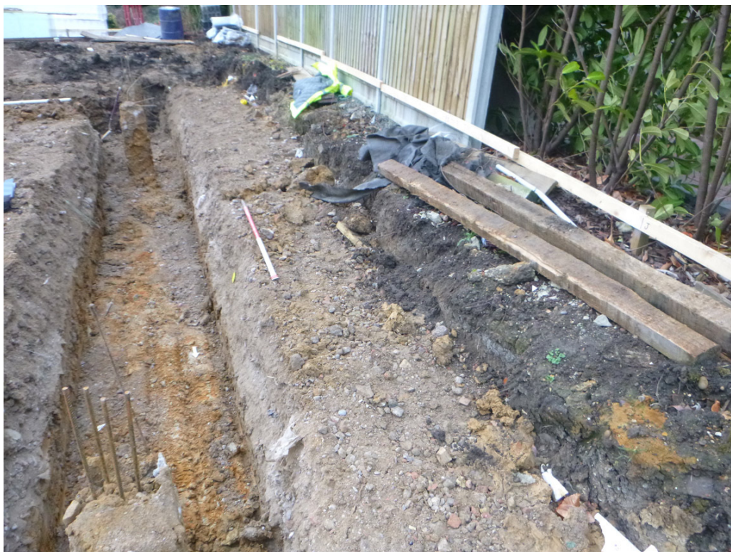
Photograph 1 Foundation trenches excavated through the piling mat onto natural. Previous ground level is shown around the edge of the site boundary.
