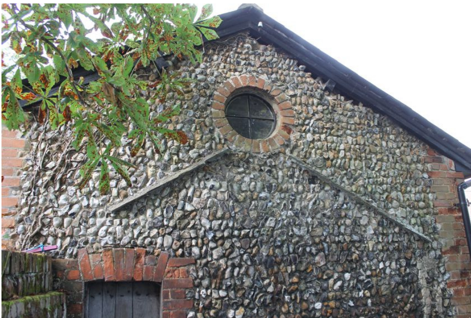
Photograph 5 Detail of northeast elevation of outbuilding and outshot, showing window, scarring and hatch – looking west.
