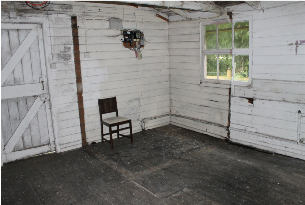
Photograph 7 Recently removed division in the south-east corner of Mission Hall. Shot taken facing south-east.
