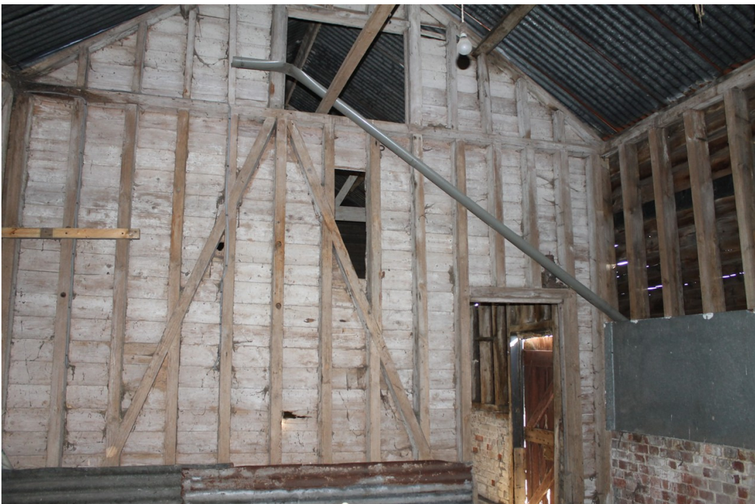
Photograph 28 South-west framing of bay 9, with the locations of the primary bracing indicating that the doorway to the right is an original feature – view north-east.
