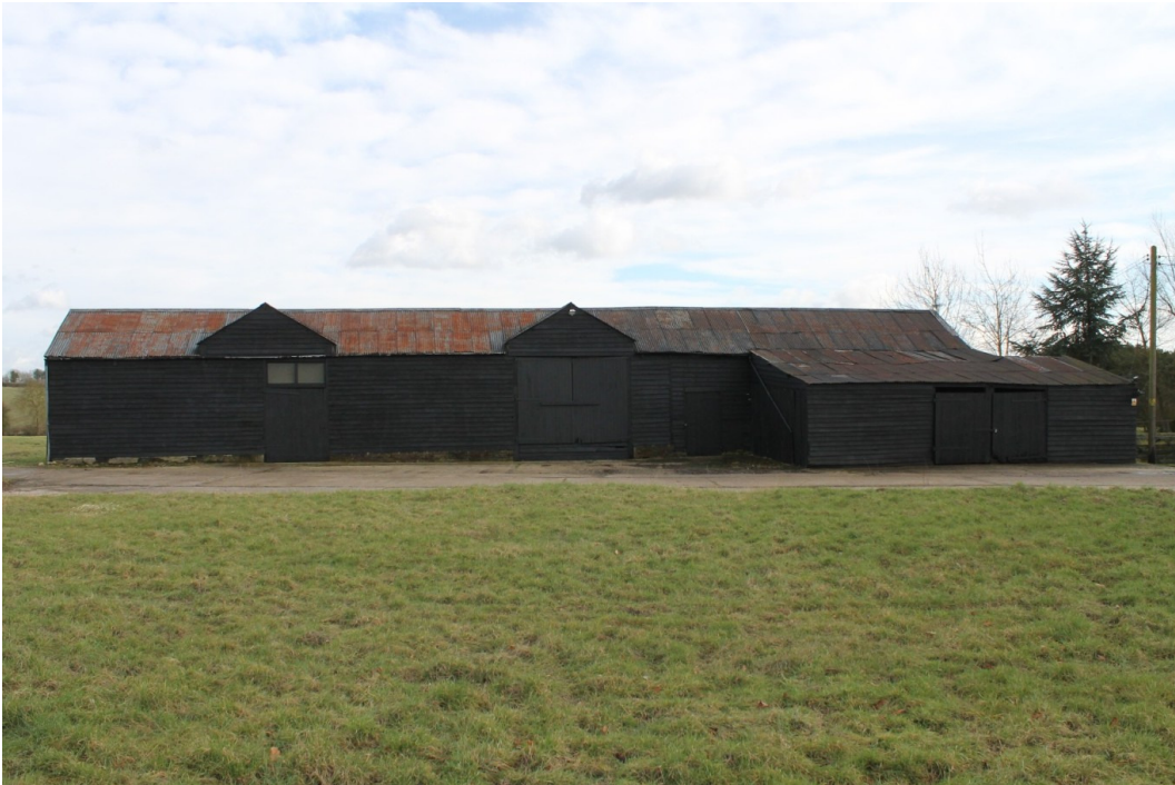
Photograph 1 North-west elevation of the barn, with OB1 to the right - view south-east.
