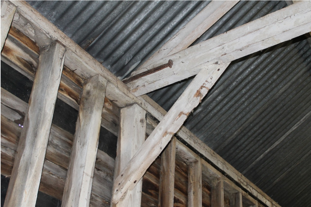
Photograph 11 Nailed brace to south-east post of truss B and iron cramp to later tie beam - view south-east.
