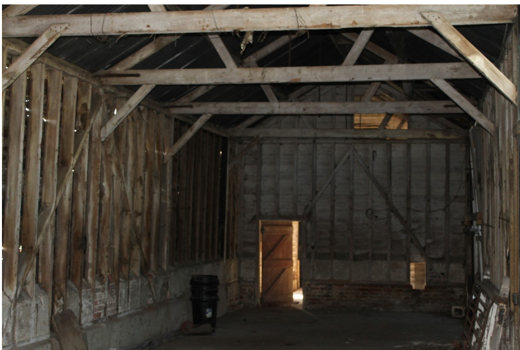
Photograph 8 Interior of the 18th-century barn, with the 19th-century extensions behind the gable frame – view south.
