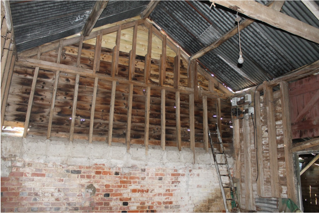
Photograph 29 South-east frame of bay 10, constructed upon the rear wall of the 18th-century brick stable block – view south-west.
