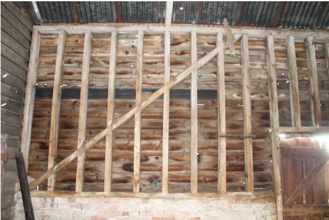
Photograph 26 South-east framing of bays 7 and 8 showing the frame built up against the exterior of the main barn and sitting on a much taller brick plinth, which is probably an earlier farmyard wall. The doorway to the right appears to be an original opening through this wall. The primary bracing crosses both bays – view south-east.
