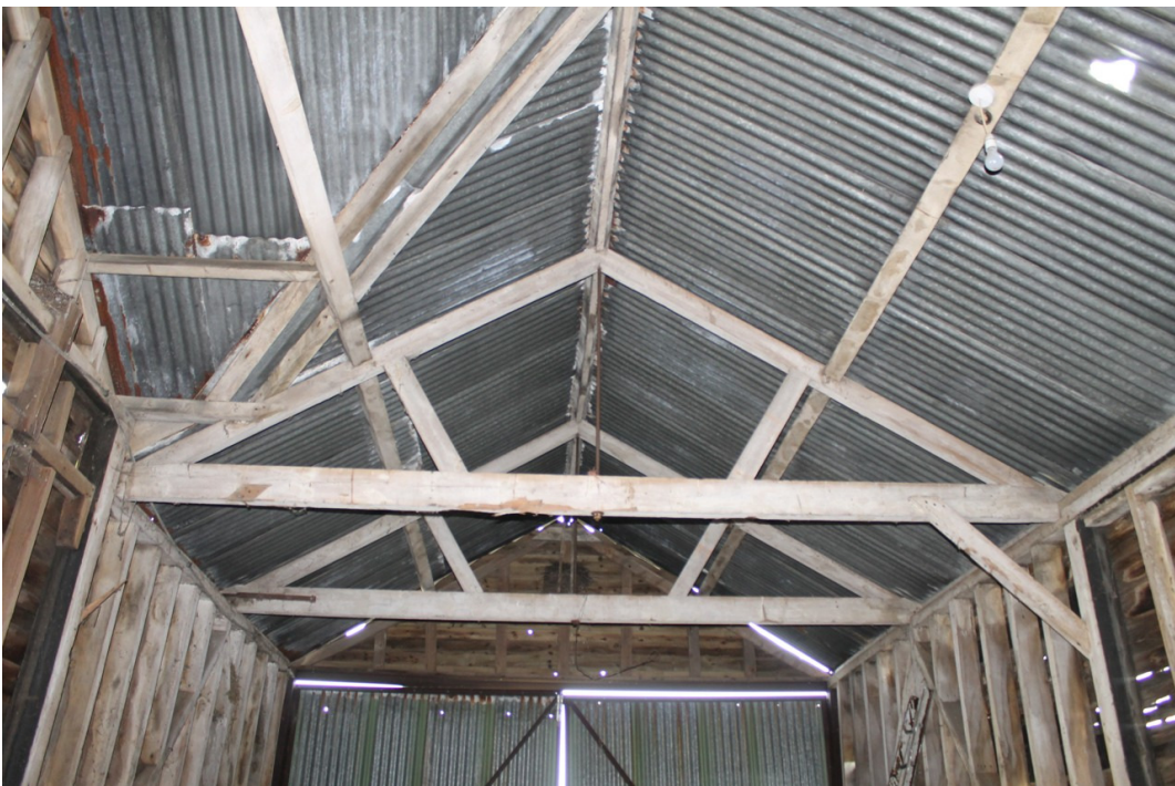
Photograph 10 Replacement roof truss (truss B) of machine-cut timbers in 18th-century barn, with nailed brace and steel king bolt – view north-east.
