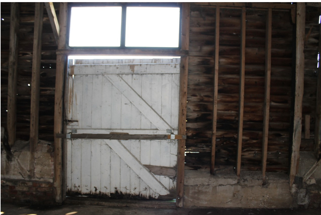
Photograph 16 North-west framing to bay 3 showing partially blocked cart door opening to midstrey and replacement door – view north-west.
