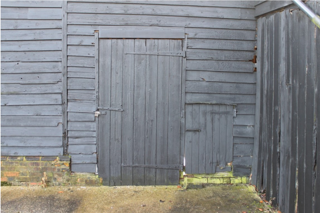
Photograph 3 North-west elevation, door to bay 7 (19th-century extension) with small modern door to the right - view south-east.
