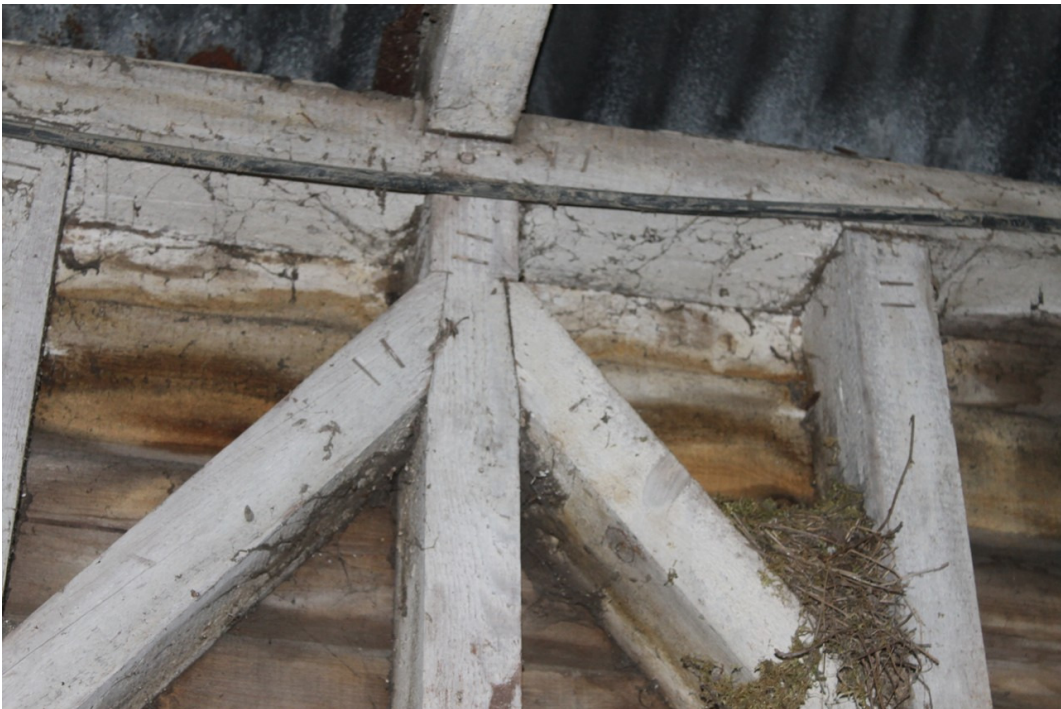
Photograph 14 North-west framing to bays 2 and 1 showing carpenters' marks 'll' on heads of studs and principal post to truss A - view north-west.
