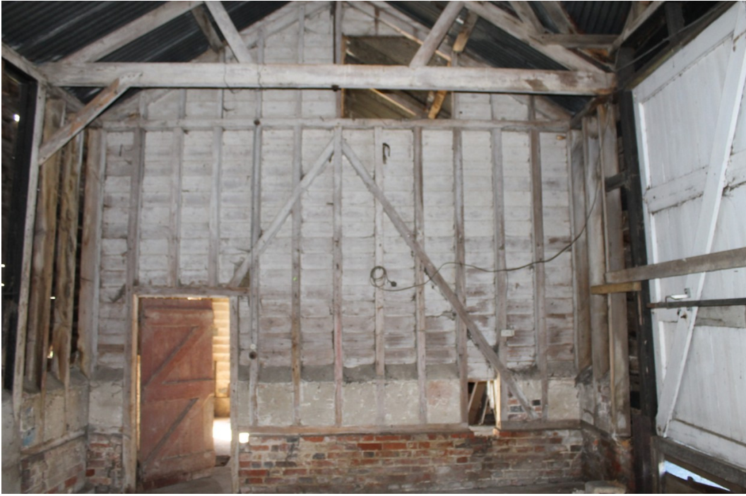
Photograph 23 Gable end framing separated from bay 6 by a narrow bay, with inserted doorway to the 19th-century extensions beyond – view south-west.
