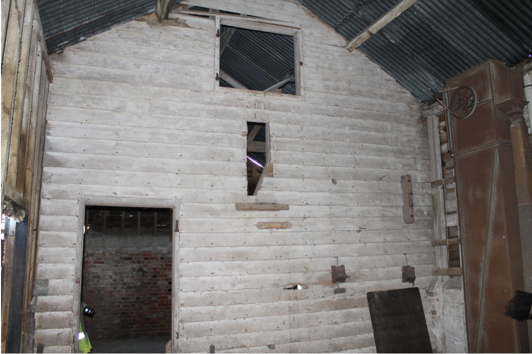
Photograph 25 Weatherboard covering the north-east frame of bays 9 and 10, an earlier structure incorporated into the barn, viewed from bay 8. The frames of bay 7 and 8 are built up against this early 19th-century structure - view south-west.
