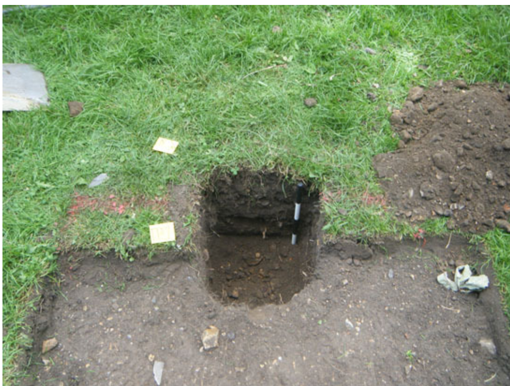
Photograph 1 Hole for the interpretation panel and area strip for paving, looking W
