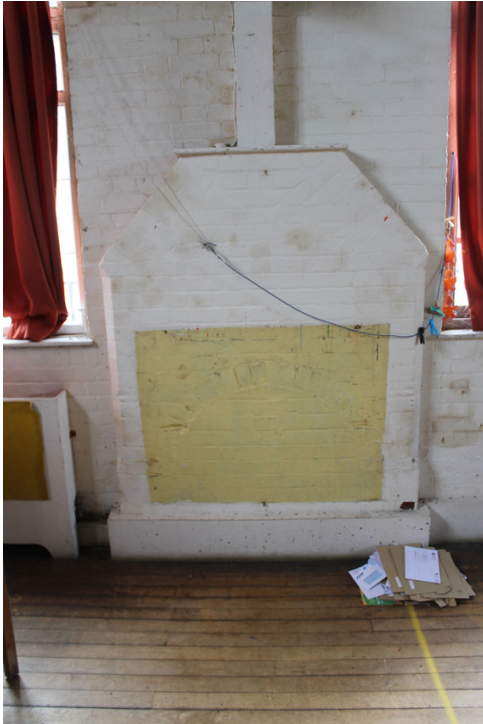
Photograph IX Blocked reinforced fireplace with principal post rising to truss. Shot taken facing north-east.
