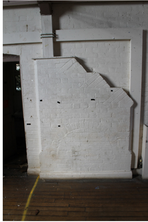
Photograph X Blocked fireplace with buttressing supporting principal post rising to truss. Shot taken facing south-west.
