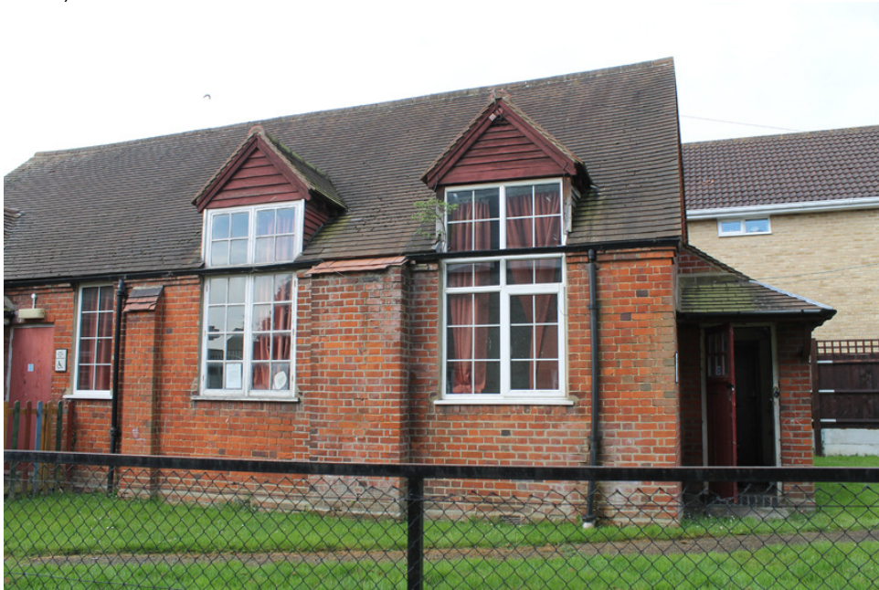
Photograph IV North-east elevation of building. Three replacement windows and inserted dormers visible. Central window opening has been raised – with replaced brickwork below.
