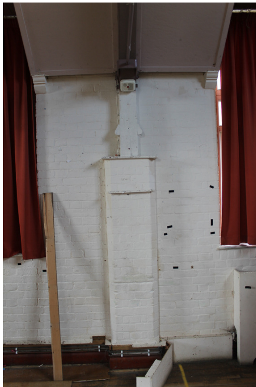
Photograph VIII Brick plinth supporting principal post and truss above. Shot taken facing south-west.
