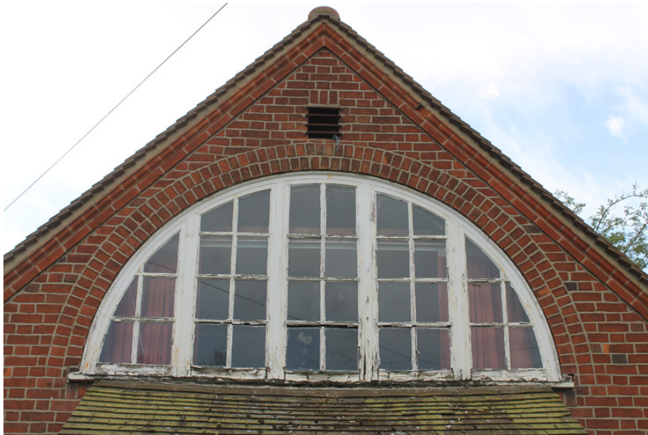
Photograph V Original north-western gable end window. Inserted ceiling panels visible. Shot taken facing south-east.
