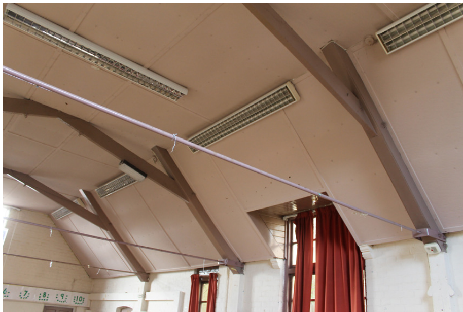
Photograph XI Shot showing roof trusses and supporting brackets for inserted ceiling panels. Shot taken facing south.
