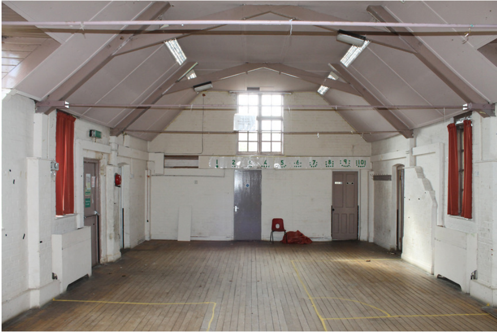
Photograph VII Interior of building. Composite truss and inserted ceiling panels visible. Shot taken facing south-east.
