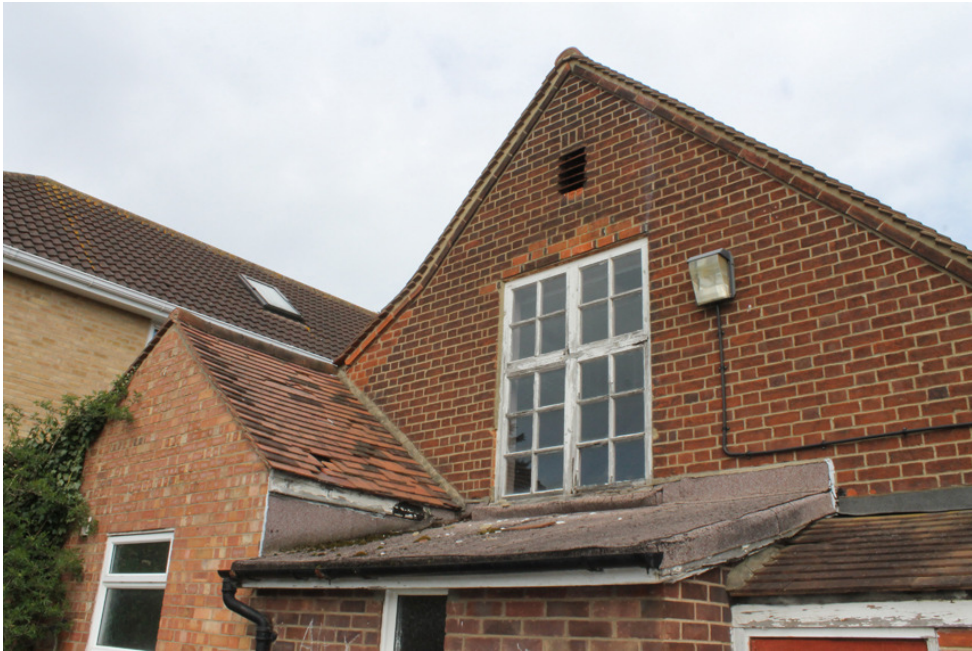
Photograph VI South-eastern gable end of building. Original window visible with evidence of possible replaced lintel. Extension of tile roof to cover second extension also visible. Shot taken facing west.
