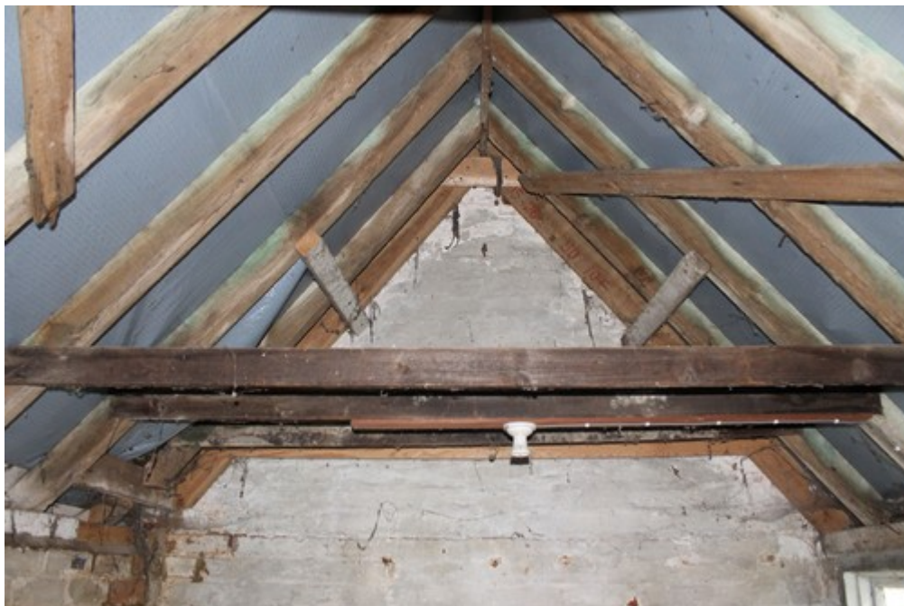
Plate 16 Rebuilt roof of outbuilding, showing machine cut timbers and underlay – view north.
