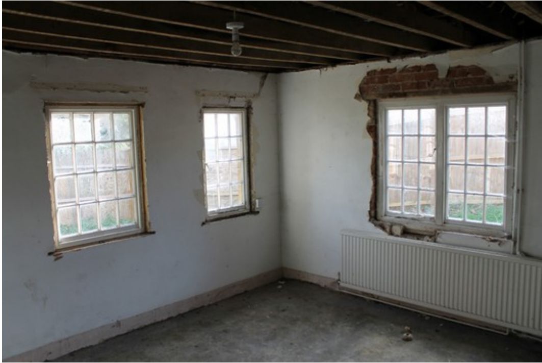
Plate 9 Interior shot of Room 1, with inserted window through original doorway to the left – view south-east.
