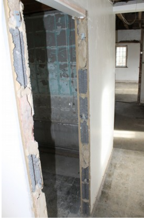
Plate 19 Interior shot of 20th-century extension, showing internal wall construction of breeze blocks and wooden panels – view north-east.
