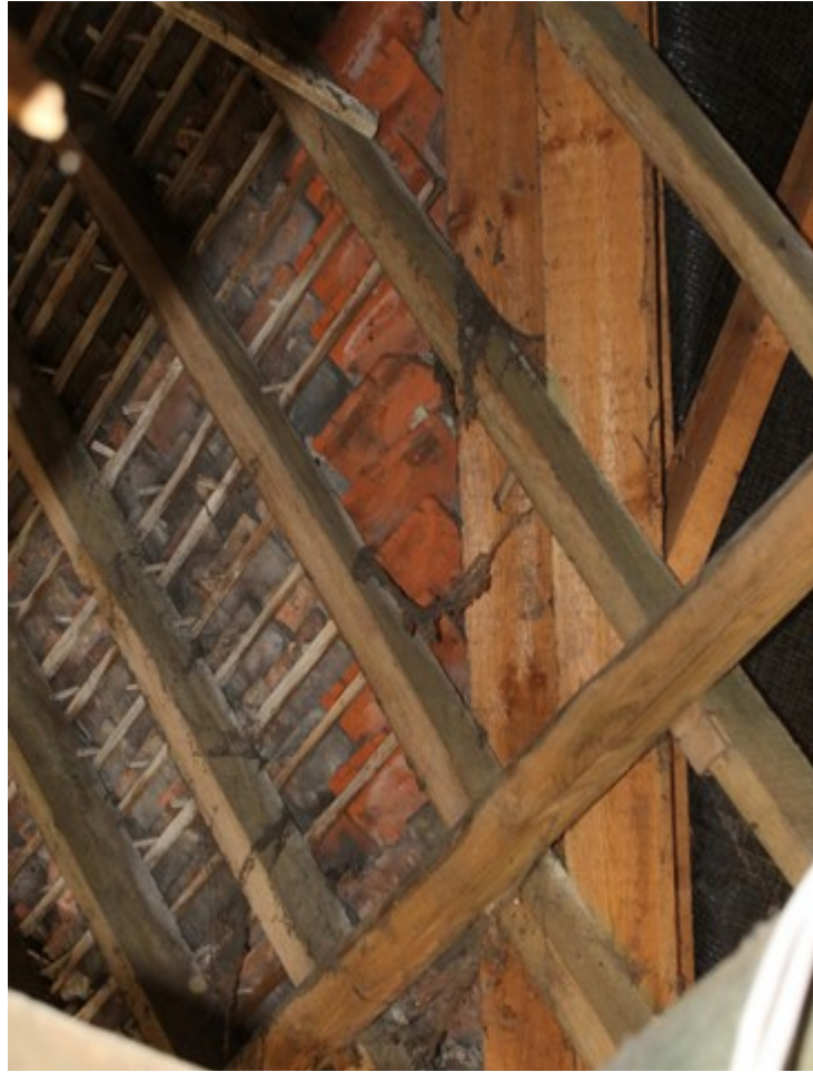
Plate 23 Detailed shot of 20th-century tiles. They are hung rather than pegged onto the battens – view south-west.
