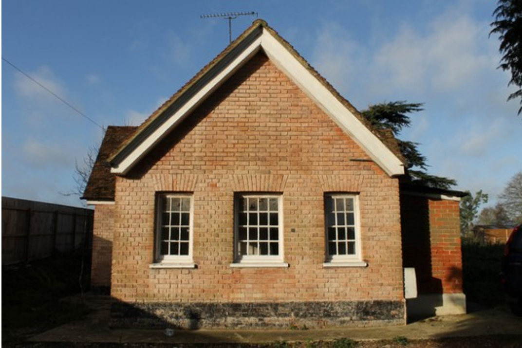
Plate 5 East elevation of the lodge, showing blocked up original entrance and replacement windows – view west.
