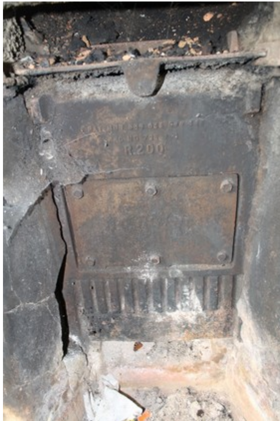
Plate 12 Detailed shot of back boiler, just visible is the brand name "RedFyre" - view west.
