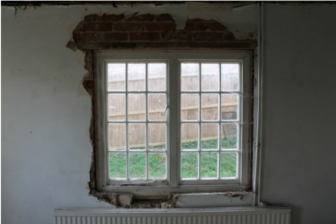
Plate 10 Detailed shot of replacement window on south wall of Room 1. Wooden lintel clearly visible – view south.
