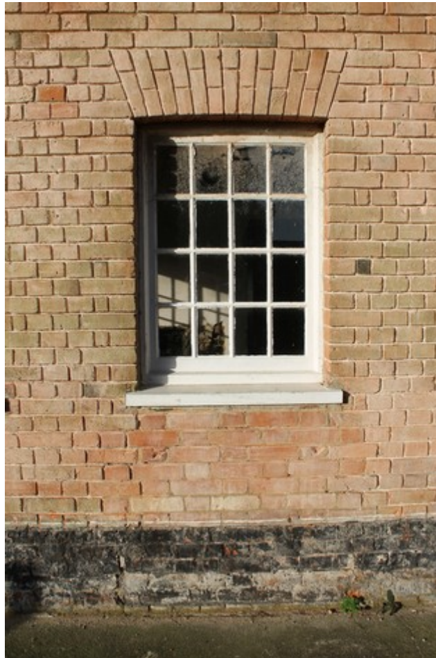
Plate 6 Detailed shot of blocked up doorway and inserted window in east elevation – view west.
