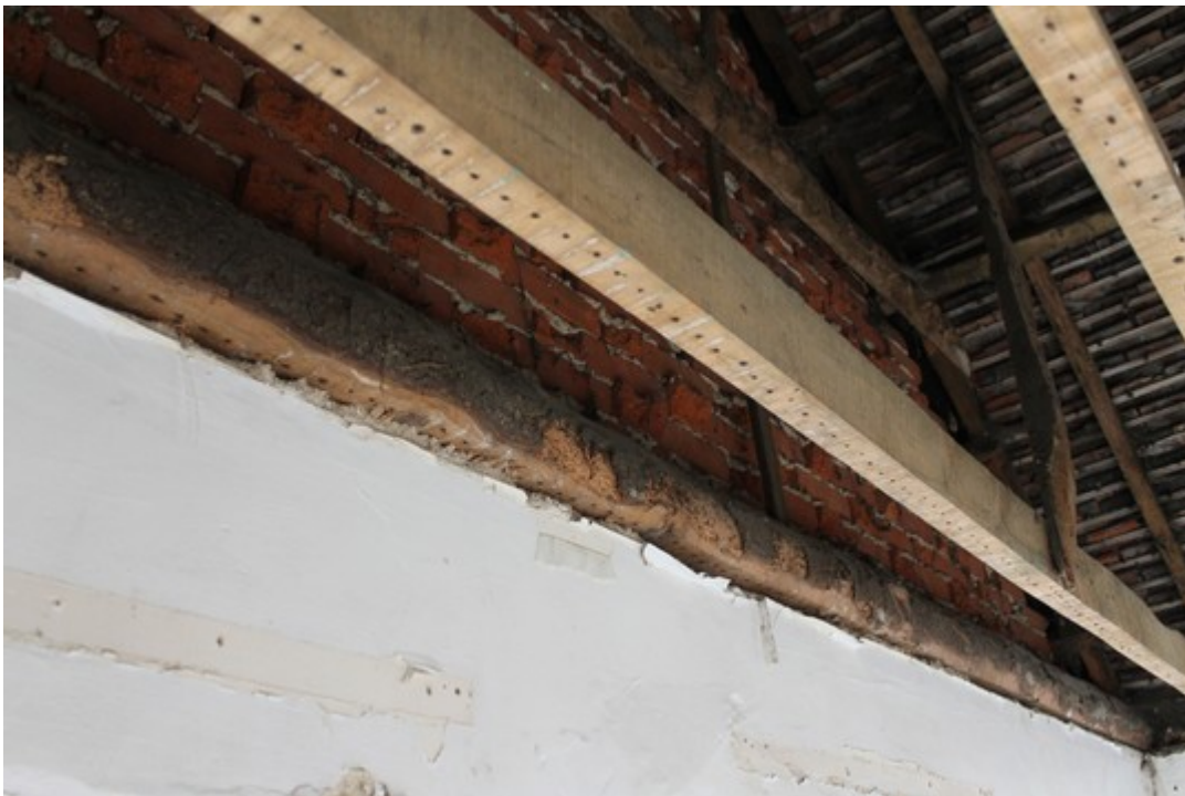
Plate 20 East gable end of lodge, showing partly worked tree trunk in use as a wall plate – view south-east.
