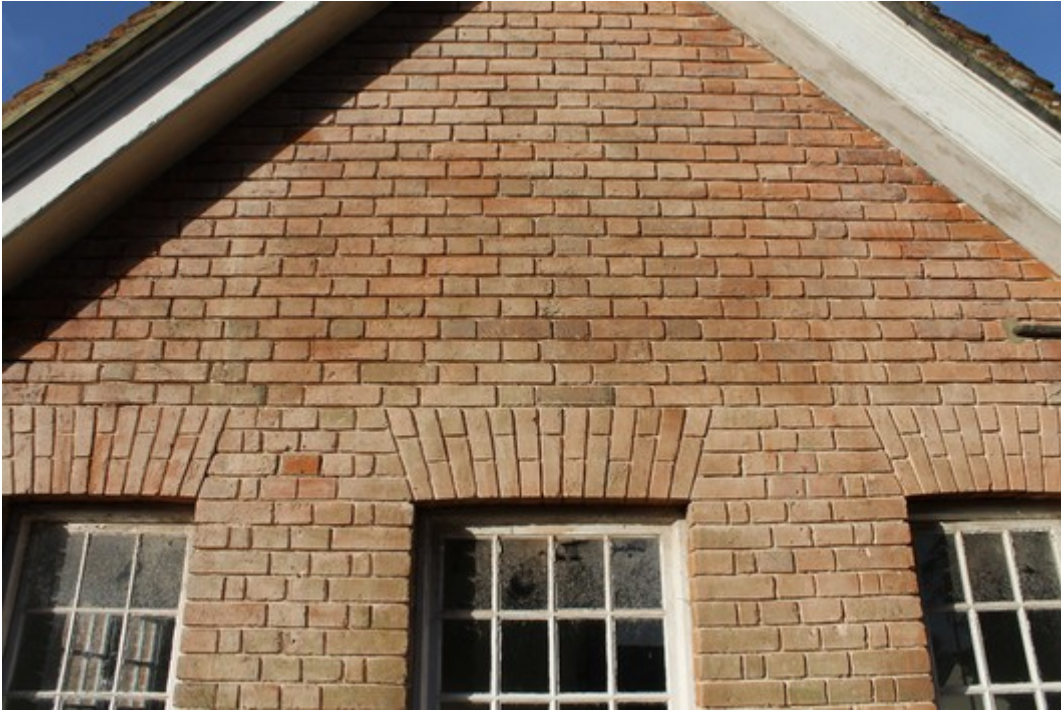
Plate 7 Faint scarring of porch visible on east elevation above blocked up doorway – view west.
