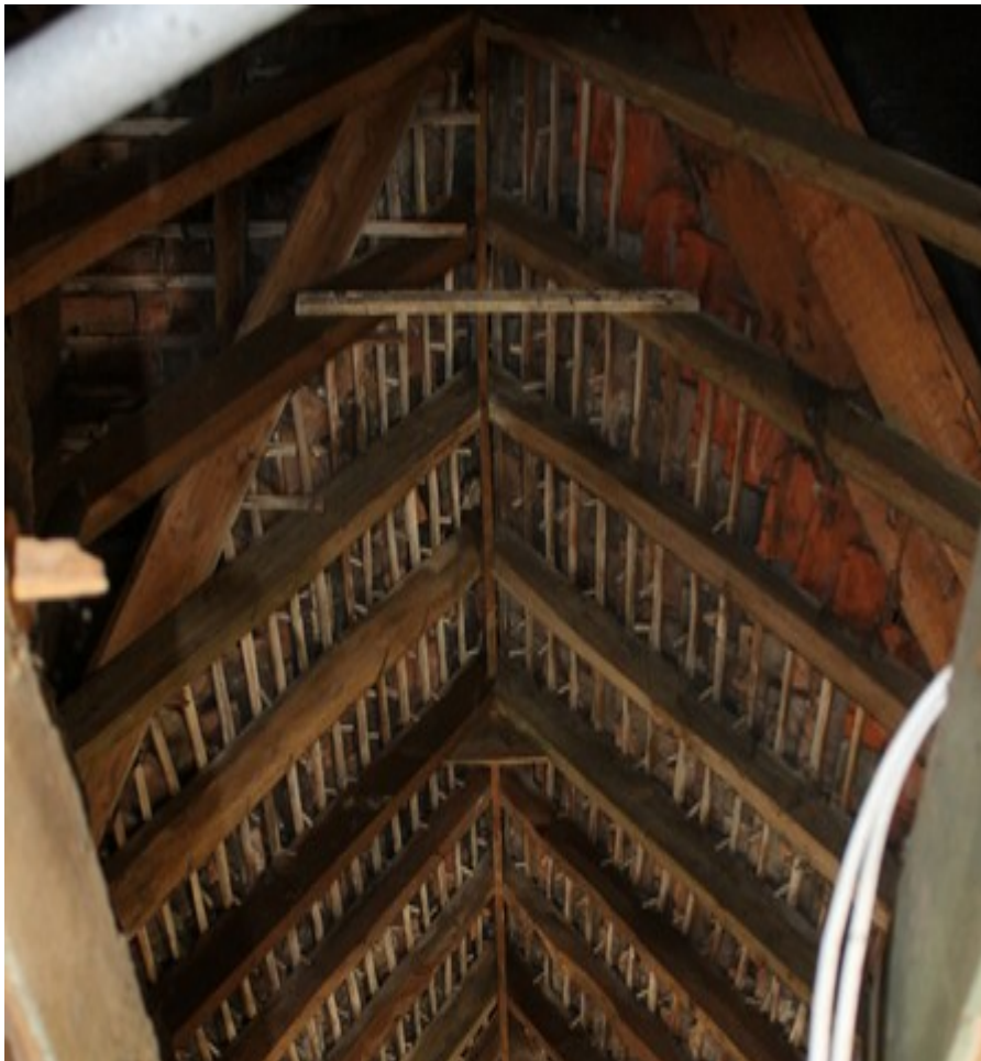
Plate 22 Roof structure leading to south gable end above Room 2. Visible to the right are 20th-century tiles joining from the extension – view south.
