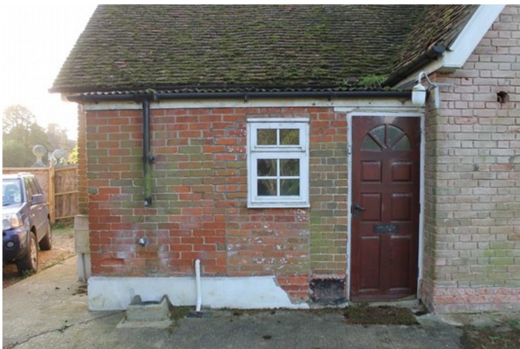
Plate 2 North elevation of the lean to, showing 20th century additions and inserted door and window – view south.
