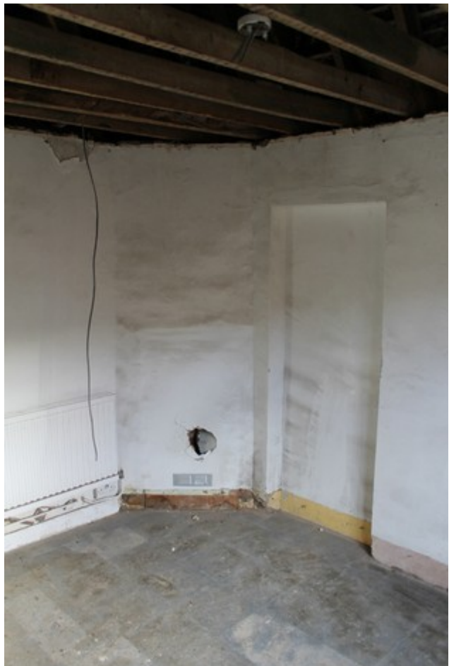
Plate 18 Interior shot of Room 2, showing blocked up doorway into Room 1 and fireplace – view north-east.
