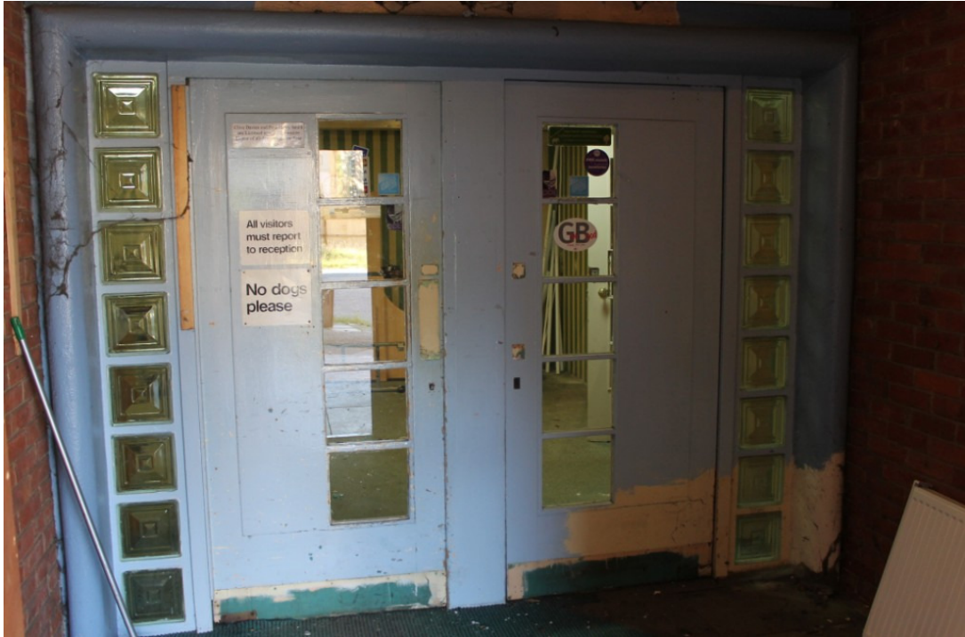
Photograph 12 The modern entrance to the Arena (GF2), one of the original entrances to the NAAFI with probable replacement doors – view north-west
