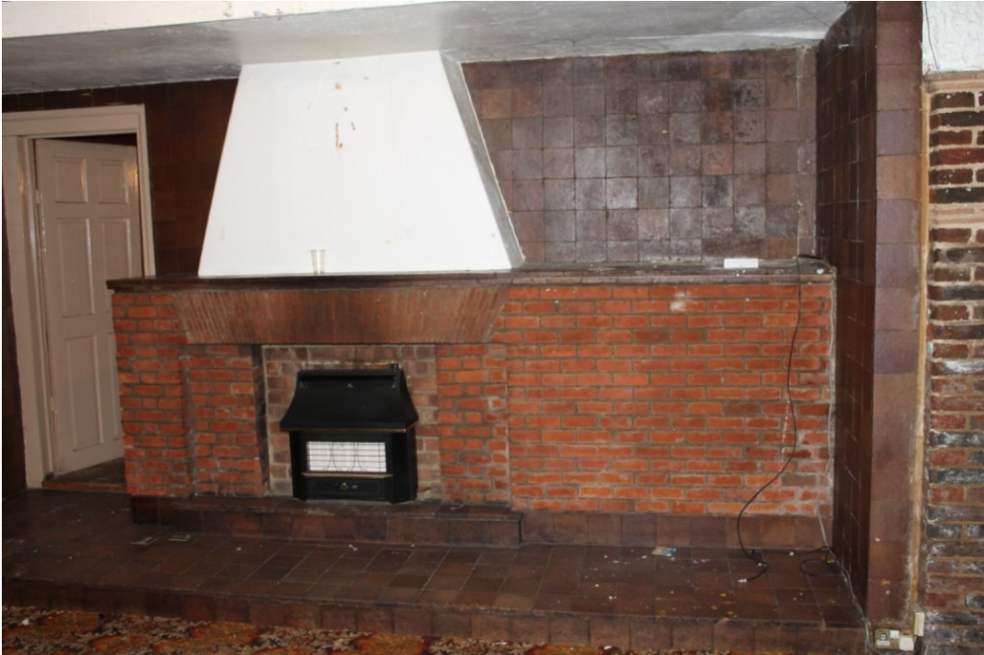
Photograph 19 Original NAAFI Lounge smoke hood located in GF3 - view south-east
