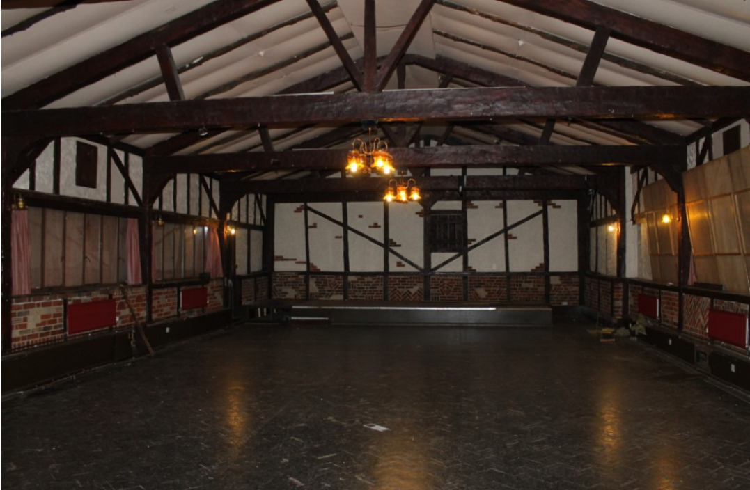
Photograph 27 The interior of FF1, with original parquet flooring and later faux rustic decoration - view south-east
