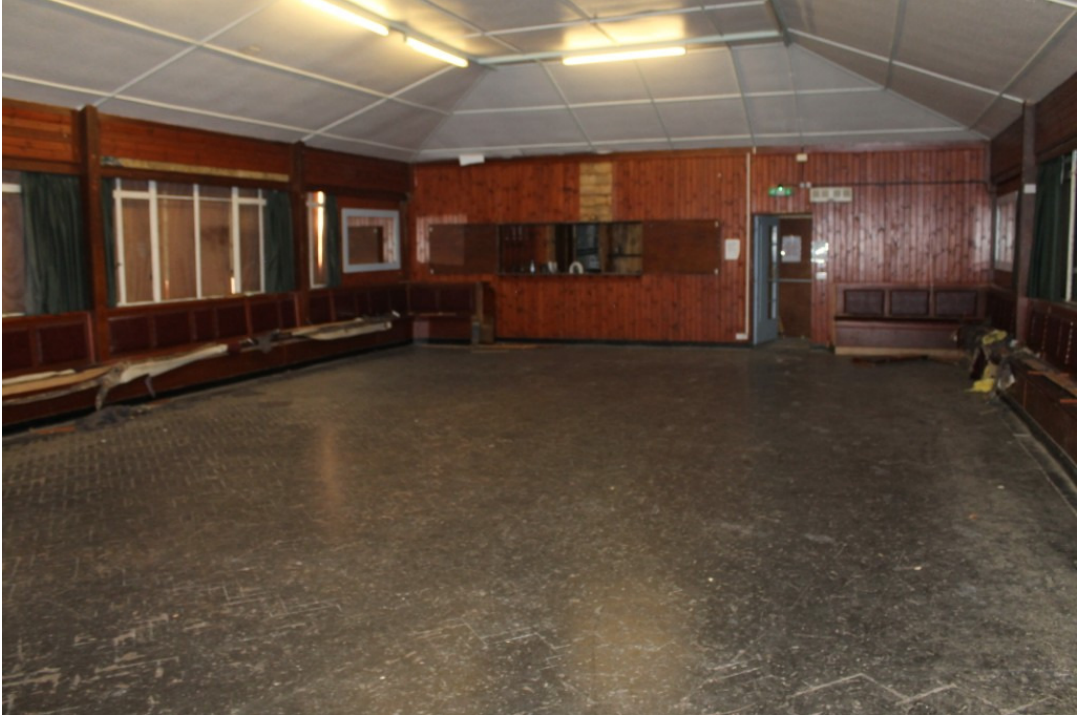
Photograph 26 The interior of GF7, with original parquet flooring, vertical tongue and groove cladding and bar in the far wall; the benches around the walls are probably later additions - view south-west
