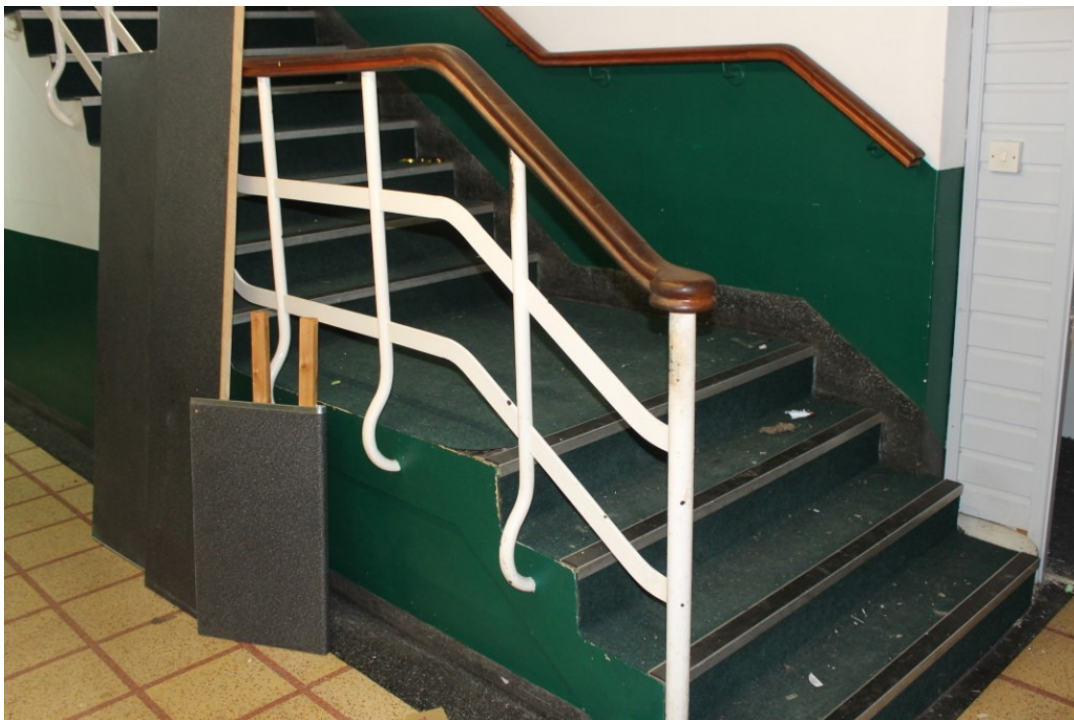
Photograph 17 The staircase located in GF2 providing access to the first floor – view north
