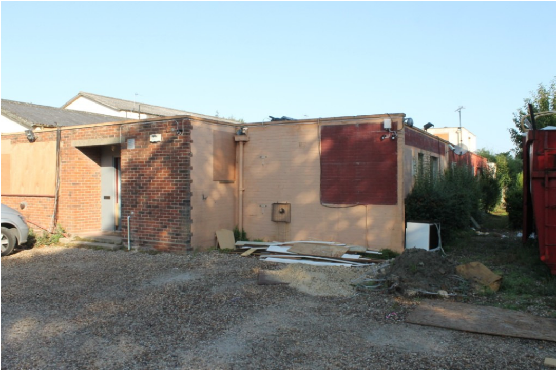
Photograph 5 South-east elevation of GF5, most recently used as a base for a taxi firm – view north-west
