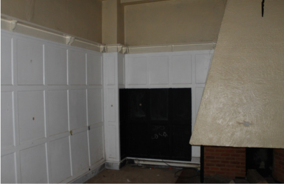
Photograph 25 A probable dining room located in GF6, with original parquet flooring, wood panelling and hearth with large smoke hood, identical to the one in GF3 - view north-west
