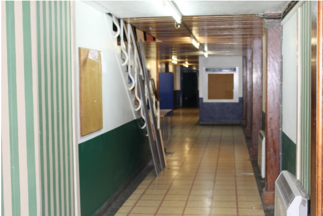
Photograph 16 The corridor extending the length of GF2 with the original flooring and the stairs to the first floor – view south-east
