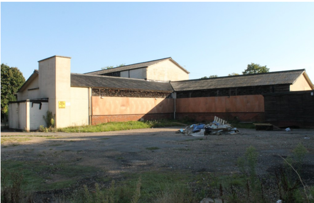
Photograph 6 Areas GF7 and GF4, most recently used for the Arena Gym – view north
