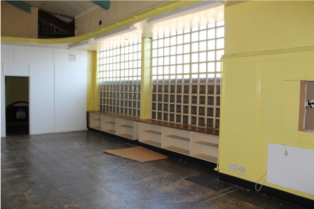
Photograph 30 Eastern half of FF2 showing the original parquet flooring, wood panelling and glass block wall. The white painted stud wall to the right conceals the original curved wall and brick hearth at the end of the room. The serving hatch connecting FF2 and FF3 is just visible on the right of the photograph – view north
