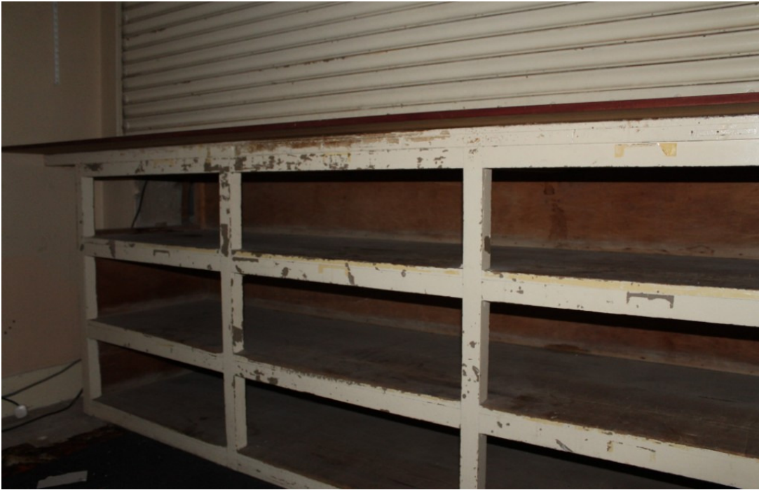
Photograph 10 An original NAAFI serving hatch and counter in the south-east corner of GF1 – view south-east
