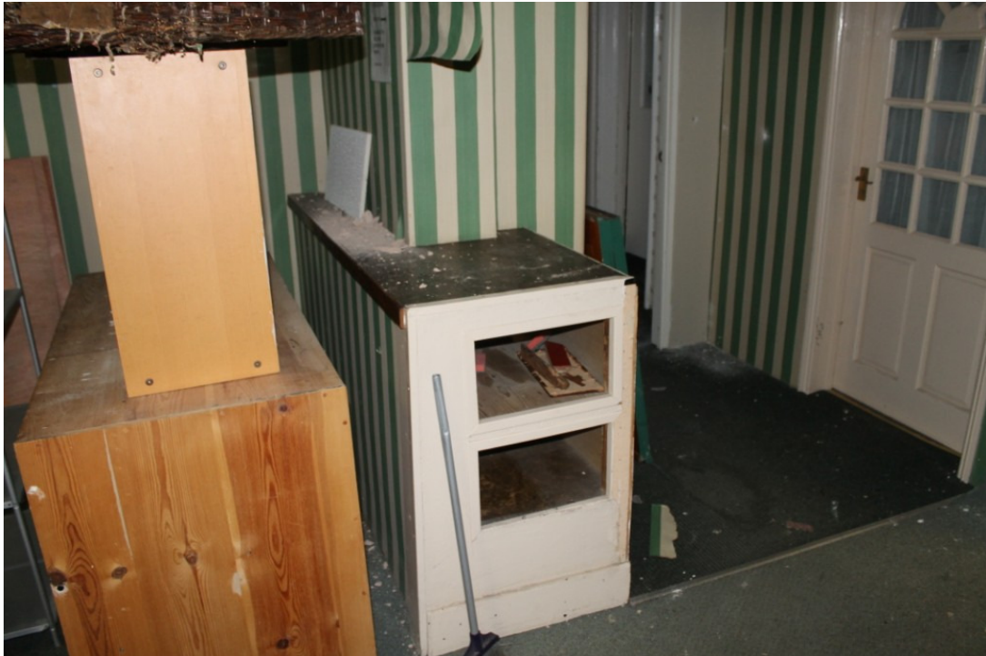
Photograph 14 Part of the original NAAFI servery in GF2, cut to provide access to the rooms behind – view south
