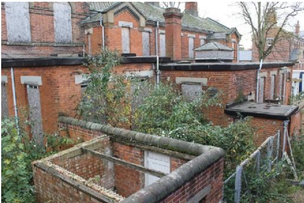
Plate 12 The north-west elevation with the 1922-62 single-storey extensions in the foreground - view south
