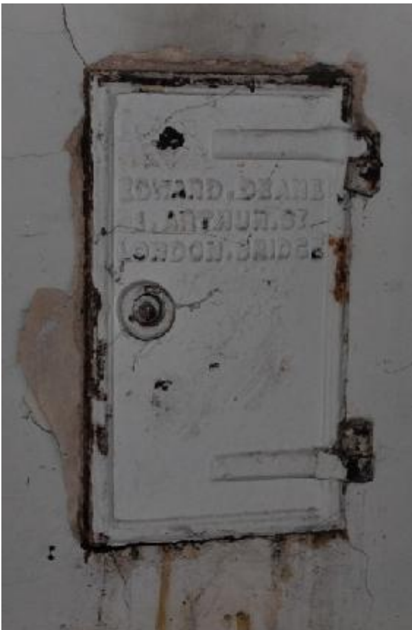
Plate 36 Detail of the original soot door in the first floor wall of stairwell iii
