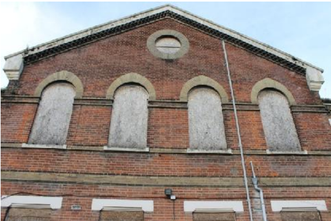
Plate 2 Central projecting gabled section of south-east elevation, showing the pointed arches of the first floor windows and the oculus above – view north-west
