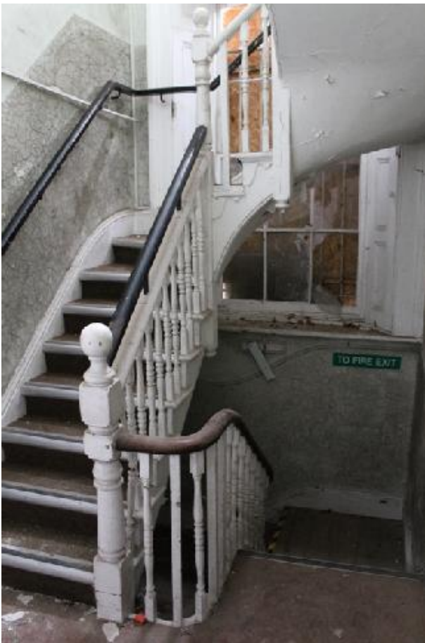
Plate 26 Servants' stairwell v, with the original access to the basement and the inserted staircase to the first floor - view west
