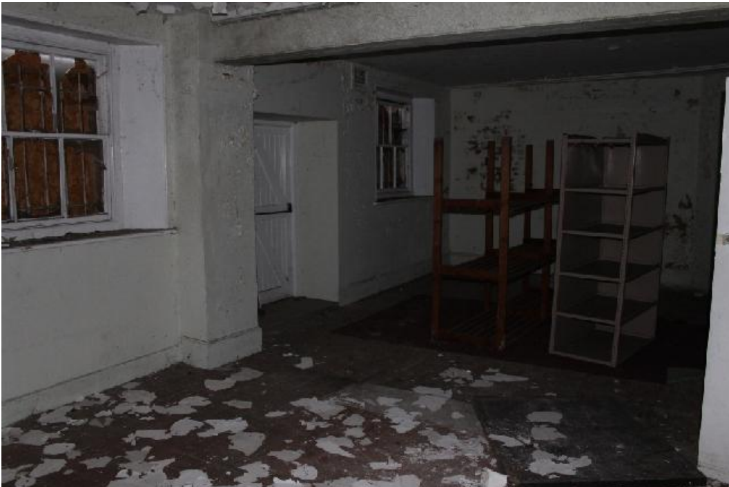
Plate 44 Rooms 39 and 38, the former kitchen and mess manager's room, with the dividing wall removed and a doorway inserted through one of the windows of the mess manager's room – view south
