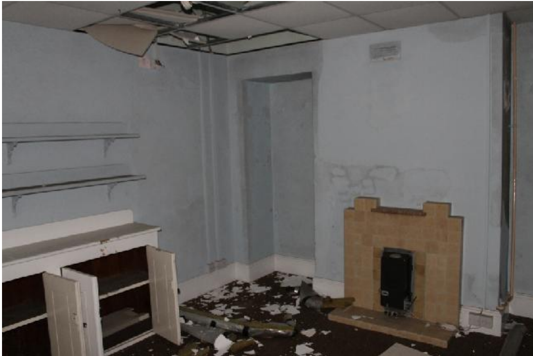
Plate 31 Room 18, formerly quarters for the servants of Officers Nos.1, 6 and 7, showing the bricked-in original doorway to the left of the chimney breast and the double-width dresser on the dividing wall – view south
