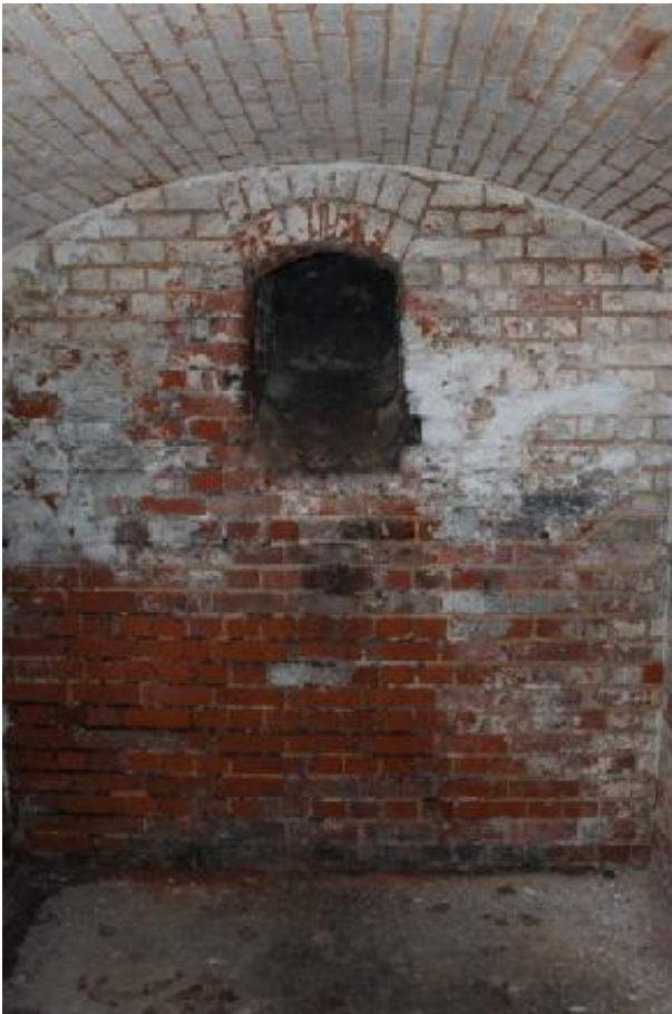
Plate 40 Room 34, the brick vaulted coal store with the original coal chute – view north-east
