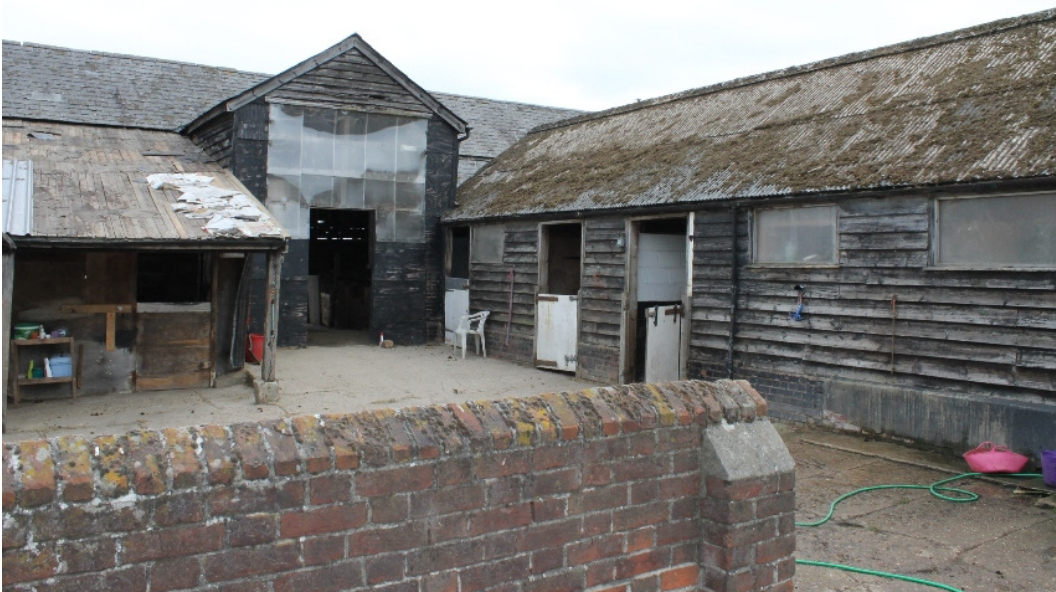
Plate 2 North midstrey with boarded over opening and modern stable blocks to left and right – view south-east
