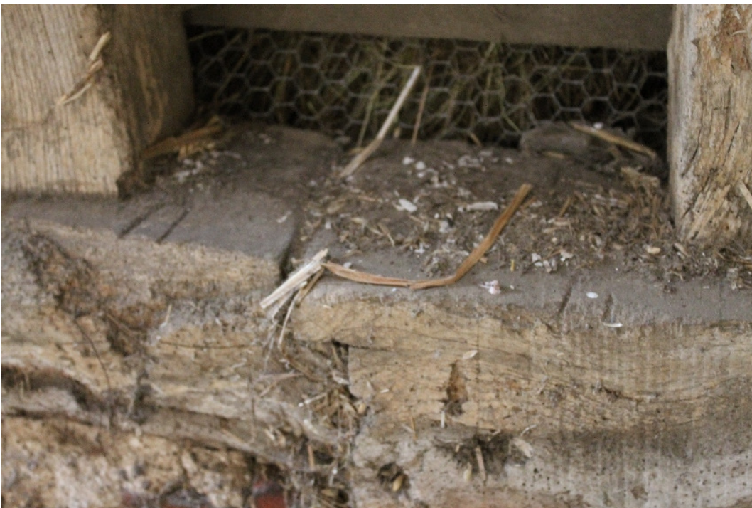
Plate 8 Carpenter's marks (II) on either side of edge-halved scarf joint in the sill beam of the south wall - view south-east.
