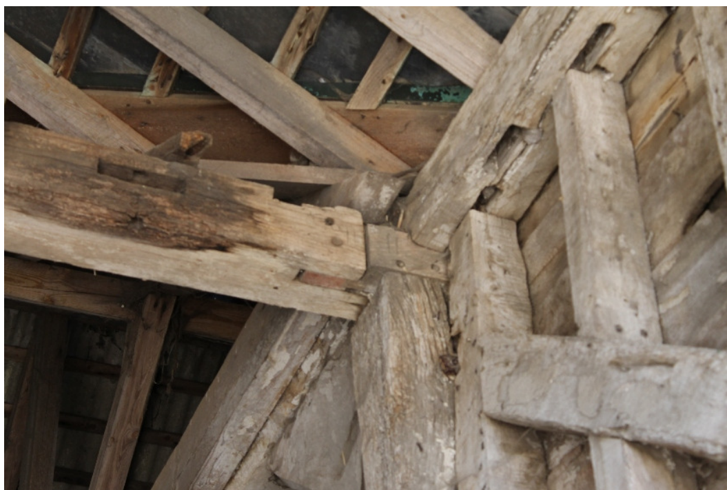
Plate 15 Chiselled carpenter's marks 'll' on post of truss J and bridging beam of south midstrey - view east
