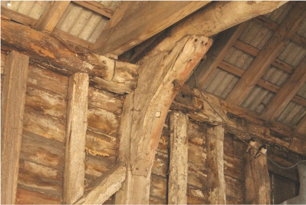
Plate 7 Bolted knee brace to truss J and face-halved scarf joint on wall plate of bay 10 – view north-east
