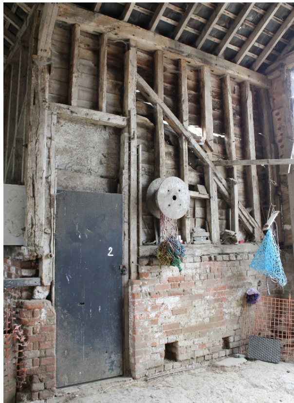
Plate 12 North midstrey, original doorway to lean-to and recess in brickwork, possibly for a boot scraper - view south
