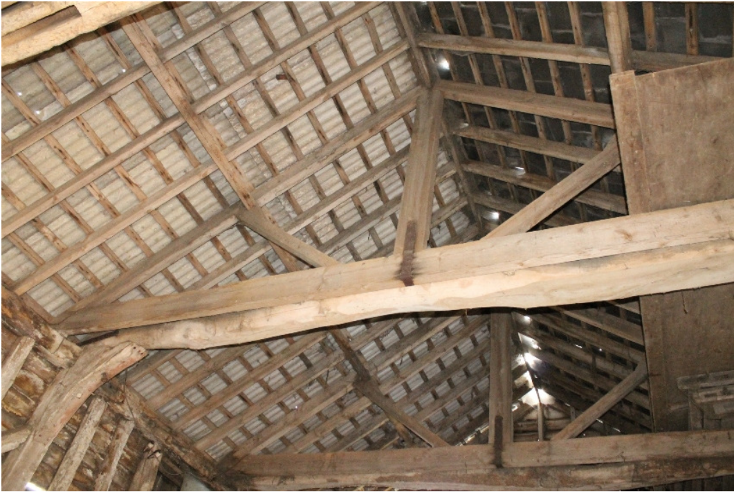
Plate 9 Truss J, original cambered tie beam and bolted knee brace with machine-cut secondary tie beam, king post, inclined struts and principal rafters – view south-east
