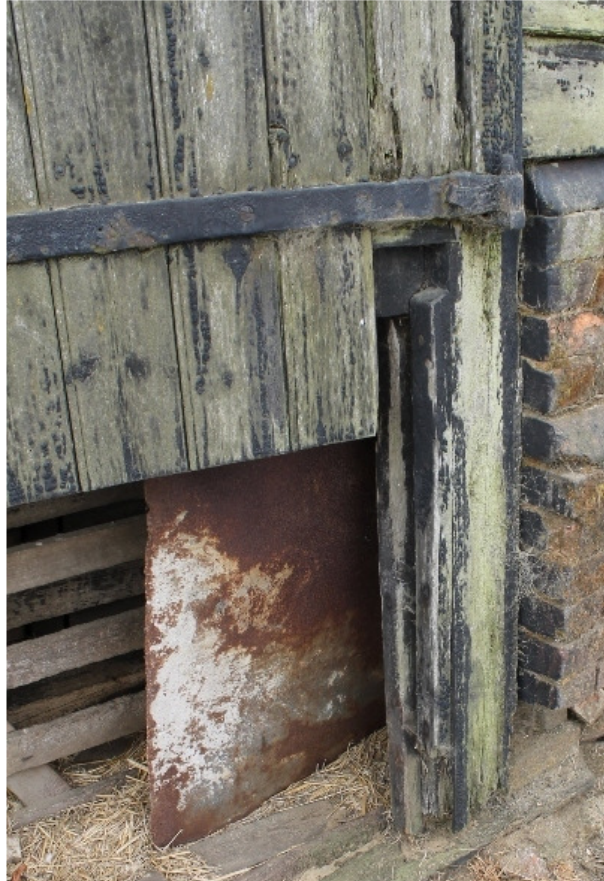
Plate 5 Detail of strap hinge on barn door to bay 9 and threshold leap – view north-west
