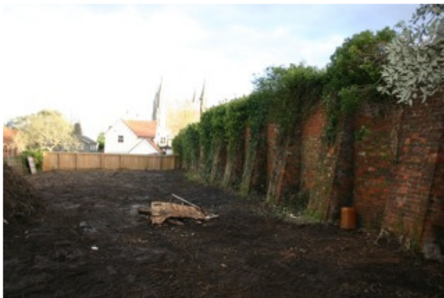
Plate 1: part of the rebuilt stretch of St John's abbey precinct wall, which forms the south boundary of the site (north is to the left).
