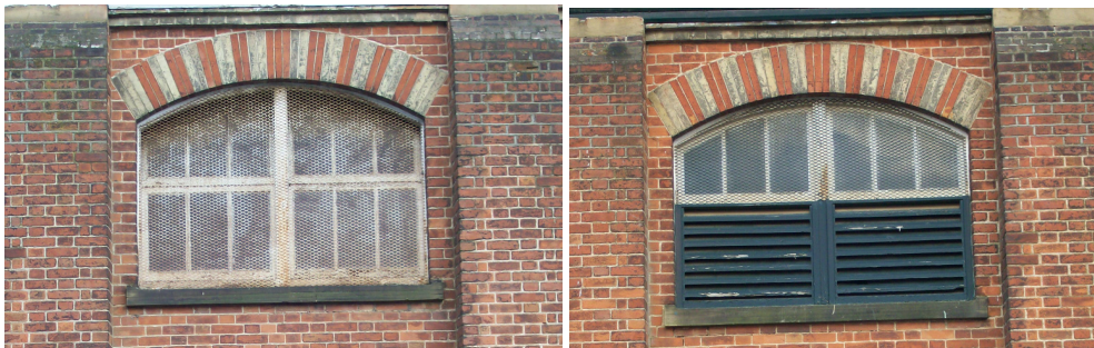
Plates 2 and 3. South-east wall – differences between windows.
